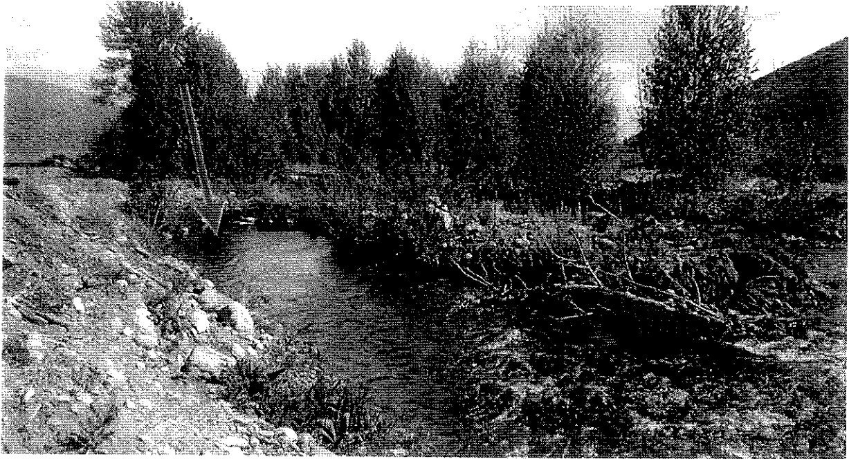
Figure 3. Upstream of Ashcroft diversion looking at inlet to turbulent fountain trash screen.
