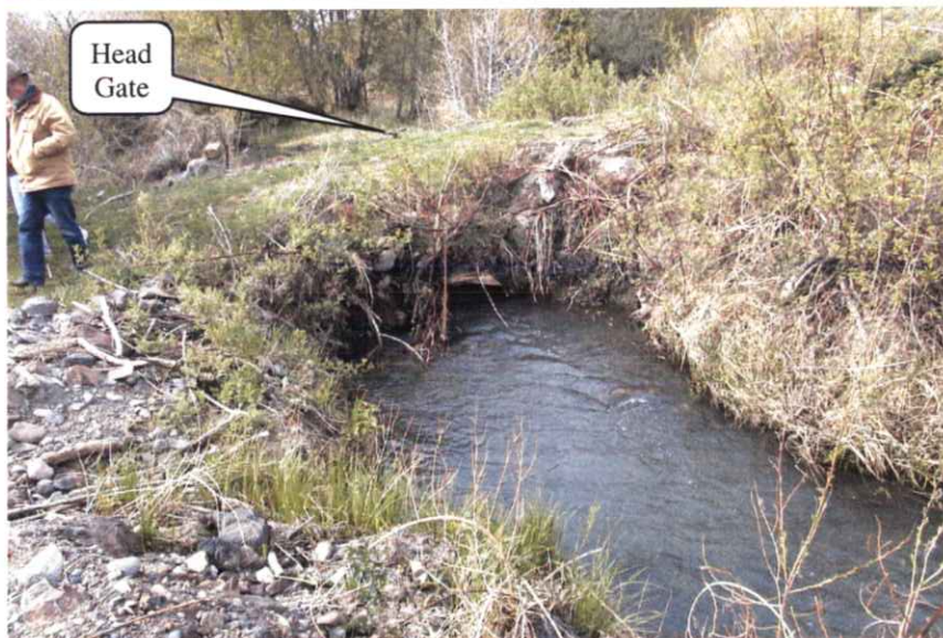
LEFT: View directly below the West Ditch diversion looking back up the West Ditch toward the diversion. Note the large flow entering the West Ditch from Rock Creek despite the diversion gate being in the closed position.
