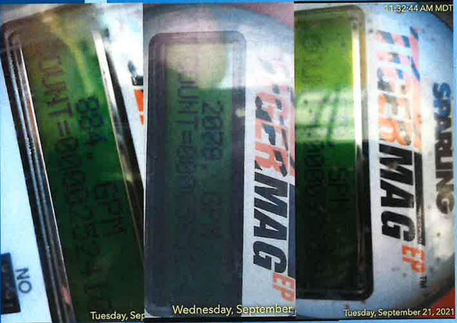
Sparling meters registering gallons while not pumping
