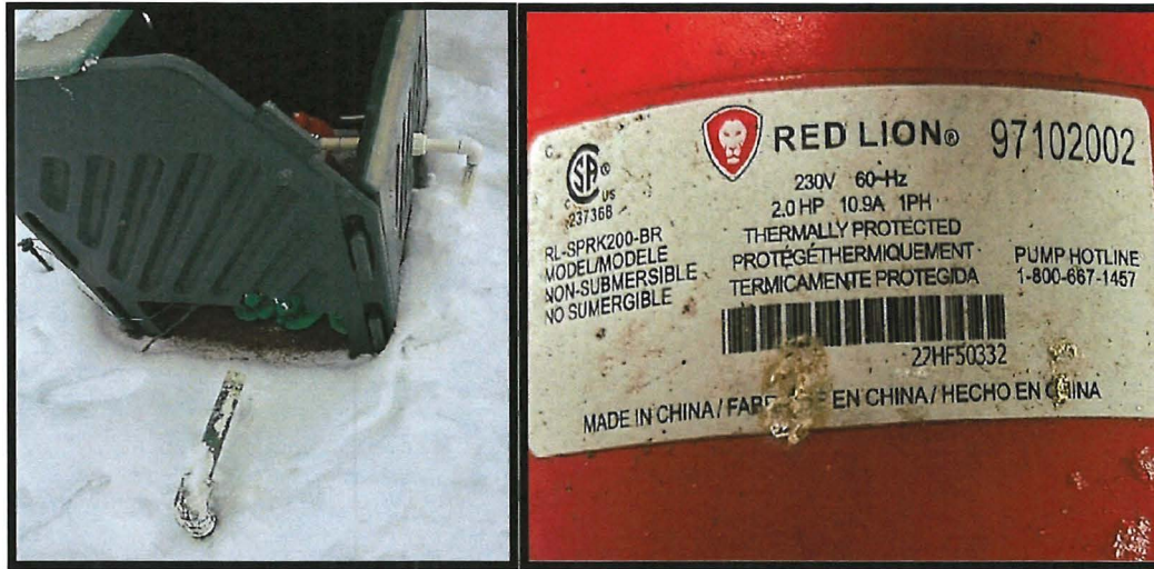
Photo 8a-(left) Green Plastic pump house with the intake disconnected for the winter and two 3/4" PVC discharge pipes deliver water to the 2 control valve boxes. Photo 8b-(right) Tag on the 2Hp pump motor used for irrigation within the POU.
