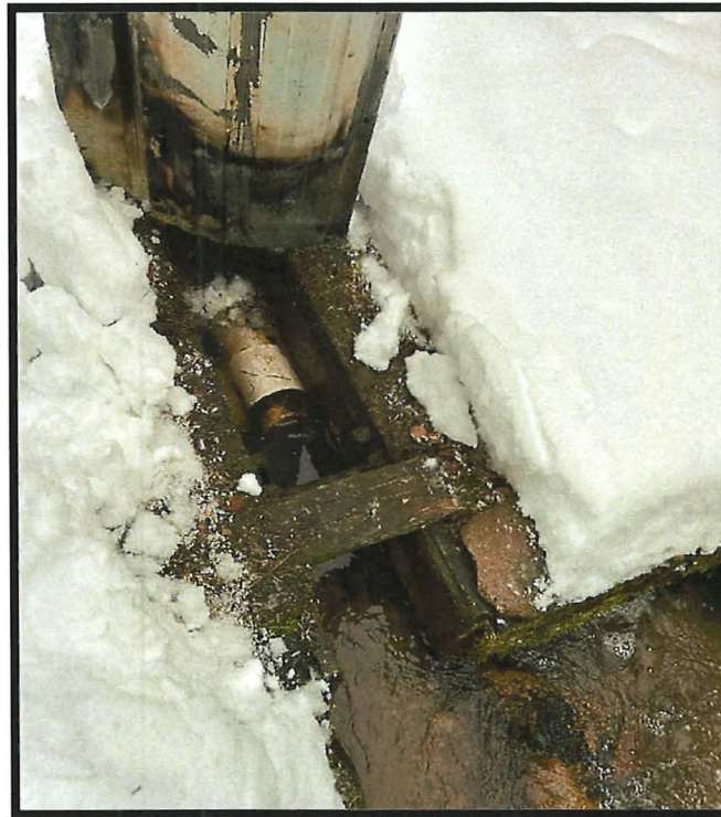
Photo 2- At the back of the wooden enclosure a 6" PVC pipe with a cap that covers \frac{1}{2} of the end of the pipe which can be rotated to allow for control of the volume entering the pipe and to keep sand from being entrained.
