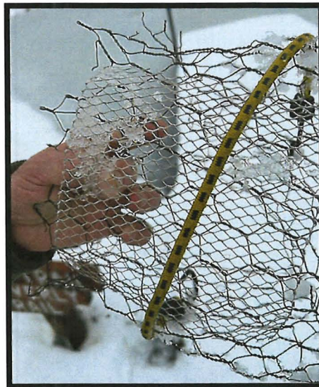
Photo 6- A ¼" screen like the one pictured here is normally wrapped around the outlet . They are removed and to be cleaned periodically.
