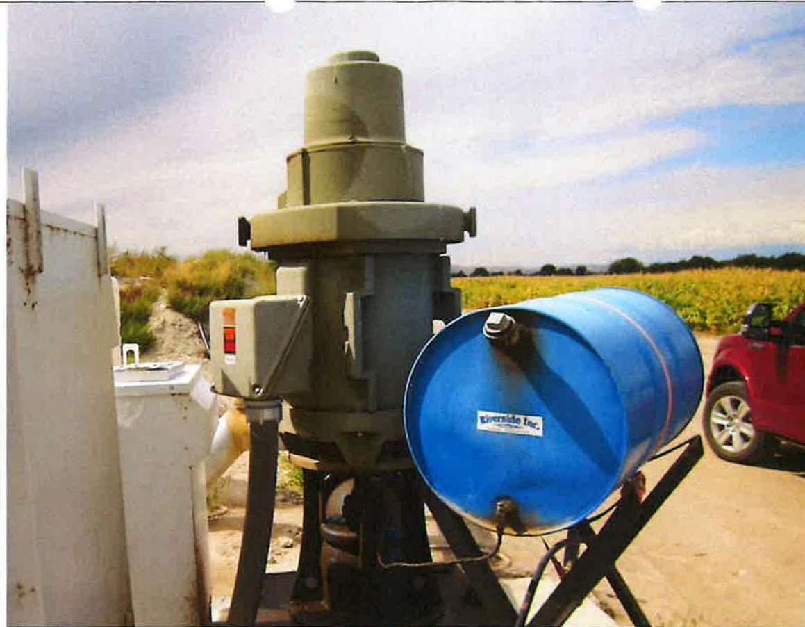
Figure 3. 200 hp motor and vertical turbine pump sitting atop well.
