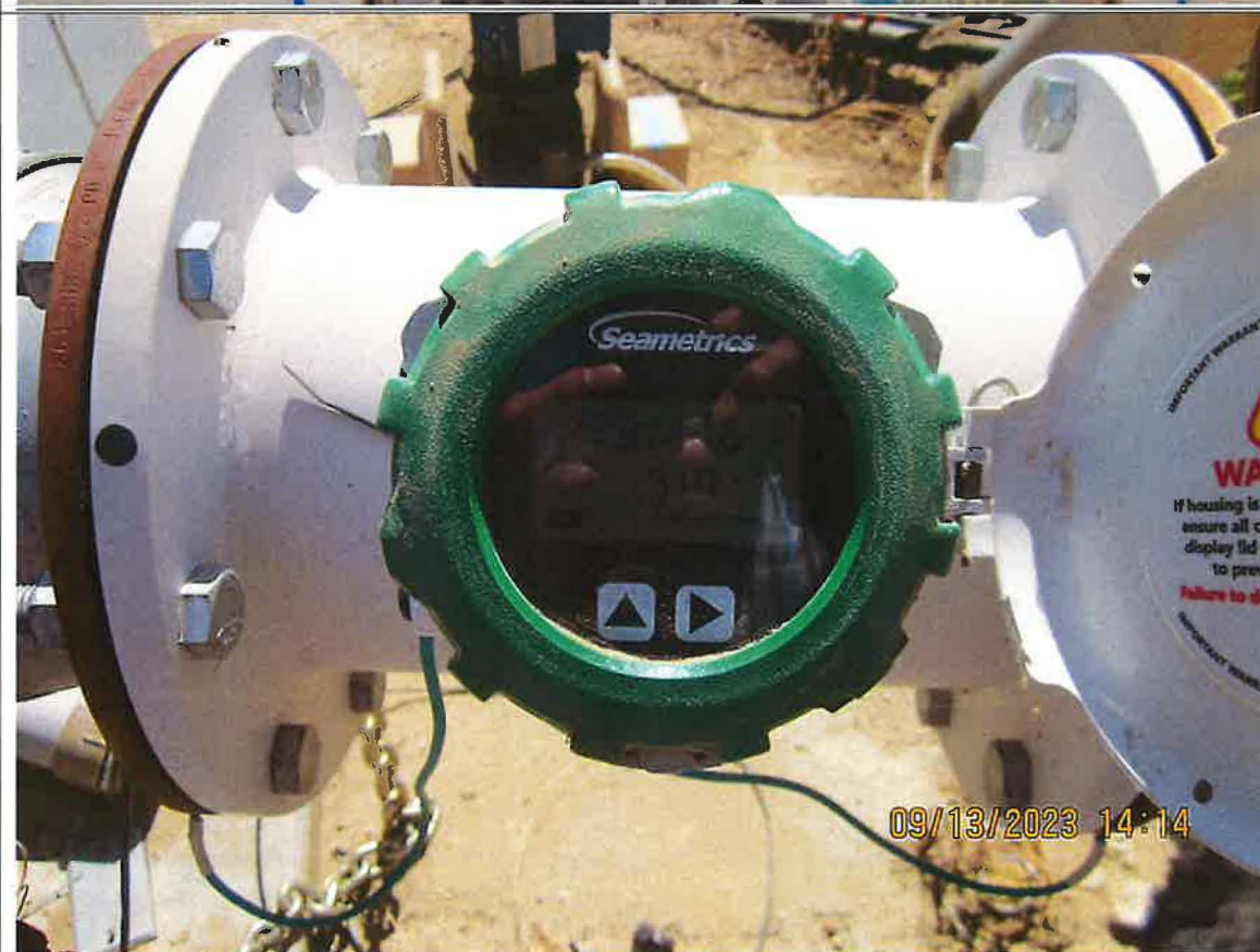
Figure 6. Seametrics flow meter reading 819 gpm.
