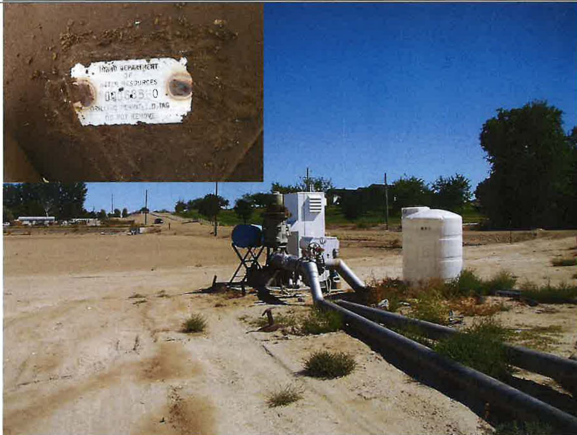
Figure 2. Pump, controller, and pipe manifold coming from well. Well ID tag # D0068860.
