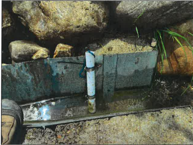
Photo 3. Looking across at the white plastic section of pipe that contains the water level monitoring transducer and the water flow gauge in the measurement flume in Ditch #1 on July 31, 2026. The water level is reading about 0.10 cfs on the plate with leakage that is coming in under the canal headgate.
