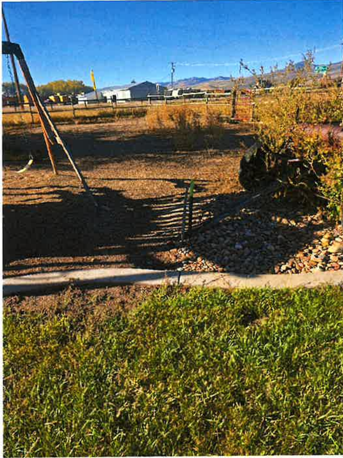
Figure 11: Riser located in in the center of the back yard at the Sparks residence where the system branches.
