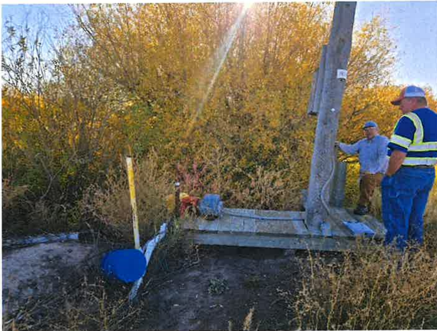
Figure 1: Irrigation pump assembly mounted to a wooden platform.
