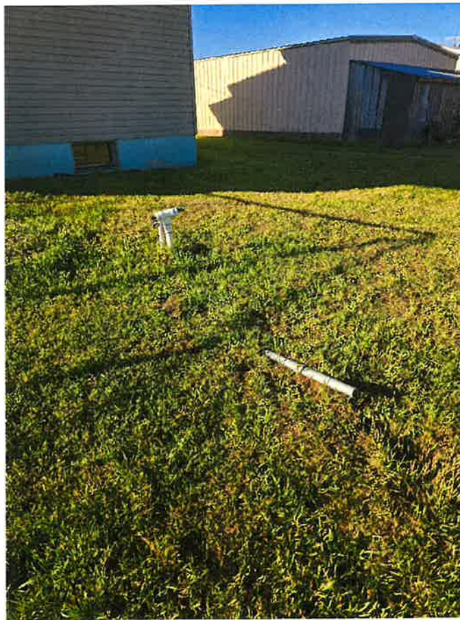
Figure 6: Riser located behind Kovack residence.
