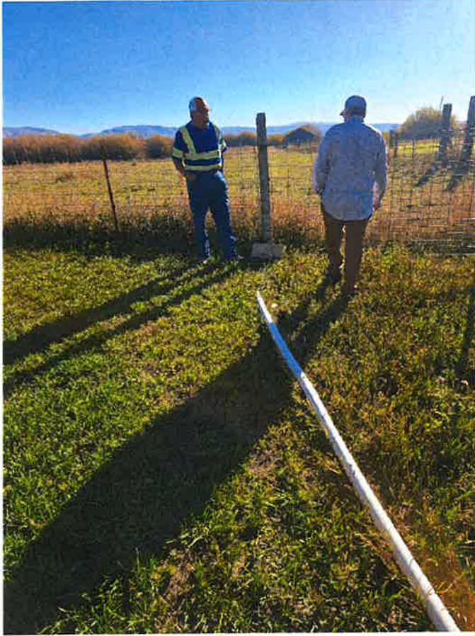
Figure 15: Conveyance line that breaches the surface on the Bergs Residence.
