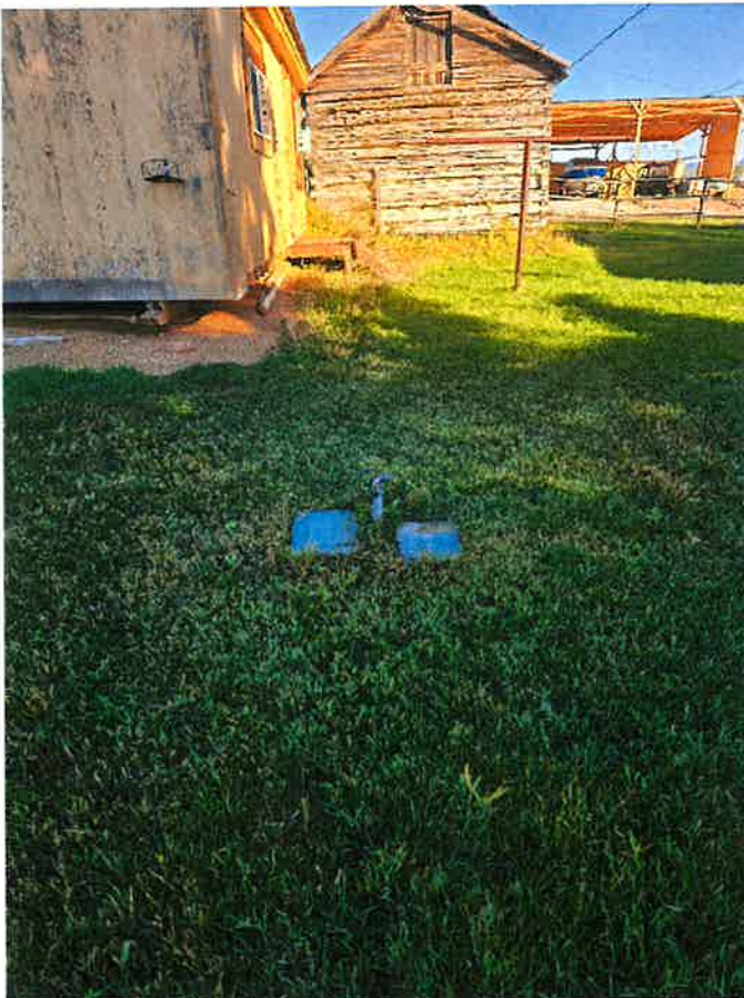
Figure 12: Riser located behind the Sparks residence with the control valve box and blow out box.
