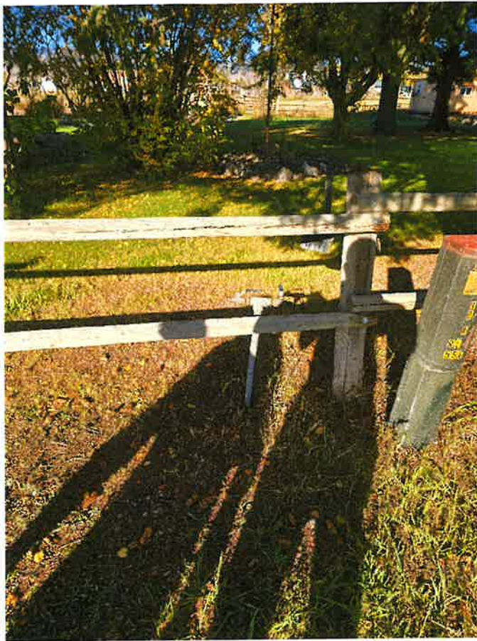
Figure 9: Riser located in front of the Sparks residence. Initial riser that the system connects into from under the street.
