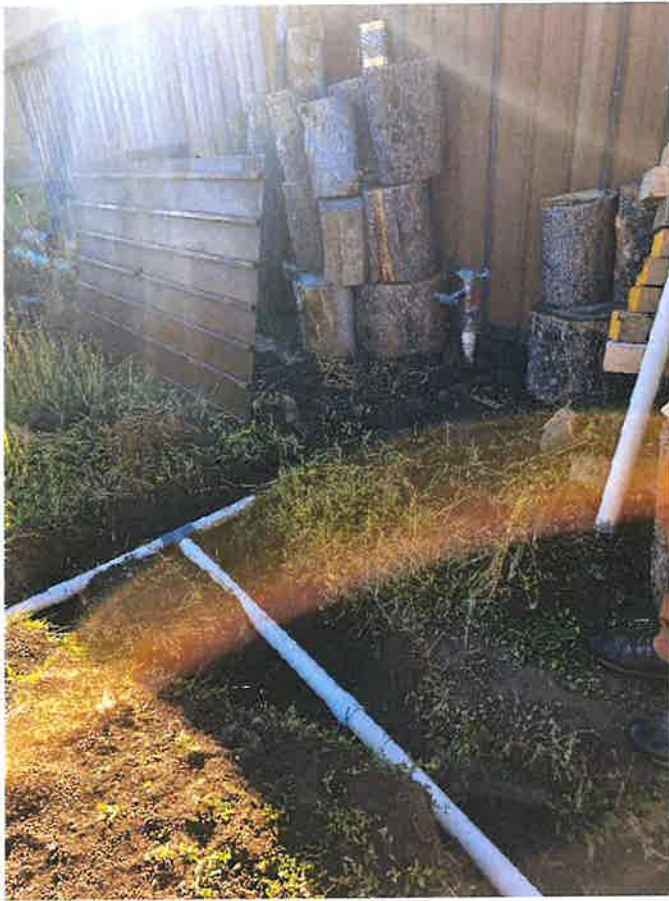
Figure 7: Riser located behind workshop at the Mattson residence showing the initial "T" branch towards the rest of the system..
