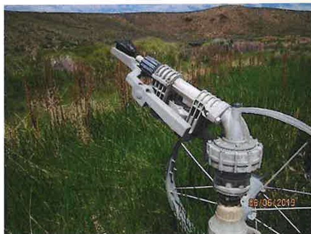
Sprinkler gun on west side of airstrip.
