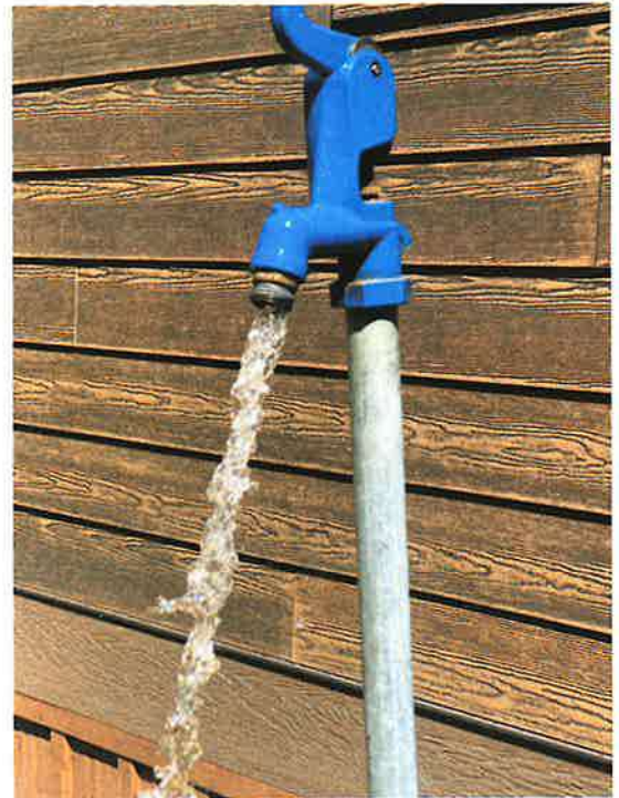
POU: A frost-free outdoor faucet at the house supplies water to the yard and garden via a hose connection.
