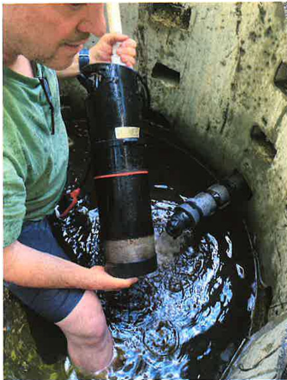
POD: Diversion pump intake equipped with fish screen inside culvert. Pump disconnected from 1" pipe for photo clarity.
