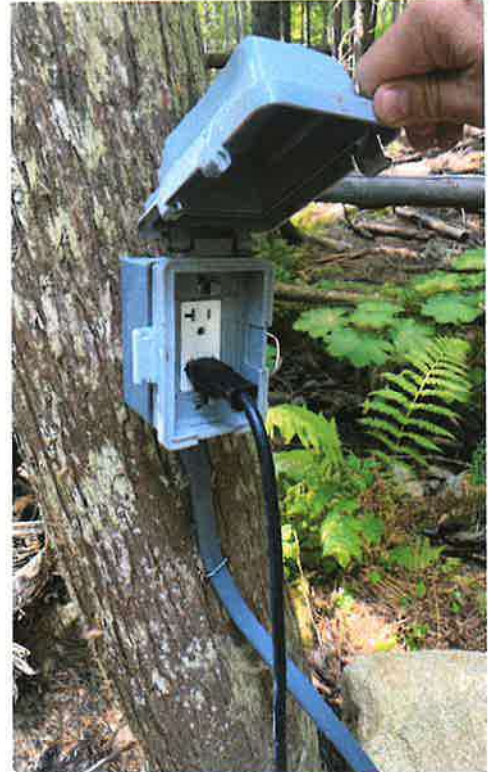
POD: Electrical box supplying power to the pump.
