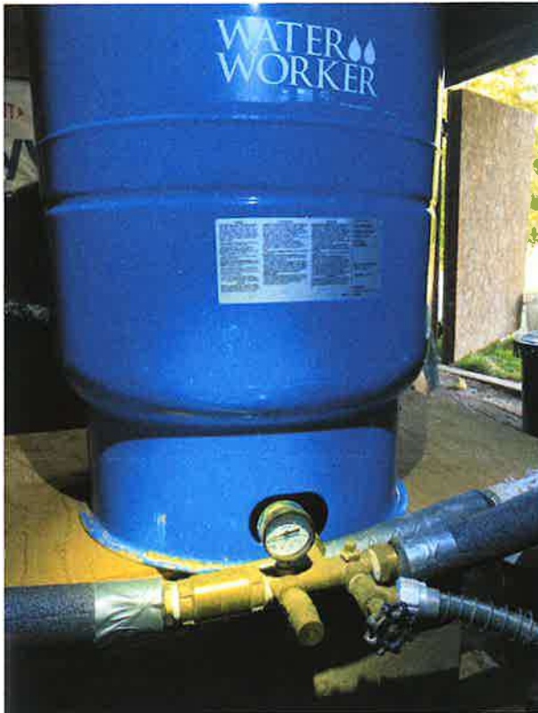
POU: Water is transported via the 1-inch supply line into a 44-gallon pressure tank, which then distributes water throughout the house.
