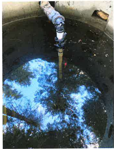
POD: Water is pumped using a dedicated Grundfos pump and transported directly to the home via a 1-inch main water line.
