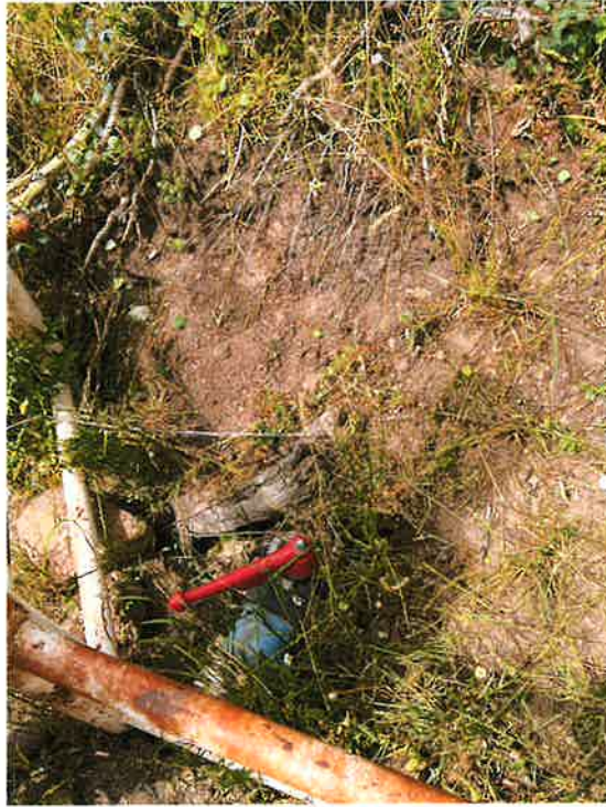
Photo 3: South pond valve to pipeline.
