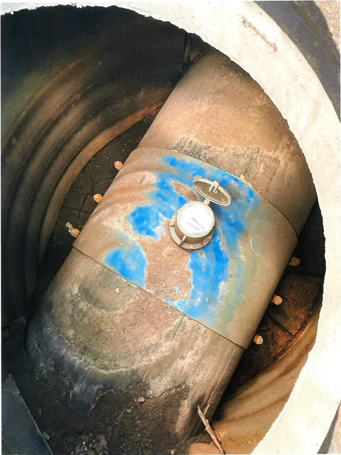
Photo 3: Flow meter on 30" HDPE pipe.
