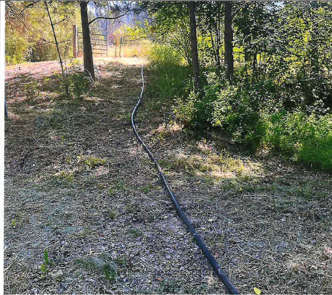
Figure 4. Facing northeast and away from the pump, the piping that carries water to the POU
