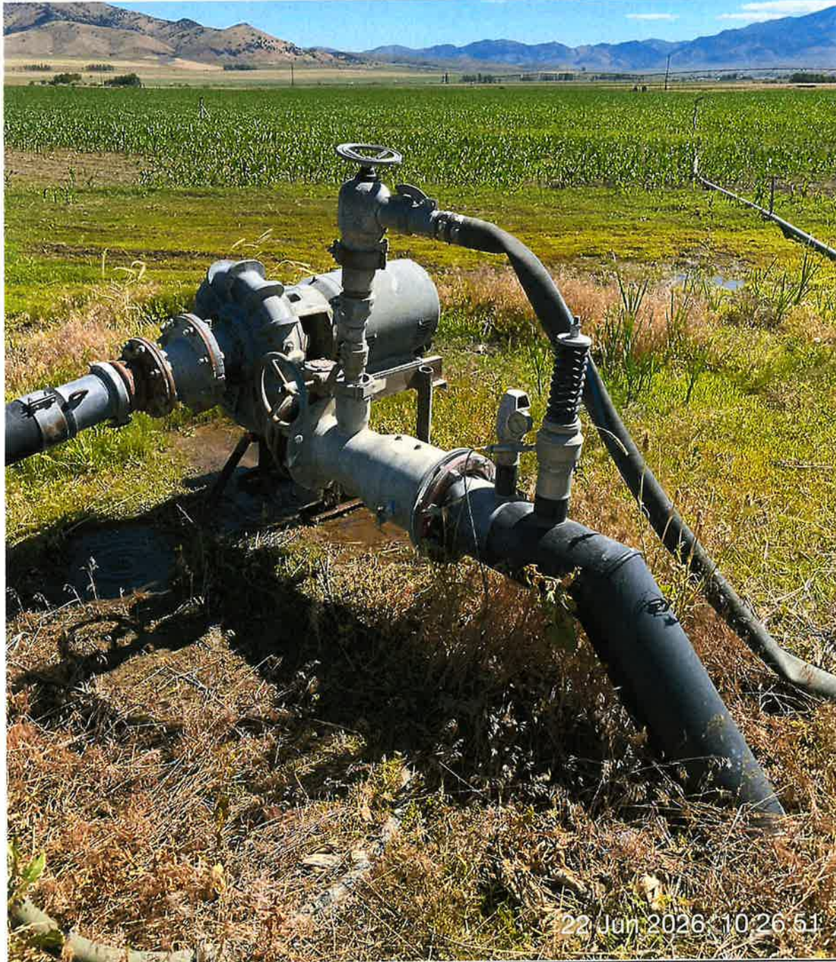
Pump station delivering surface water from St Johns Irrigating Co into the interconnected mainline.
