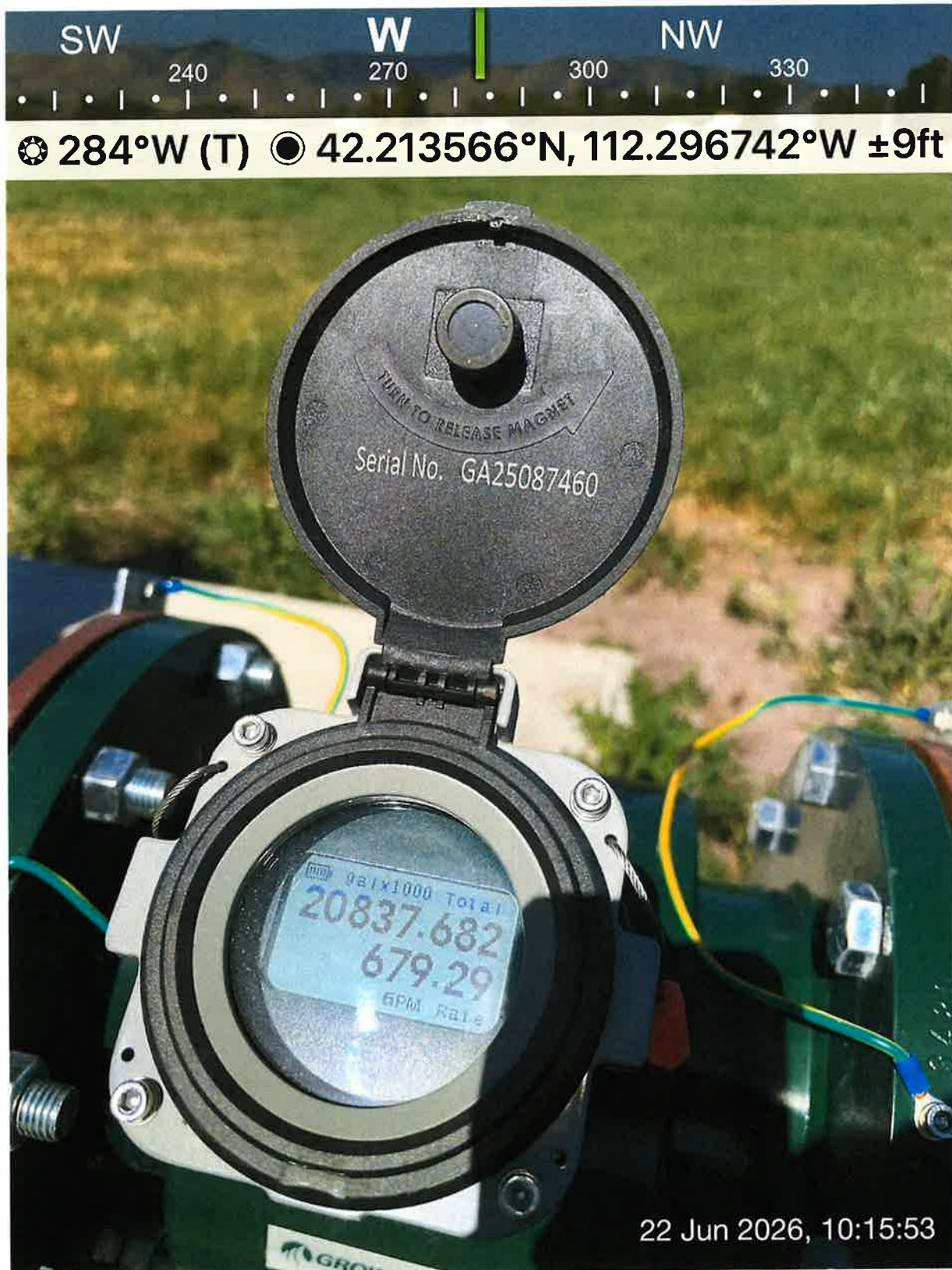
Flowmeter displaying 679 gpm
