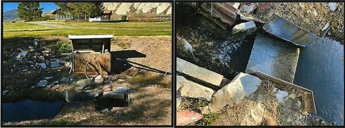
Photos 5 & 6- Fish screen weir in the lateral with intakes entering the pump doghouse on the northeast side of the POU next to the road. 3" poly discharge is exposed for about 4ft then buried entering the POU to the southeast.
