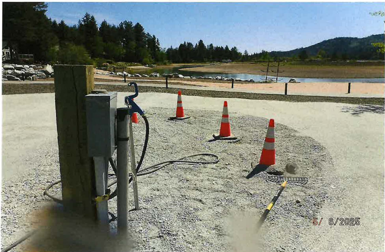
DOMESTIC POU – LOT 4; LANDINGS SUBDIVISION DEDICATED POWER / WATER / SEWER CONNECTION FOR RV USE PAD CURRENTLY BEING UPDATED FOR ROCK AND LANDSCAPING
