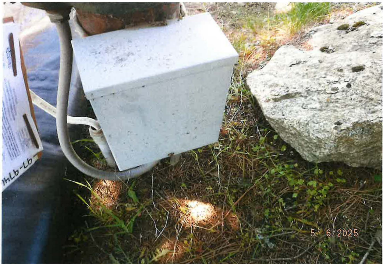
WELL PUMP MOTOR RELAY CONTROL PANEL – NON-DESCRIPT NO LABELING ON PANEL
