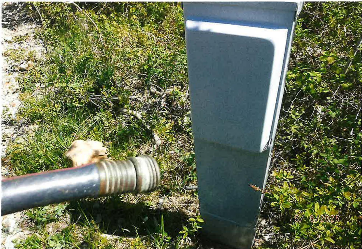
DEDICATED POWER AND WATER CONNECTION FOR LOT 6.
