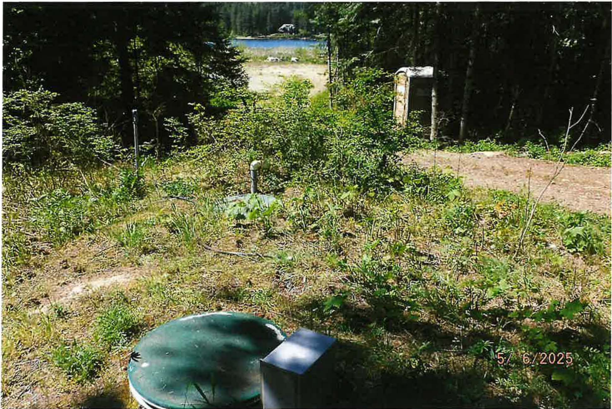
WATER CONVEYANCE SYSTEM – INCORPORATES A 2,500-GAL STORAGE RESERVOIR WITH 1-HP DISTRIBUTION PUMP FROM TANK
