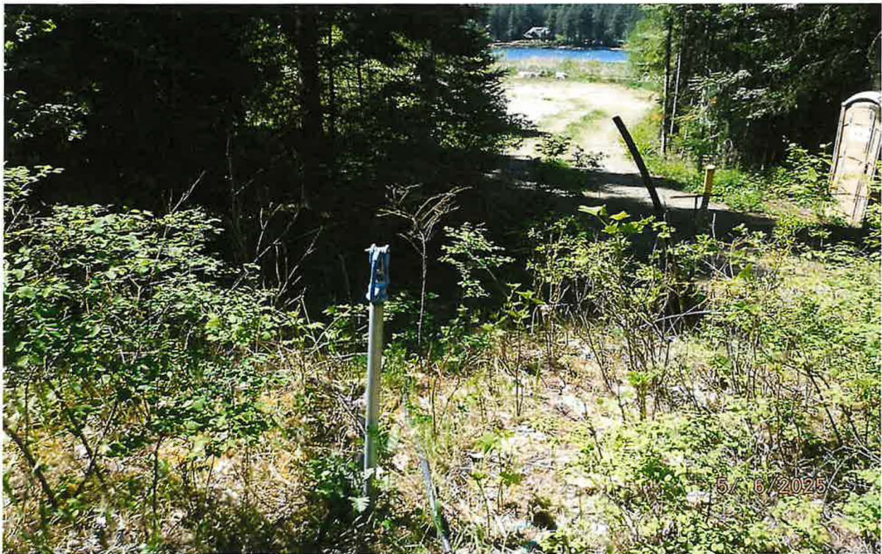
DOMESTIC POU – FROST-FREE HYDRANT AND HOSE ROUTED DOWN TO RV PAD FOR LOT 6; LANDINGS SUBDIVISION
