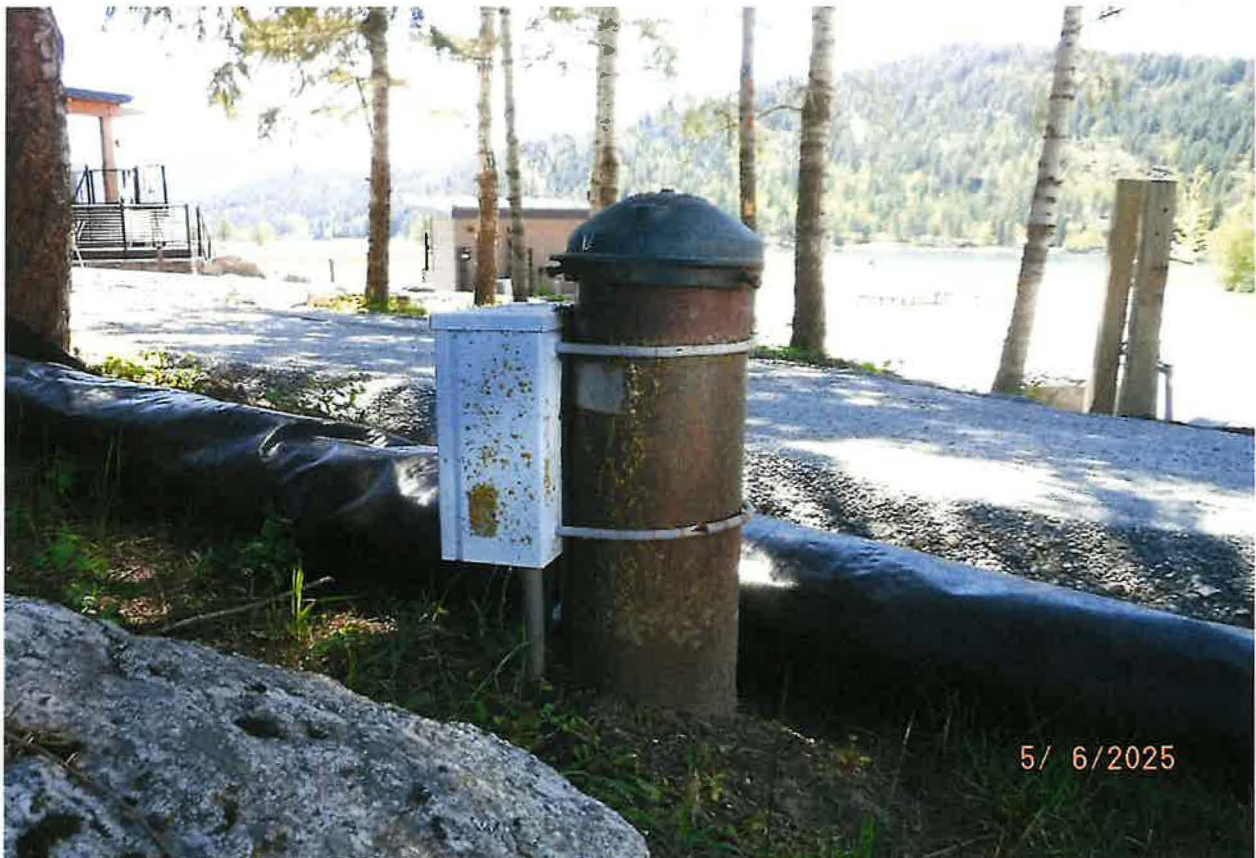
POD – CASED GROUND WATER WELL WITH 1.5 HP PUMP INSTALLED
