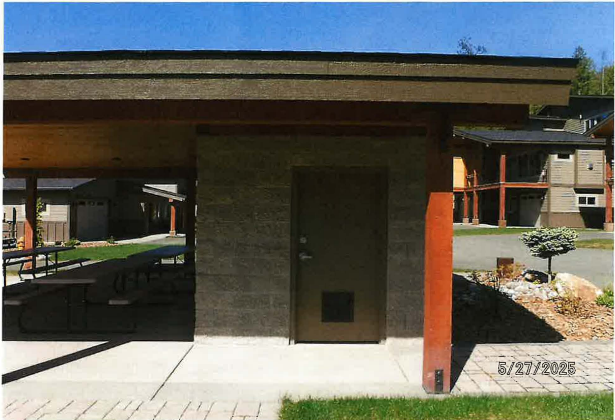
DOMESTIC POU – 2EA COMMUNITY RESTROOMS; LOCATED IN COMMON AREA NEXT TO TENNIS/BASKET BALL COURT & BBQ PAD
