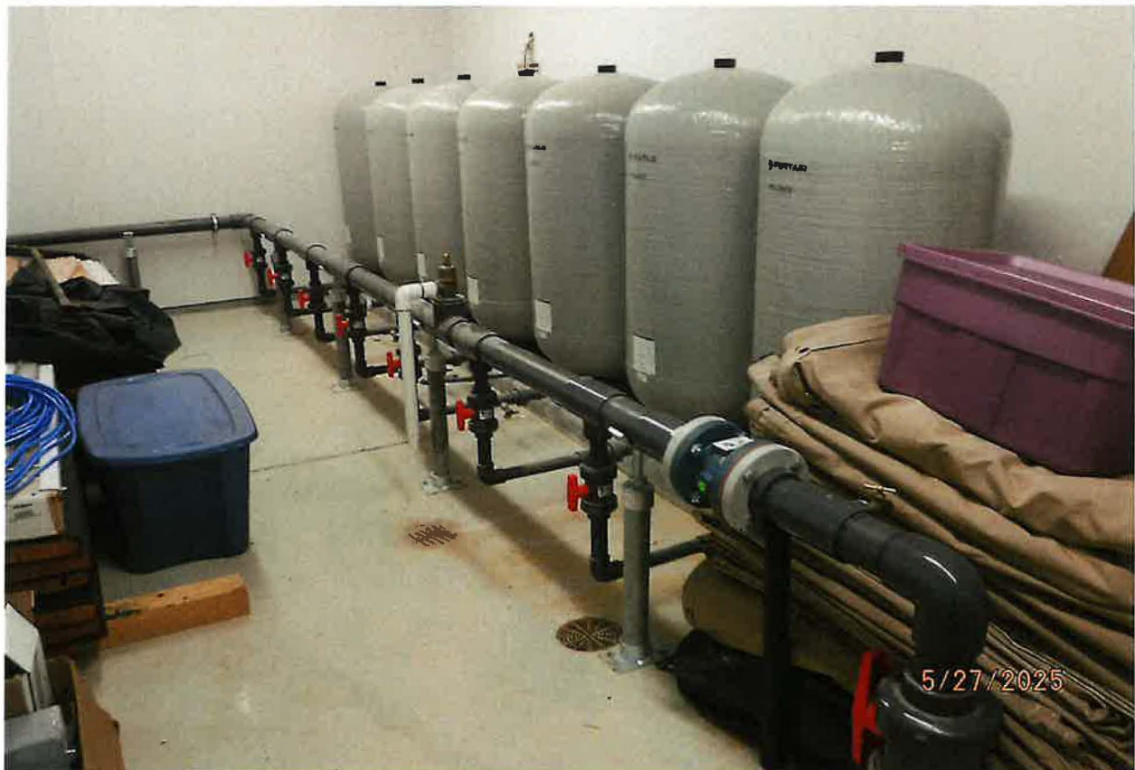
CONVEYANCE SYSTEM – 2-INCH PIPELINE INFLUENCED BY 7 PRESSURE TANKES PRIOR TO EXITING PUMP STATION FOR DISTRIBUTION TO DOMESTIC USES
