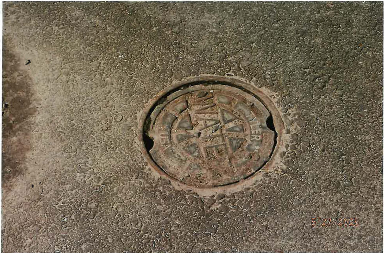
WATER CONVEYANCE SYSTEM – MAIN WATER SERVICE PIPELINE ROUTES DOWN PAVED DRIVE WITH LATERAL STUB SERVICE LINES TO EACH RESIDENCE (21 TOTAL + 2 RESTROOMS)
