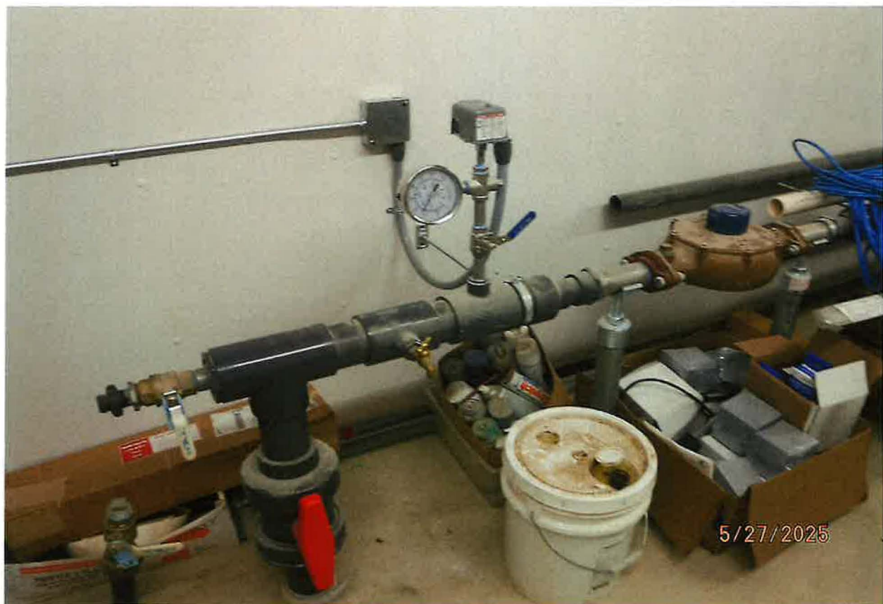
CONVEYANCE SYSTEM – INTAKE PIPE WITH RED MANUAL VALVE HANDLE ENTERS PUMP STATION ROUTING THROUGH A FLOW METER PRIOR TO DISTRIBUTION
