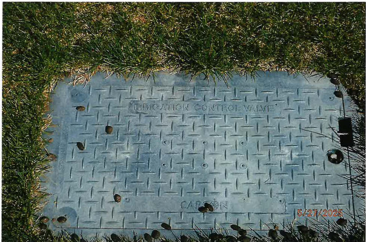
EXAMPLE IRRIGATION ZONE CONTROL BOXES
