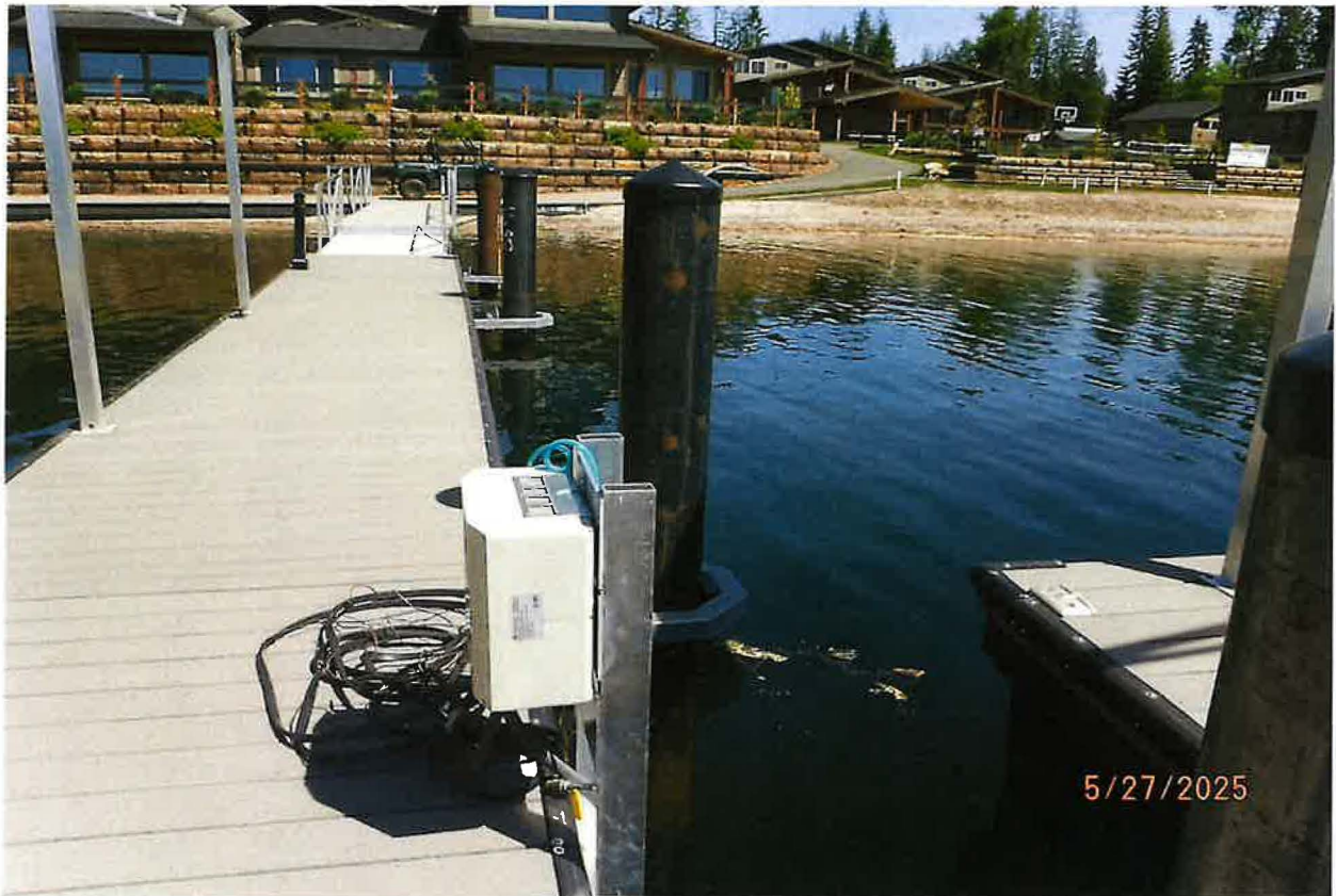
POD – LAKE PUMP WITH VIEW TO SHORE
