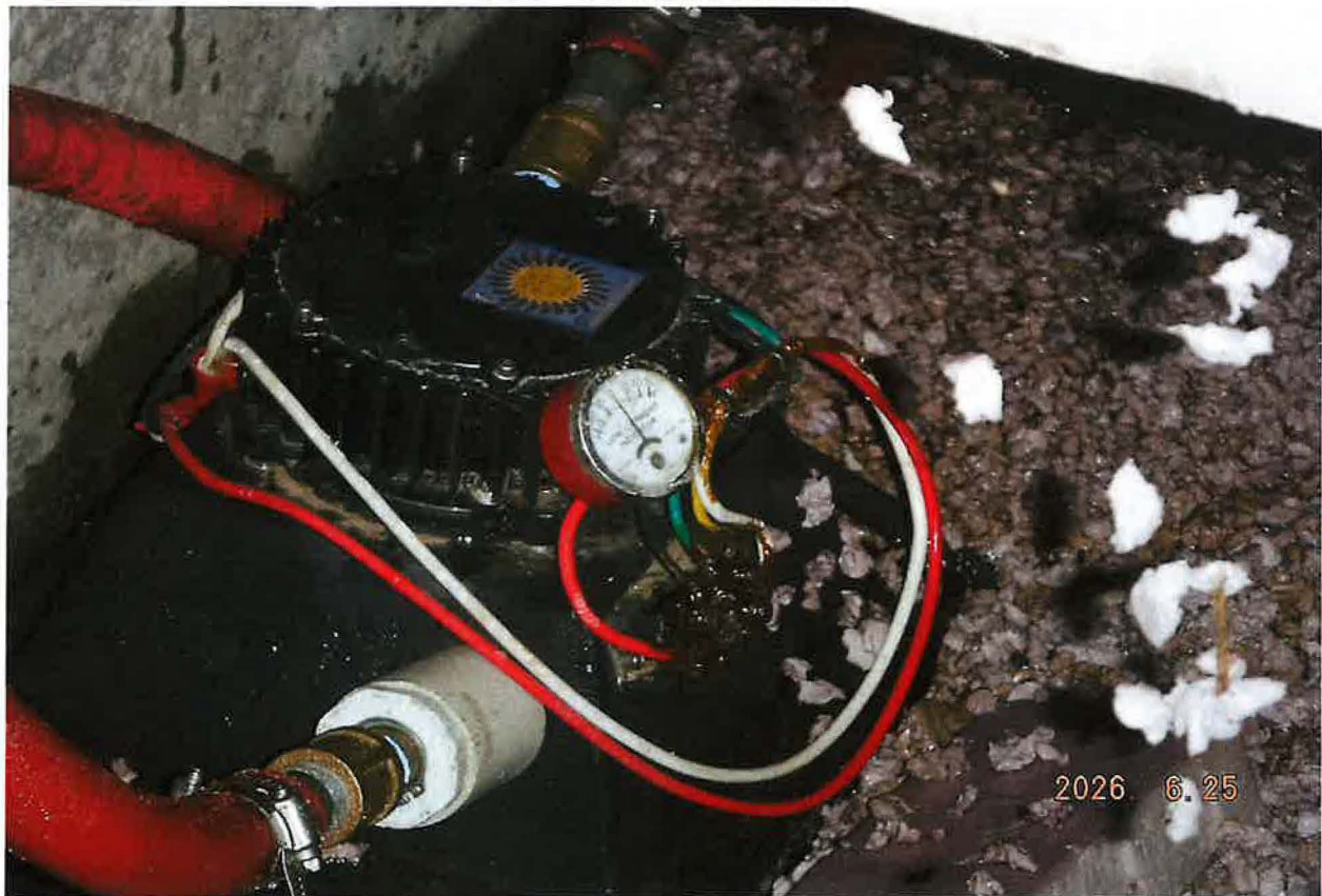
POWER UNIT – HOME HYDRO/HYDRO INDUCTION POWER BRAND MICRO-HYDRO WITH 2EA ¼ - INCH NOZZLES INSTALLED.
