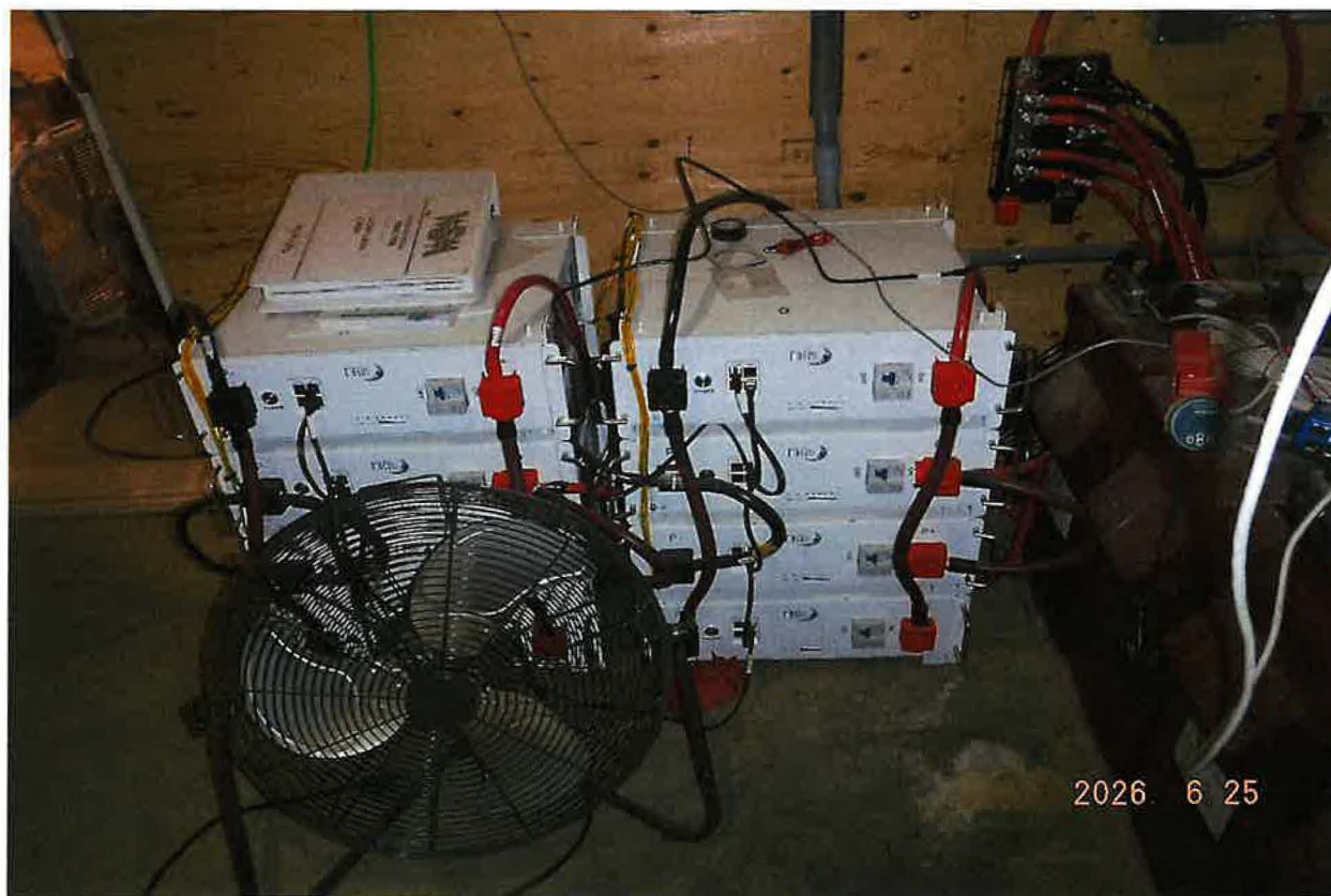
MICRO HYDRO POWER BATTERY BANK (WHITE) – NOTE SOLAR BATTERY BANK ON R/H SIDE OF IMAGE; RIGHT HOLDER USES DUAL ENERGY SOURCES.
