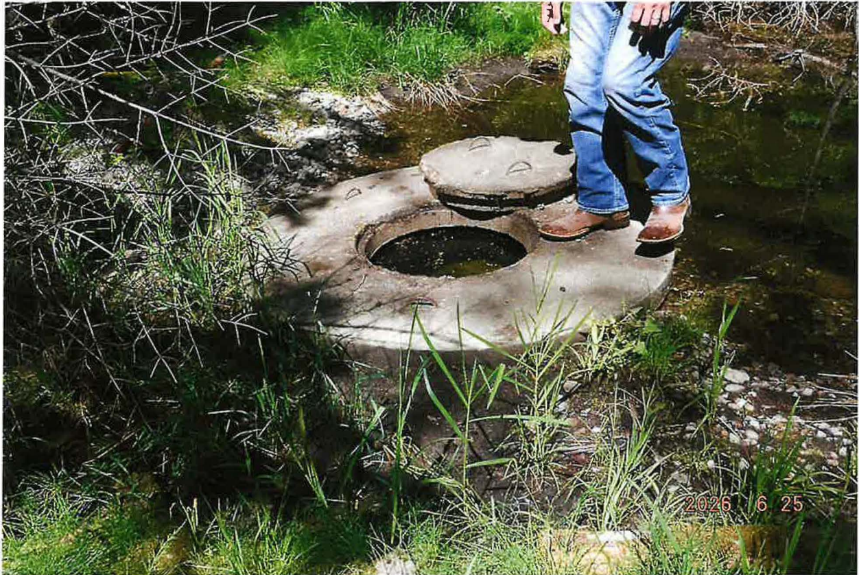
POD – DRY WELL WITH SCREENED INTAKE CONSTRUCTED INSTREAM POOL
