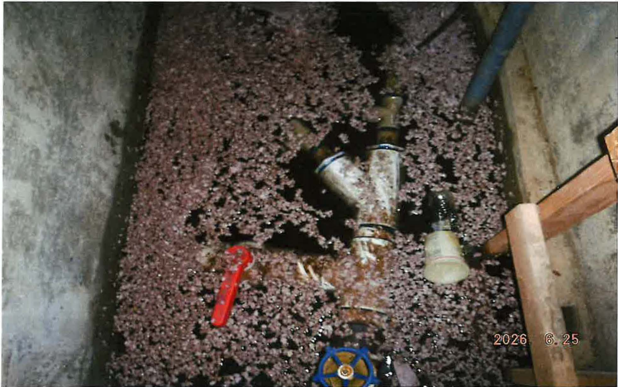
POWER UNIT INFRASTRUCTURE UNDER WATER AT TIME OF EXAM WITHIN CONCRETE CONTAINMENT – REFERENCE STATEMENT OF COMPLETION BACKFILE FOR IMAGES PROVIDED BY RIGHT HOLDER OF WATER SYSTEM
