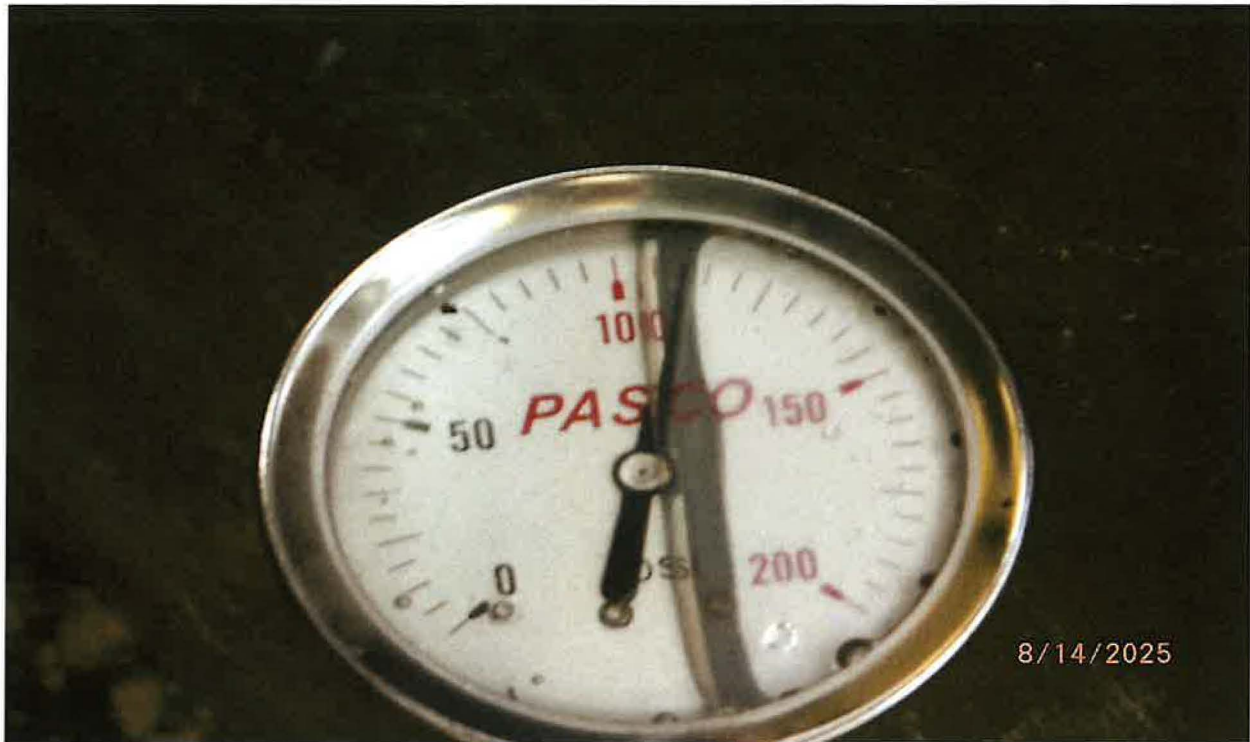
WATER SYSTEM OPERATES AT 110 PSI WITH ALL IRRIGATION RISERS IN OPERATION (NOT NORMAL); NORMAL OPERATION USES A SINGLE SPRINKLER ON AT A TIME
