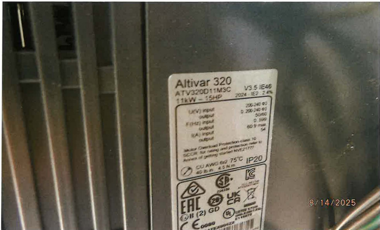
ALTIVAR 320 PUMP MOTOR RELAY CONTROL PANEL – CAPABLE TO PAIR WITH UP TO 15 HP PUMP END. SYSTEM USES A 7.5 HP PUMP END.
