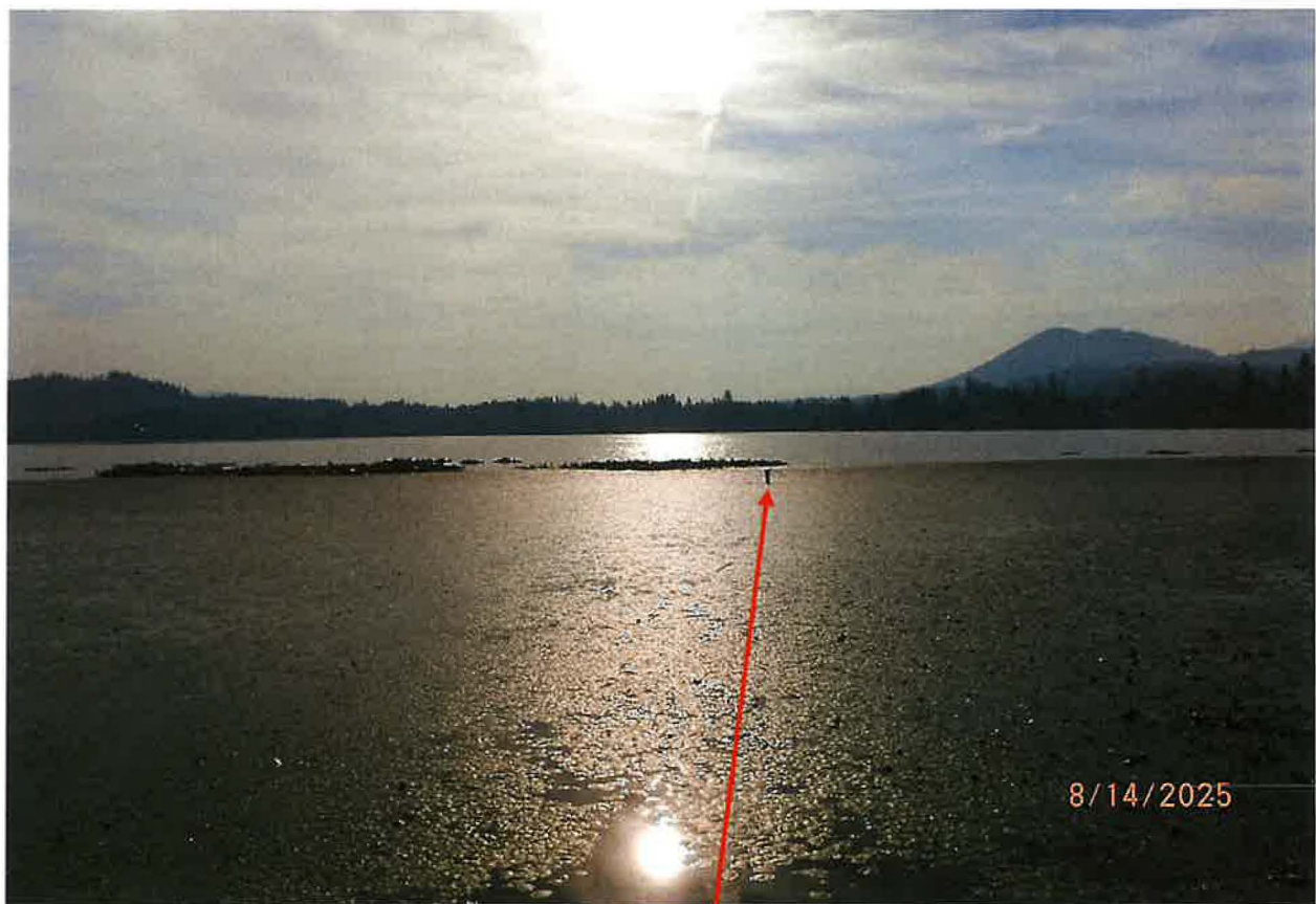
POD – SUBMERSIBLE 7.5 HP GOULDS PUMP IN ROSE LAKE (THIN BOUEY IN CENTER PORTION OF PHOTOGRAPH)
