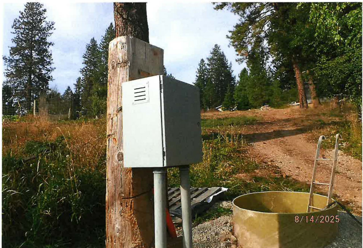
WATER CONVEYANCE SYSTEM – PUMP MOTOR CONTROL PANEL AND SEMI-VAULTED VALVE CONTROLS WITH FLOW METER
