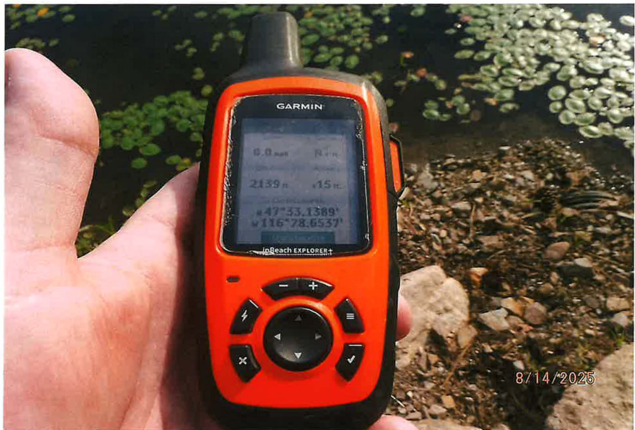
2-INCH INTAKE PIPE COMES TO SHORE AS A BURIED PIPELINE (SEE R/H SIDE OF IMAGE 2-INCH POLYPIPE ROUTED IN CORRUGATED SHIELDING PIPE)
