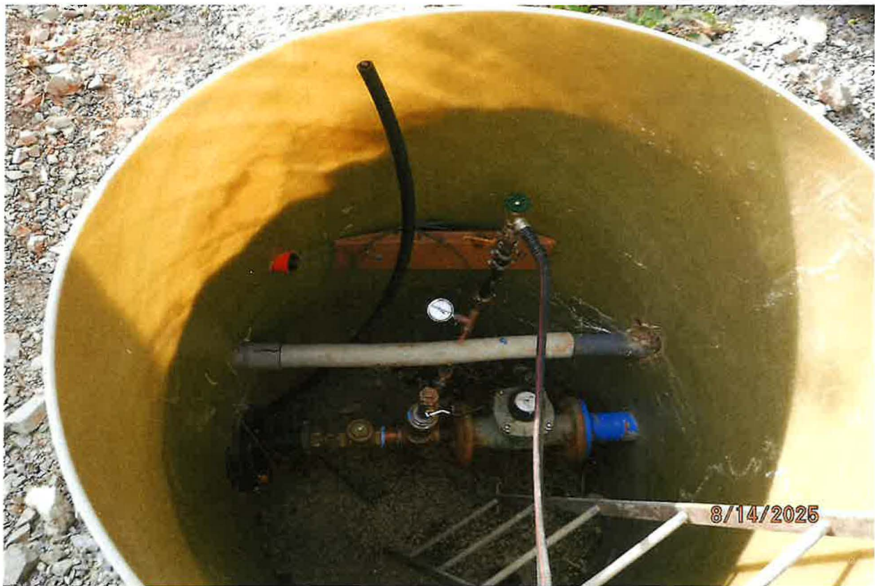
WATER SYSTEM INCLUDES AN INSTALLED FLOW METER AND CHANGES FROM 2-INCH INTAKE PIPELINE TO 4-INCH BURIED MAIN WATER LINE ROUTED TO IRRIGATION POU
