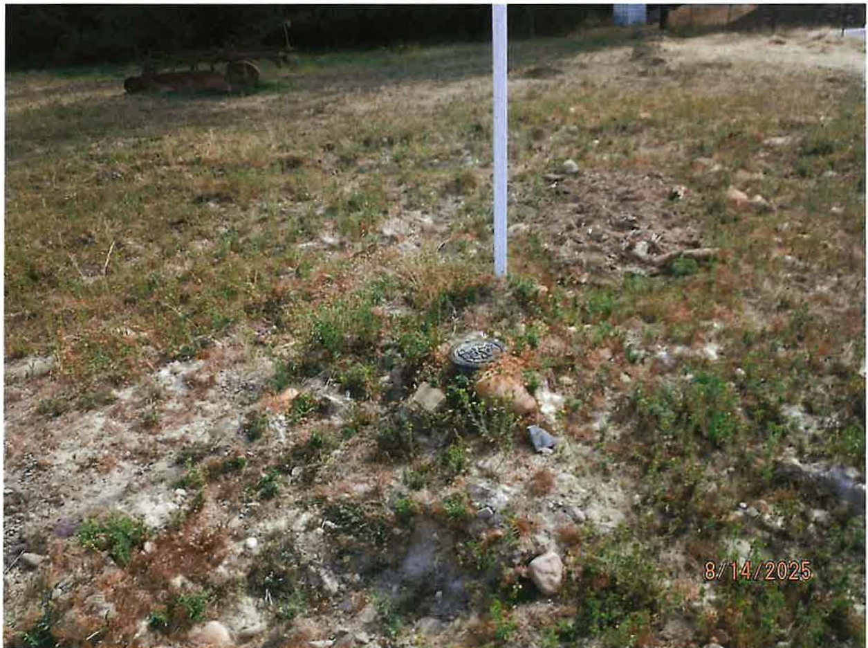
WATER LINE VALVE CONTROL PIPE
