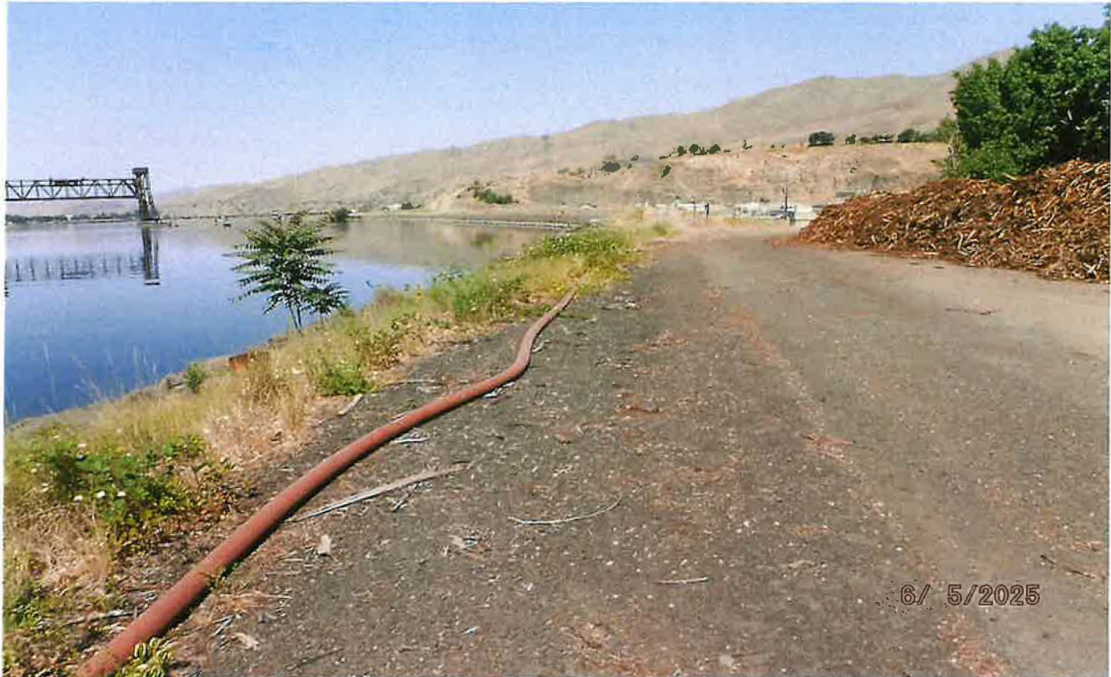
WATER CONVEYANCE SYSTEM – 4 INCH FLEXIBLE PIPELINE TO LOG YARD INDUSTRIAL WATERING
