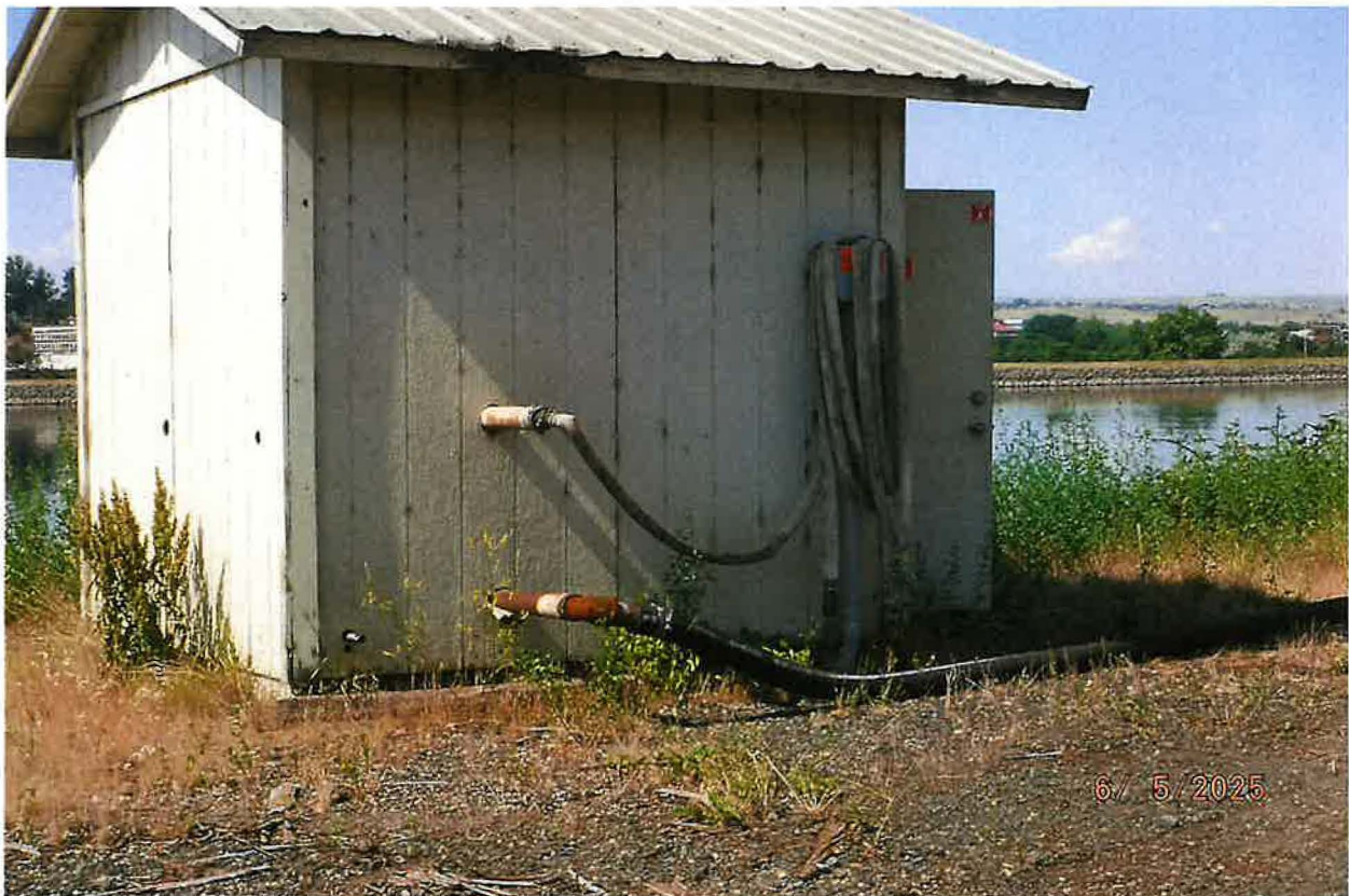
PUMP STATION WITH DISTRIBUTION SIDE HOSE CONNECTIONS – LOWER 4-INCH FLEXIBLE PIPELINE TO 4EA TOWER BIG GUN SPRINKLERS; UPPER FLEXIBLE 1.5 INCH FIRE HOSE CONNECTION WHICH ROUTES TO INDIVIDUAL SMALLER BRASS IMPACT SPRINKLERS
