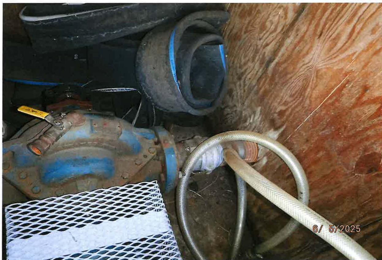
DIVERTING WORKS – INTAKE PIPELINE SUCTION PUMP END (INSIDE PUMP STATION)
