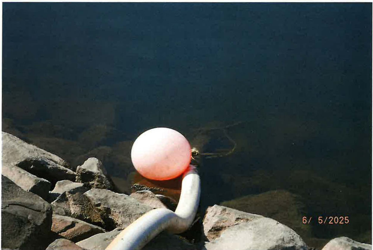
POD – FLEXIBLE INTAKE PIPE WITH 3/32 ND INCH SCREEN IN THE CLEARWATER RIVER
