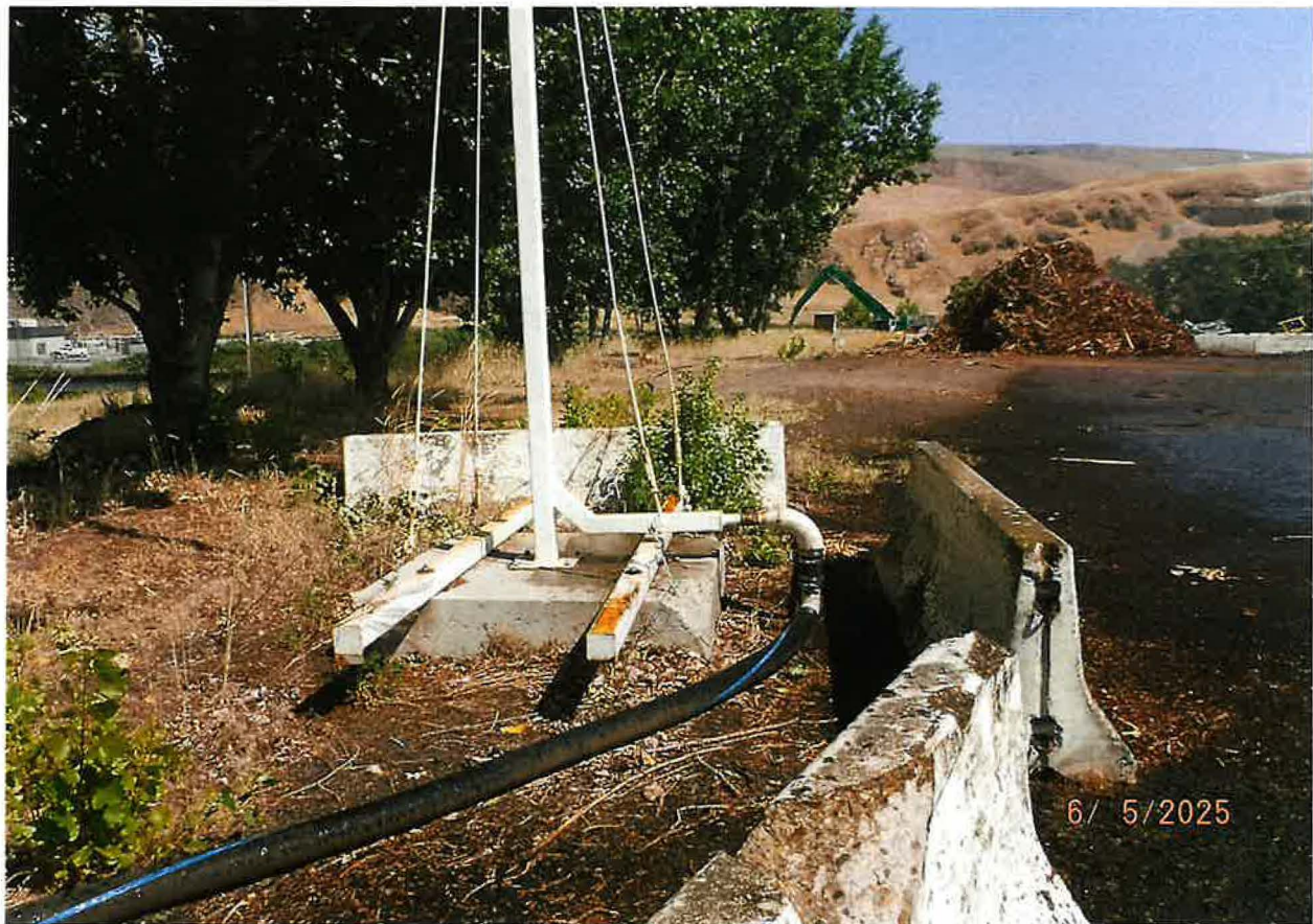
INDUSTRIAL POU – 1 OF 4 RISER PIPES TO BIG GUN SPRINKLERS
