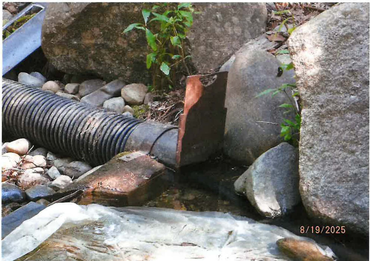
POD – TWENTY MILE CREEK DIVERSION & DIVERSION TO STORAGE – 8 – INCH CORRUGATED POLY PIPE WITH STEEL PLATE HEADGATE DEVICE
