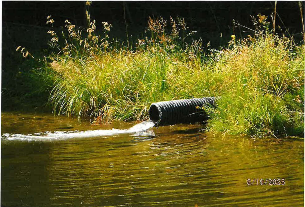
RECREATION POU – INFLOW TO EASTERN MOST STORAGE POND #1 (COVERED UNDER RIGHT 98-7937)
