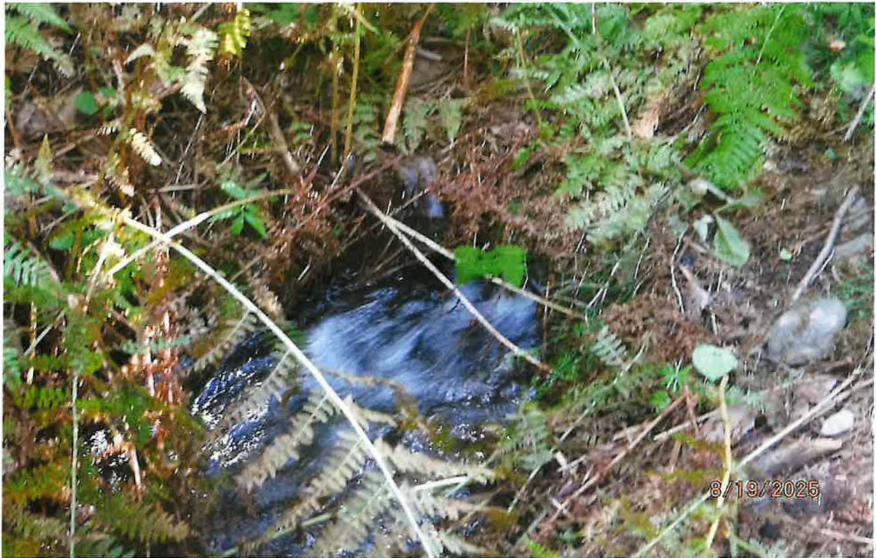
56-FT OF 8-INCH CORRUGATED POLY PIPE TRANSITIONS TO OPEN DITCH SERVING AS DIVERSION TO STORAGE CONVEYANCE SYSTEM OFF TWENTY MILE CREEK
