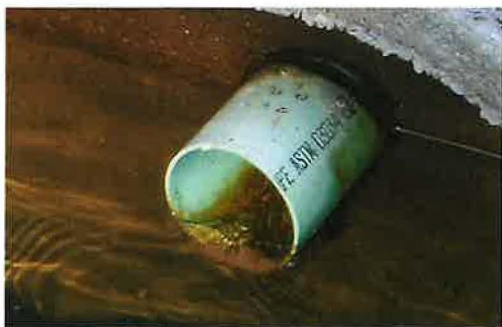
Overflow pipe with stained flow line interior of pipe
