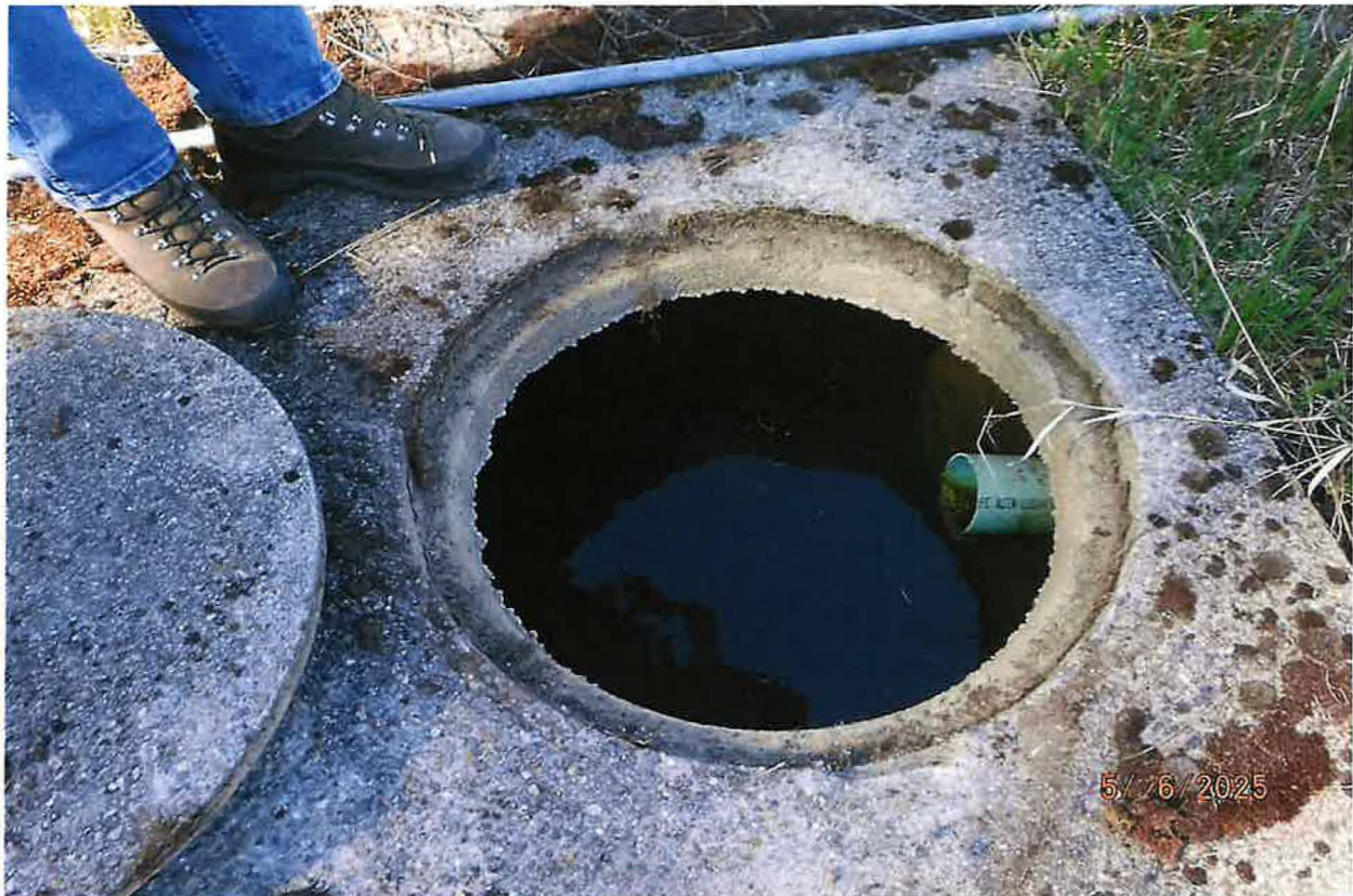
CONVEYANCE SYSTEM – 3-INCH OVERFLOW PIPE FROM TOP OF CISTERN ROUTES APPROXIMATELY 420-FT OPEN DISCHARGING TO FILL STORAGE POND
