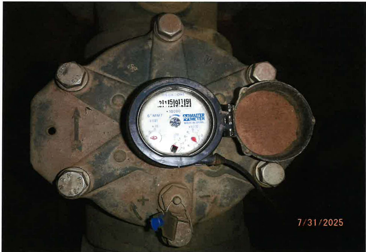
MASTER METER FLANGED VELOCITY STYLE FLOW METER INSTALLED ON MAIN DISTRIBUTION PIPELINE BEFORE PUMPING ROUTES TO DIFFERENT STORAGE PONDS FOR DISTRIBUTION.
