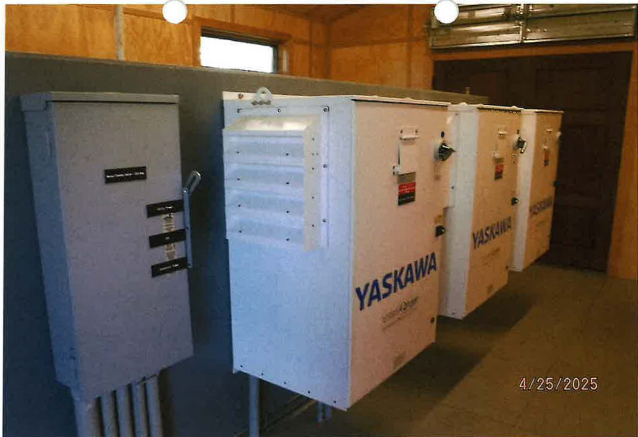
DISTRIBUTION PUMP RELAY CONTROL PANELS
