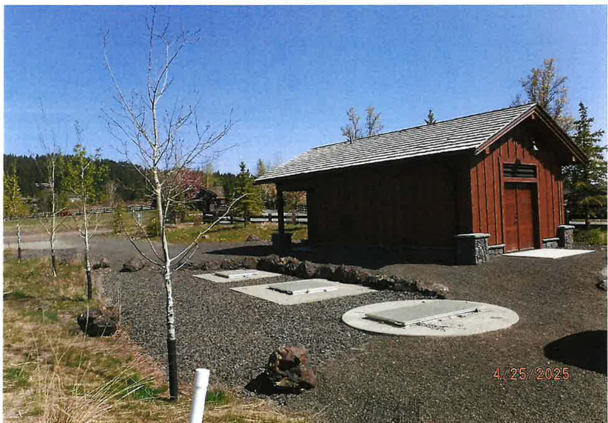
MUNICIPAL STORAGE DISTRIBUTION STATION – WET WELLS INCLUDED IN FORE FRONT OF IMAGE (DISTRIBUTION PUMPS No. 1, No. 2, & No.3)
