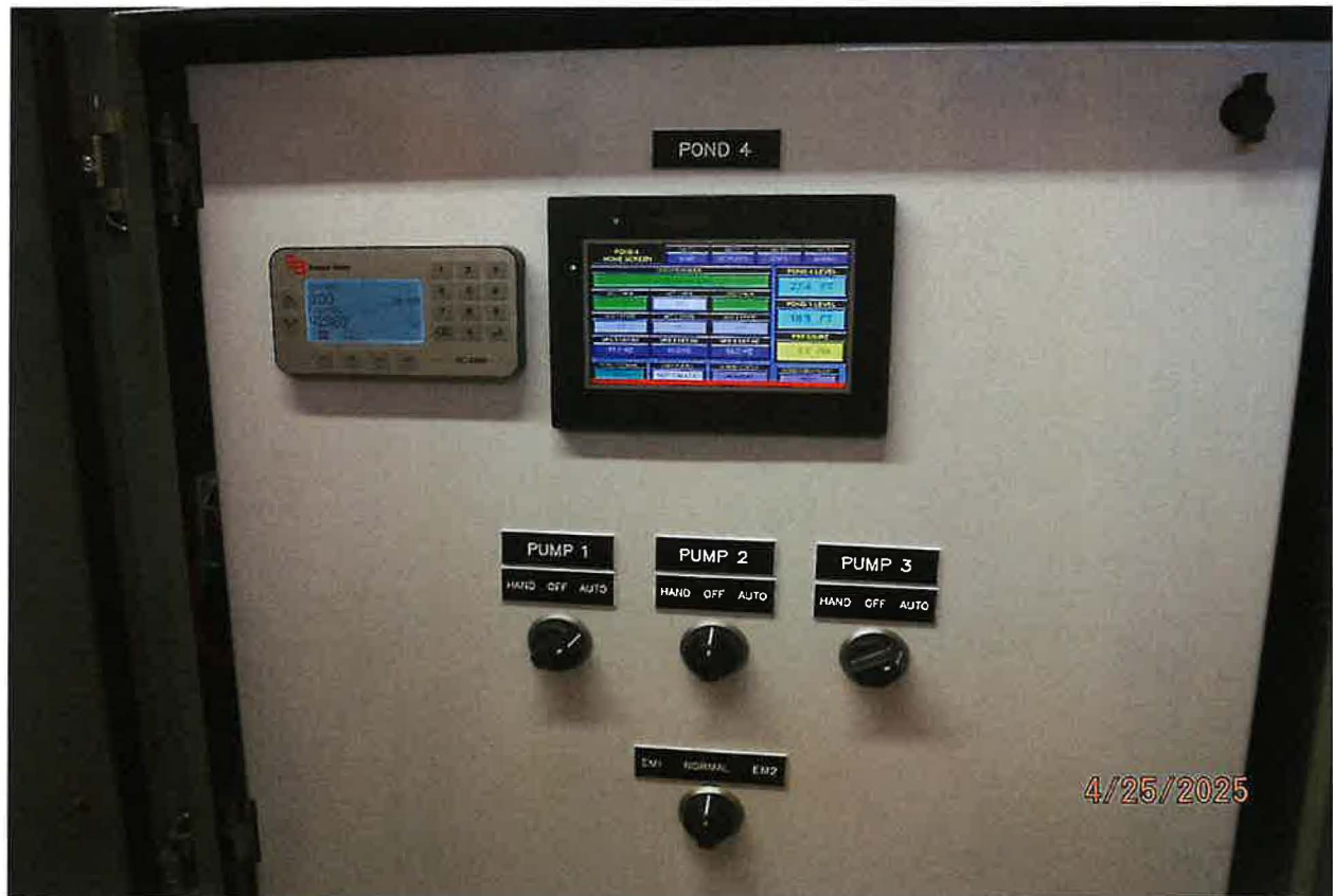
MUNICIPAL FROM STORAGE SCADA SYSTEM MANAGEMENT PANEL
