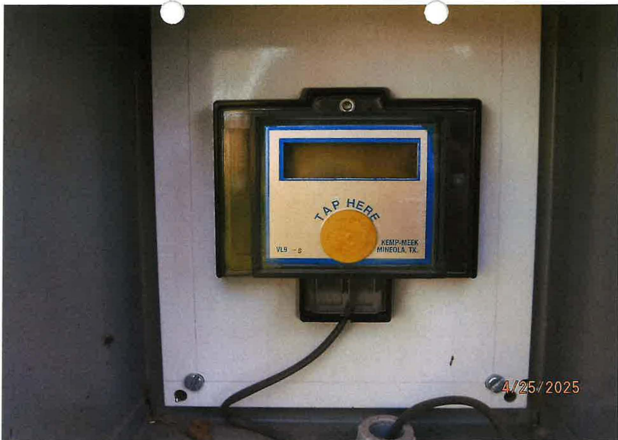
(TAP HERE METER READER CO-LOCATED WITH BOOSTER STATION IN GRASSED DRAIN FIELD)
