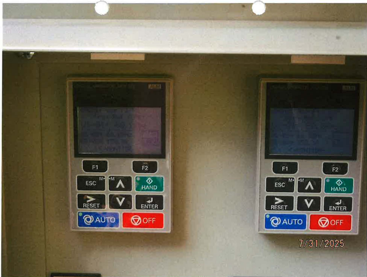
POD – TWO 125 HP VFD DIVERTING PUMPS IN OPERATION DURING SITE VISIT ON 7/31/2025; EACH MOTOR IS SET AT 60.0 Hz
