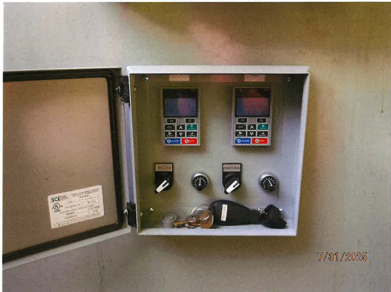
DIVERTING PUMP(S) SYSTEM CONTROL PANEL
