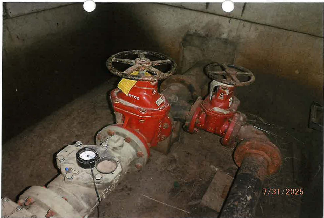
WATER CONVEYANCE SYSTEM – MAIN PIPELINE WITH BYPASS VALVE(S) AND FLOW METER
