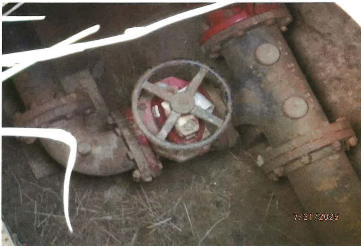
MID WAY PUMP STATION (VAULTED) HOUSES FLOW METER FOR VOLUMETRIC AND INSTANTANEOUS FLOW MEASUREMENTS
