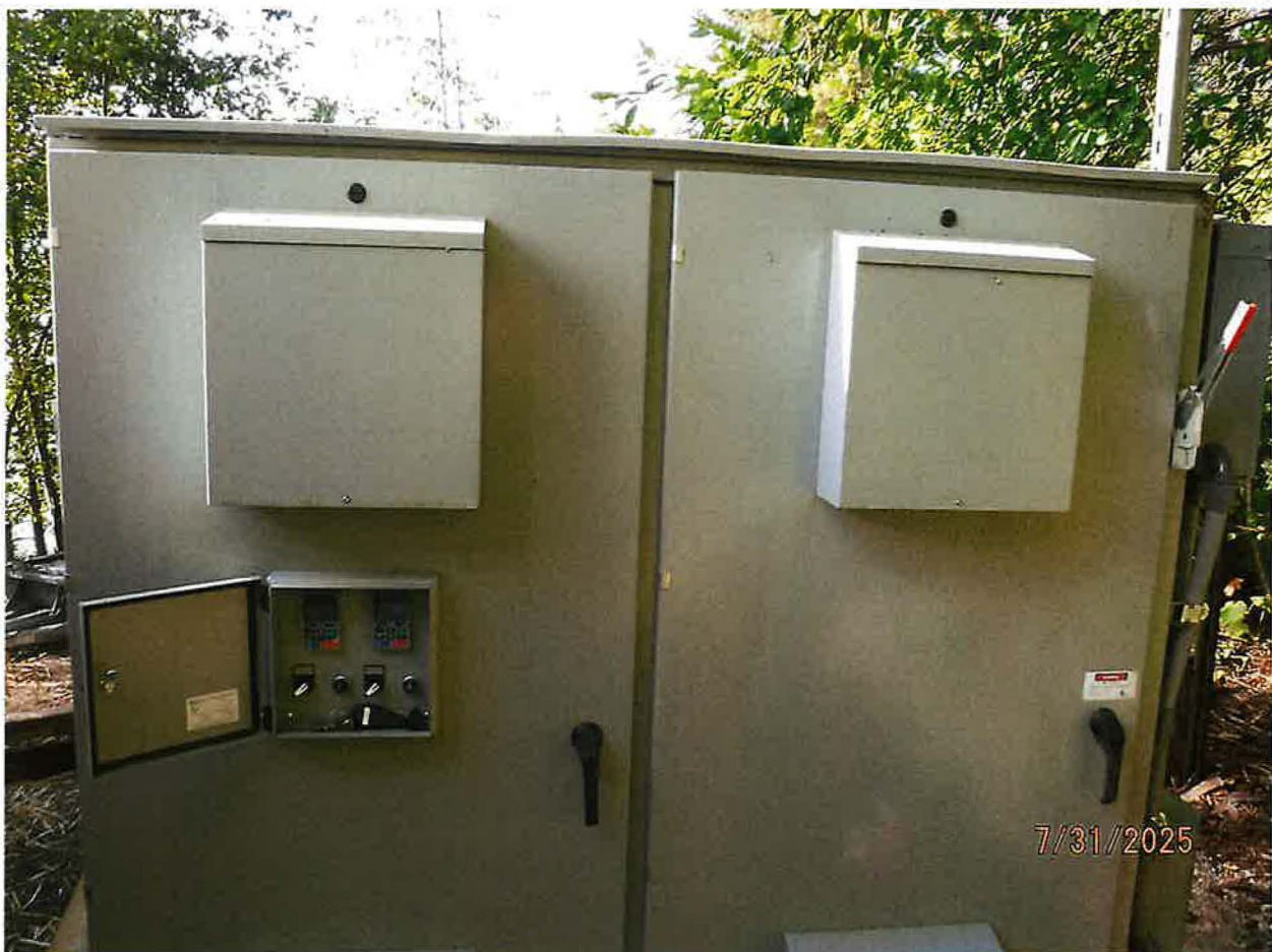
POD- LAKESIDE PUMP STATION HOUSES 2EA DIVERTING PUMP SYSTEM CONTROLS
