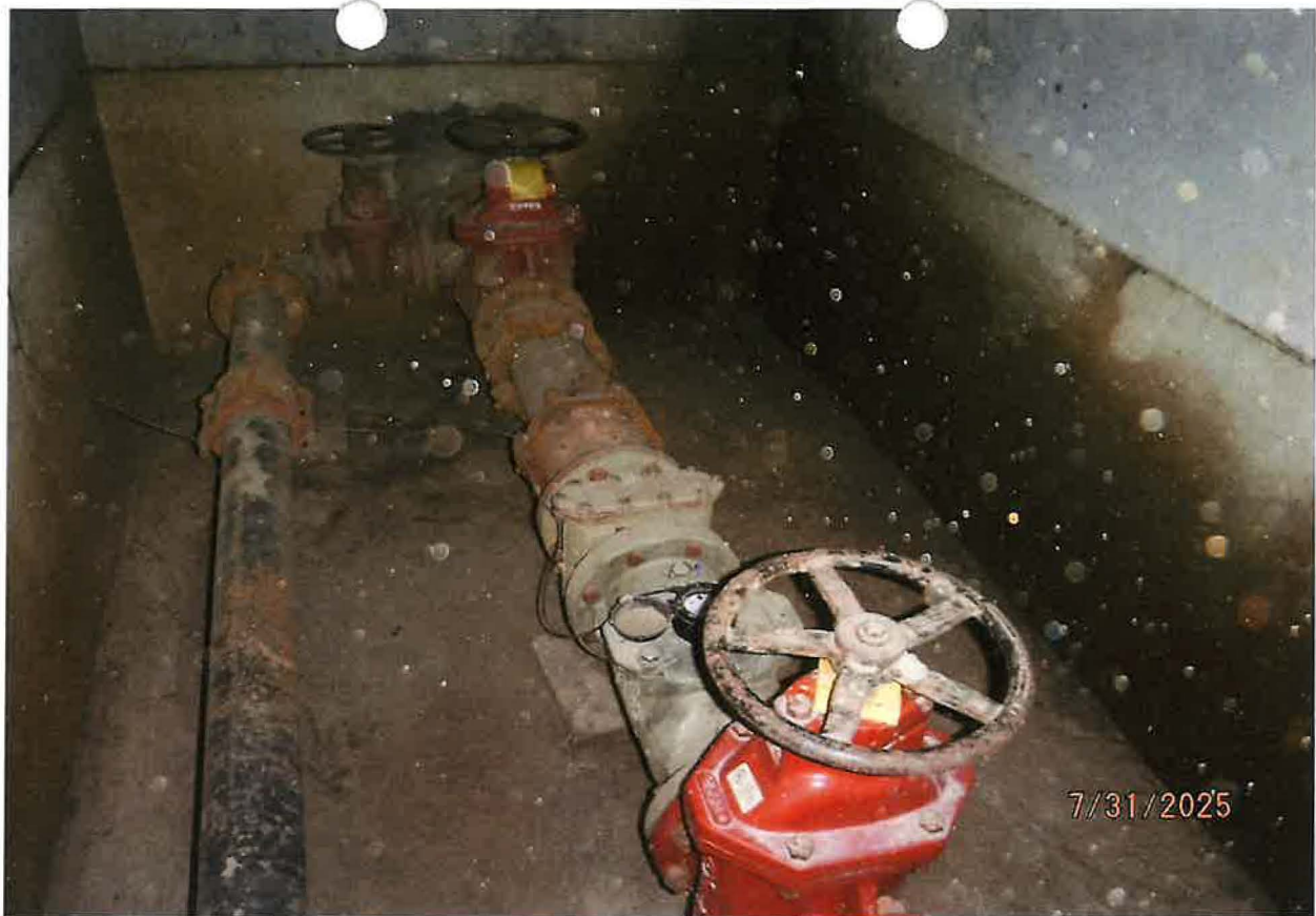
FLOWMETER INSTALLED ON MAIN 12-INCH DISTRIBUTION LINE PRIOR TO BYPASS LINES, WHICH REDUCE TO 6-INCH (VALVING ON TOP OF IMAGE)
