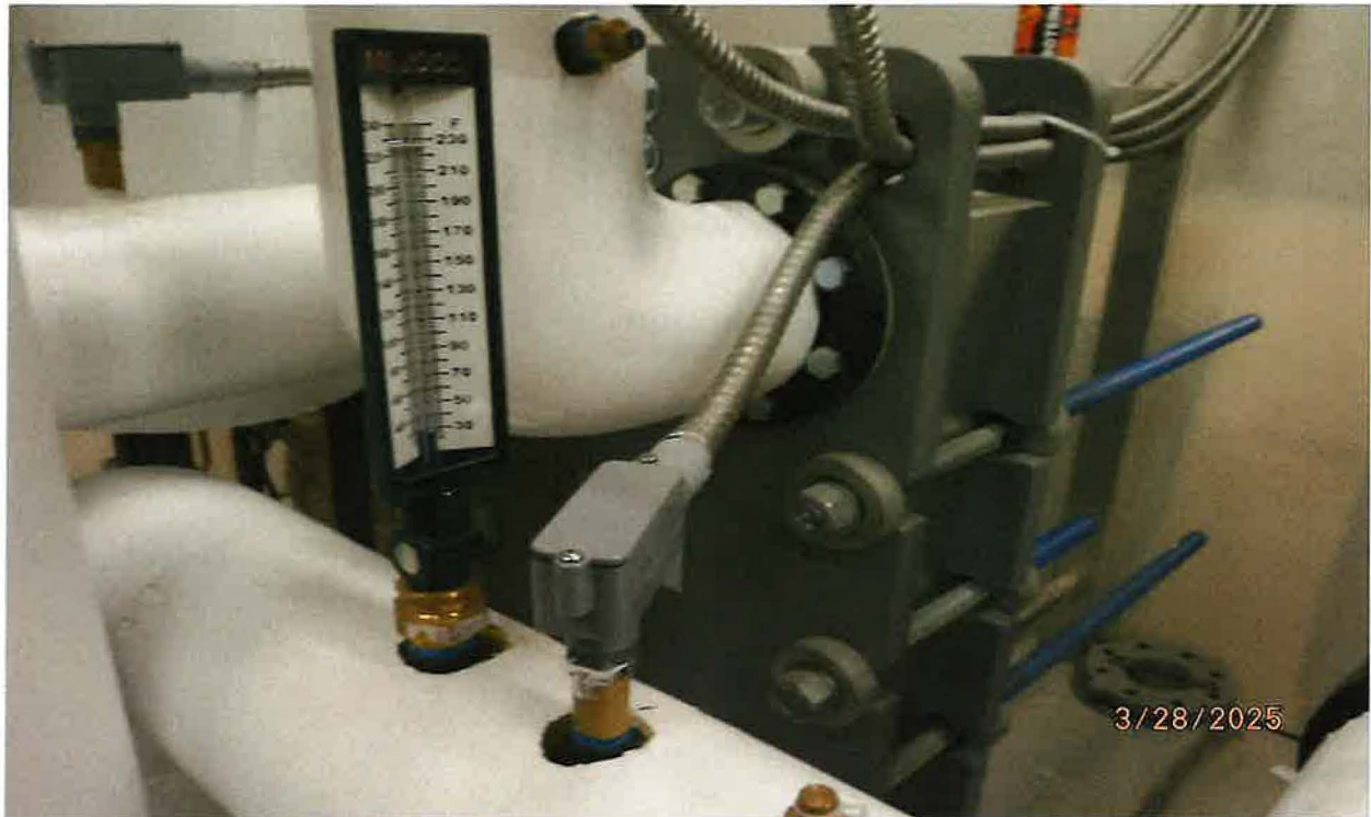
TEMPERATURE PRESSURE SENSORS – HEATING/COOLING SYSTEM OPERATED ON TEMPERATURE DIFFERENTIALS MAINTAINING 70 - 75°F SYSTEM TEMPERATURES
