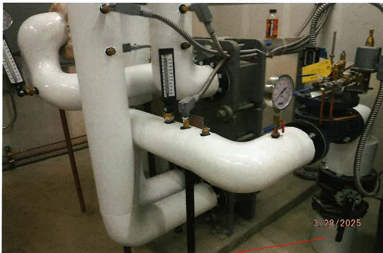
RETURN PIPELINE TO INJECTION WELL
