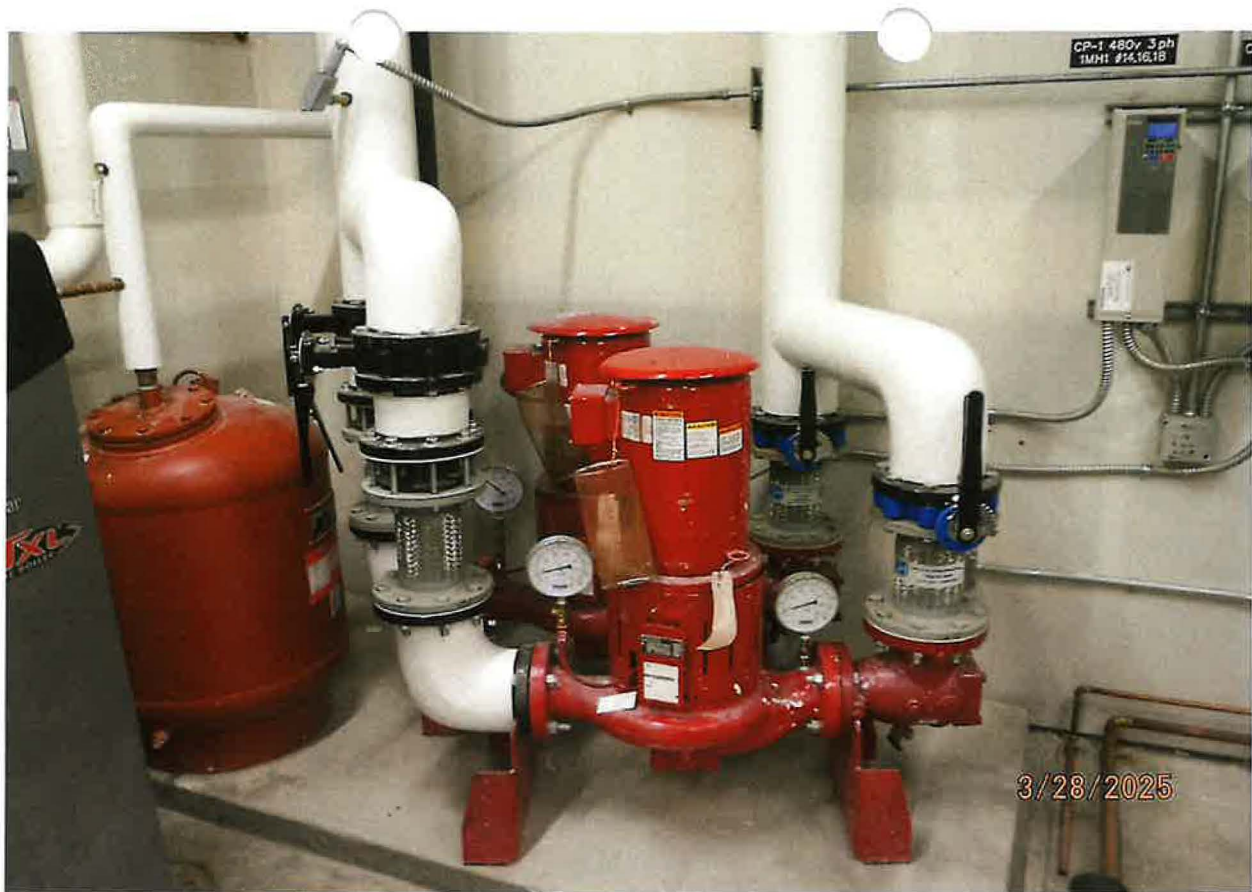
2EA – 10 HP BELL & GROSSETT BRAND LOOP PUMPS UTILIZED WITH BOILER OPERATIONS FOR CLOSED LOOP HEATING/COOLING SYSTEM OPERATION
