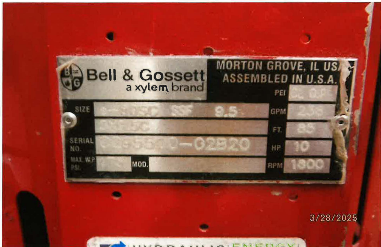
1 OF 2 DATA PLATE FOR 10 HP BOOSTER PUMPS; MODEL NO. KS3011
