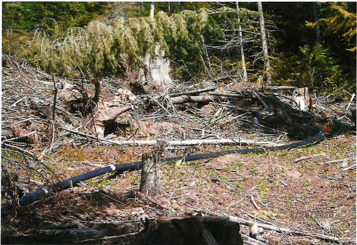
CONVEYANCE SYSTEM – OVERLAND PIPE ROUTED FROM STORAGE RESERVOIR TO FILL POINT
