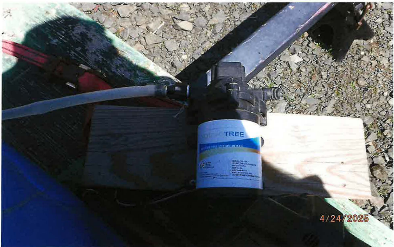
DIVERTING PUMP – PORTABLE 12V/DC WITH BATTERY MOUNTED ON TRAILER
