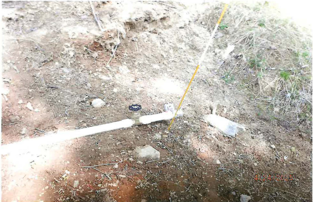
WATER FILL STATION FROM 2,500-GAL STORAGE TANK – PORTABLE TANKS FILLED FOR USE AT OFF-GRID RESIDENCE(S); CO-LOCATED WITH EASTERN MOST COLLECTION POOL
