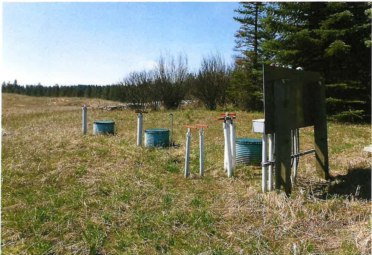
WATER CONVEYANCE SYSTEM – BURIED PIPELINE FROM SPRING TO 3EA – 3,000 GALLON VAULTED STORAGE RESERVOIRS SERVING AS 24-HR IMPOUNDMENT USE.
