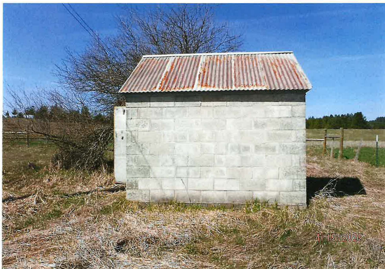
POD – SPRING (7'x 7' x 7') CONCRETE CISTERN CAPTURING SPRING SOURCE WATER
