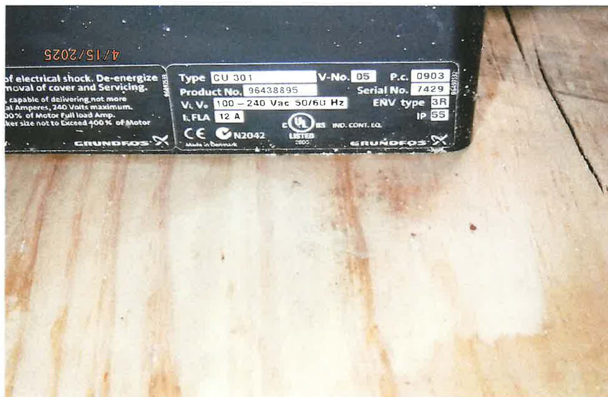
PUMP CONTROL PANEL (IMAGE ROTATED) – GRUNDFOS S/N: 7429.
