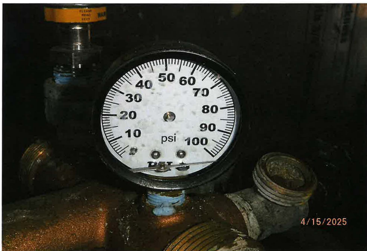
PRESSURE GAUGE KNEEDLE WAS NOT ATTACHED – UNABLE TO SECURE SYSTEM PRESSURE AT TIME OF EXAM
