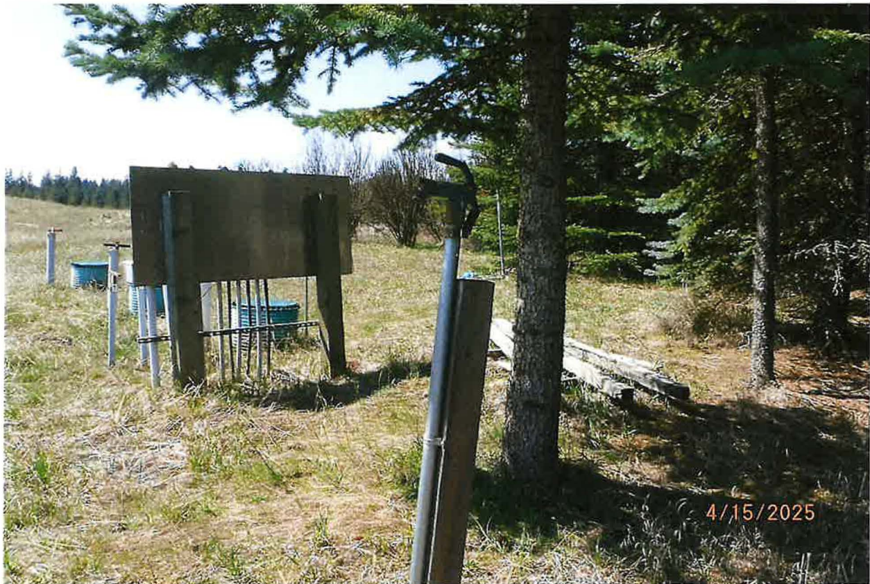
HYDRANT CO-LOCATED WITH STORAGE TANK(S)
