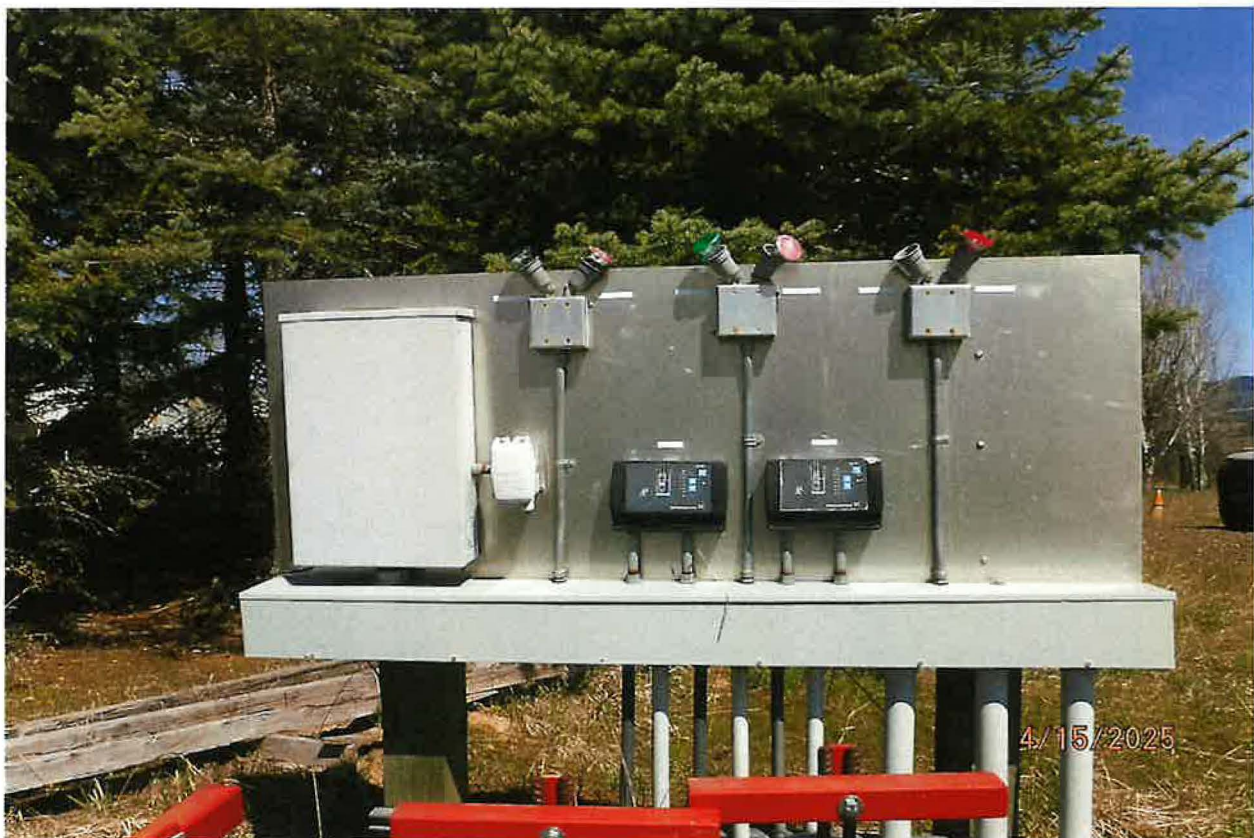
STORAGE TANK CONTROL PANEL TREE – 1 TANK WAS NOT IN USE AT TIME OF INSPECTION (ONLY TWO CONTROL PANELS OPERATIONAL).
