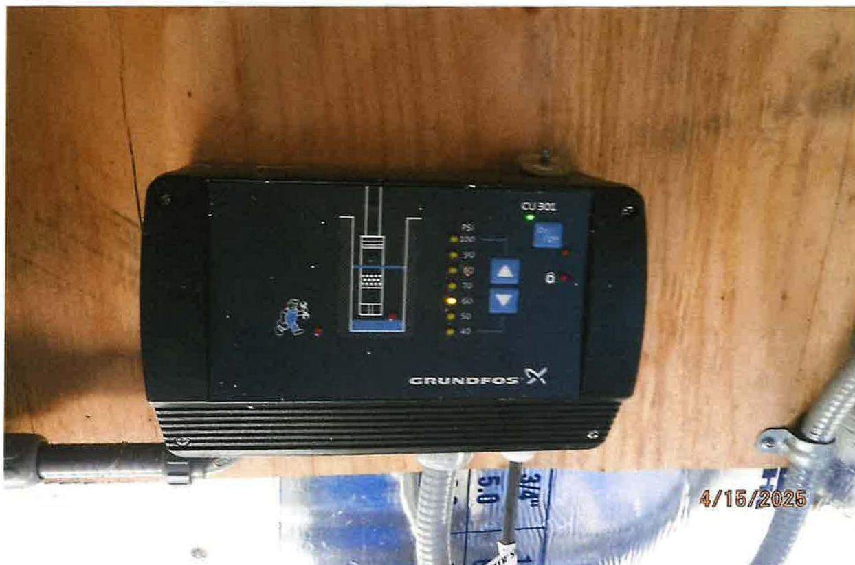
POD – DIVERTING PUMP, UNKNOW HP, WITH GRUNDFOS PUMP CONTROLLER
