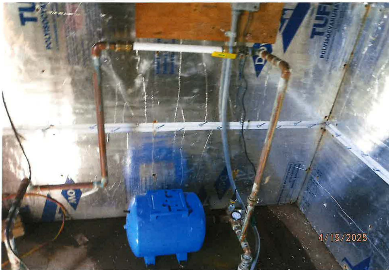
SMALL PRESSURE TANK AND MAIN DIVERTING PIPELINE
