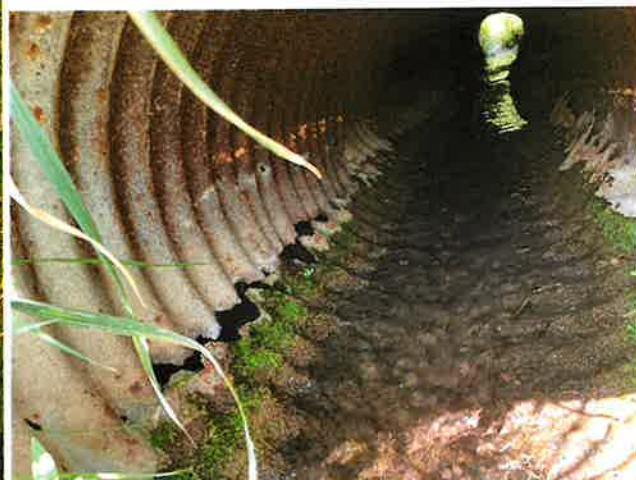
Figure 5 Interior of the culvert and large structural crack.
