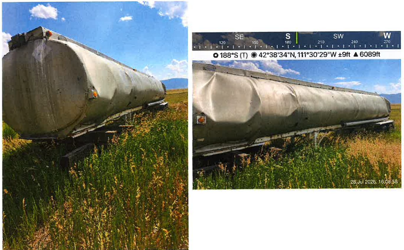
Figure 6 & 7.5 Storage tank for cistern. Not currently in use due to target practice evidence.
