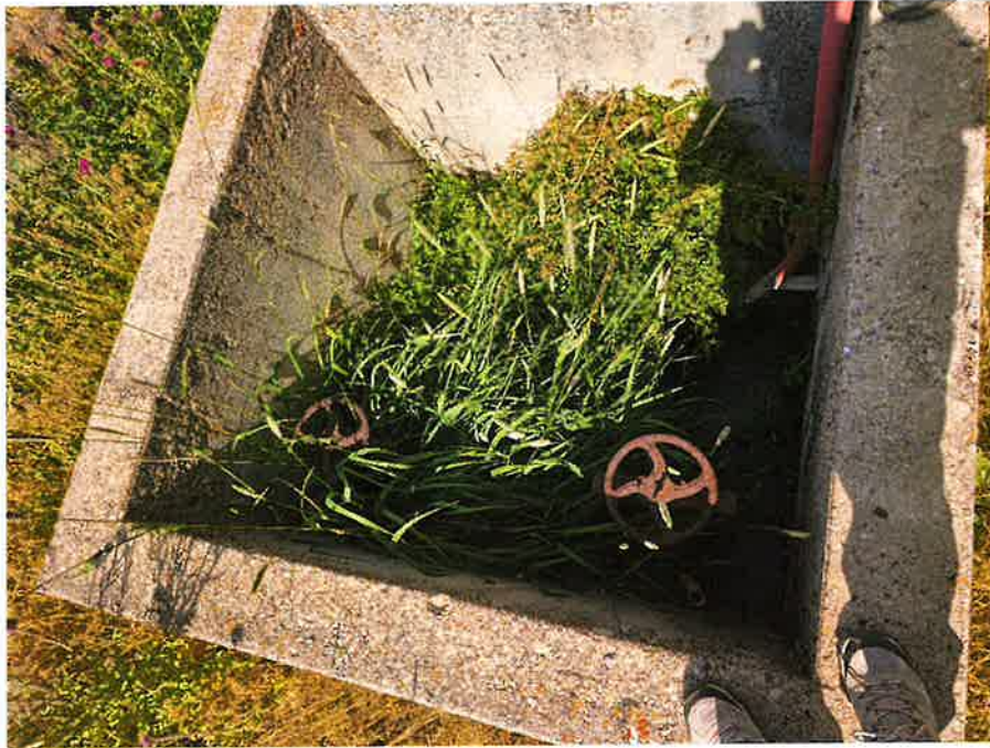
Figure 7 Cistern inner works includes two head gates and a PVC line that connects the storage tank to the cistern.
