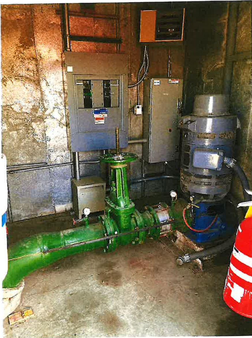
Well #10 100 HP pump
