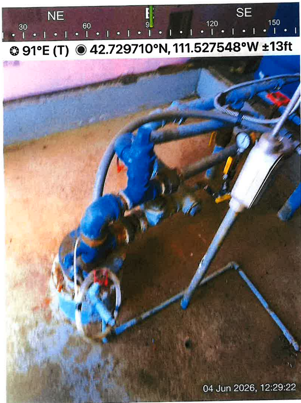
Well #11 domestic well
