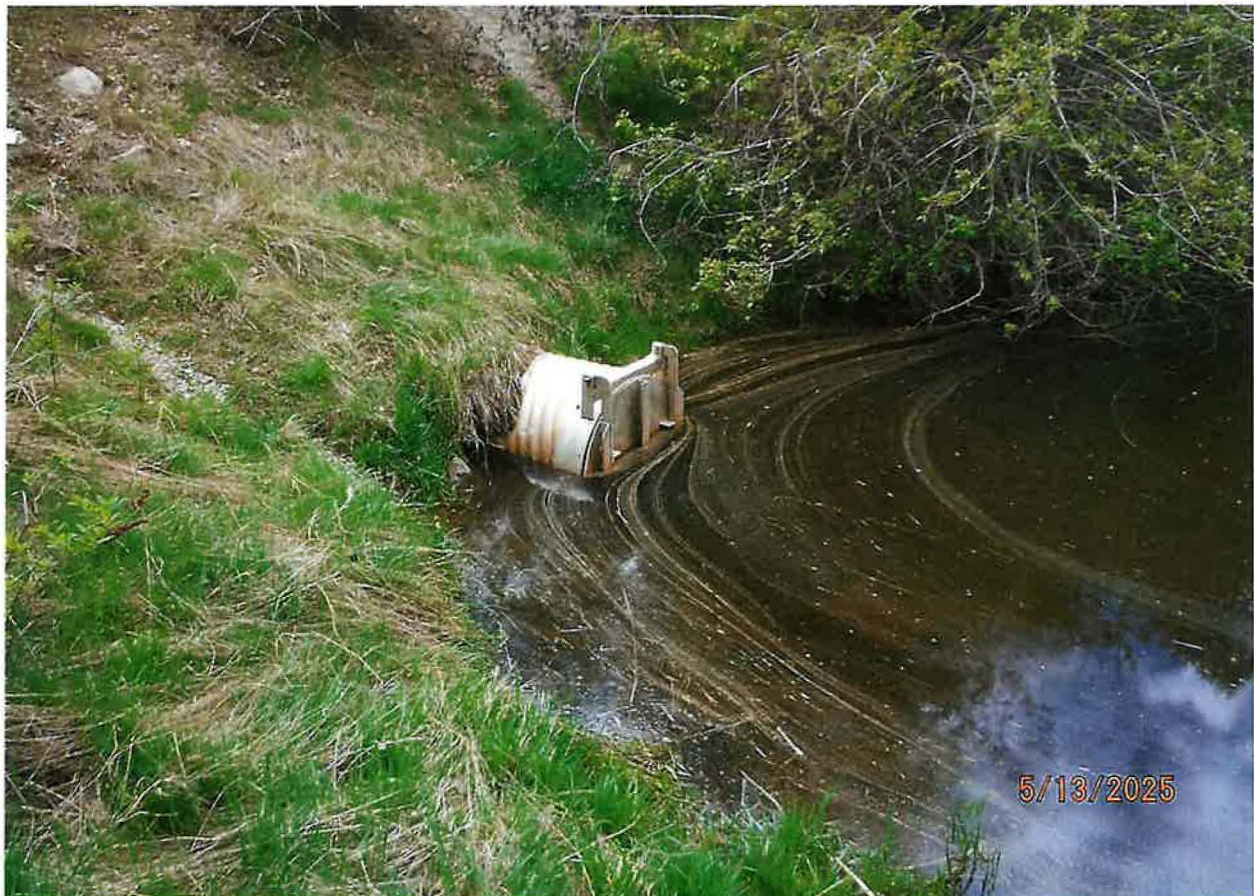
24-INCH OUTFLOW FROM SLOUGH TO RIVER. CUVLERT CLOSED TO MITIGATE BACKCHANNEL FLOW FROM RIVER
