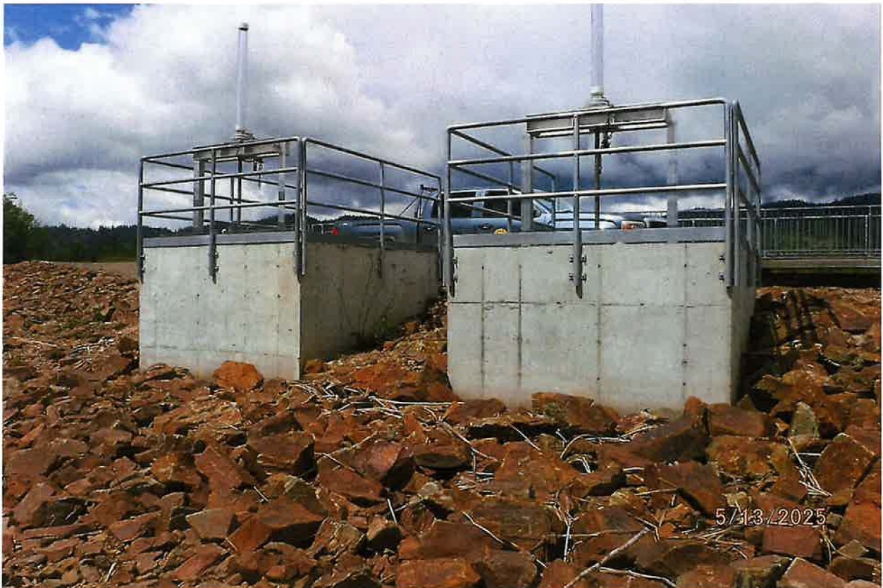
2 EA POD(s) – PRIMARY FLOW CONTROL STRUCTURES FOR BLACK ROCK SLOUGH ENHANCEMENT PROJECT
