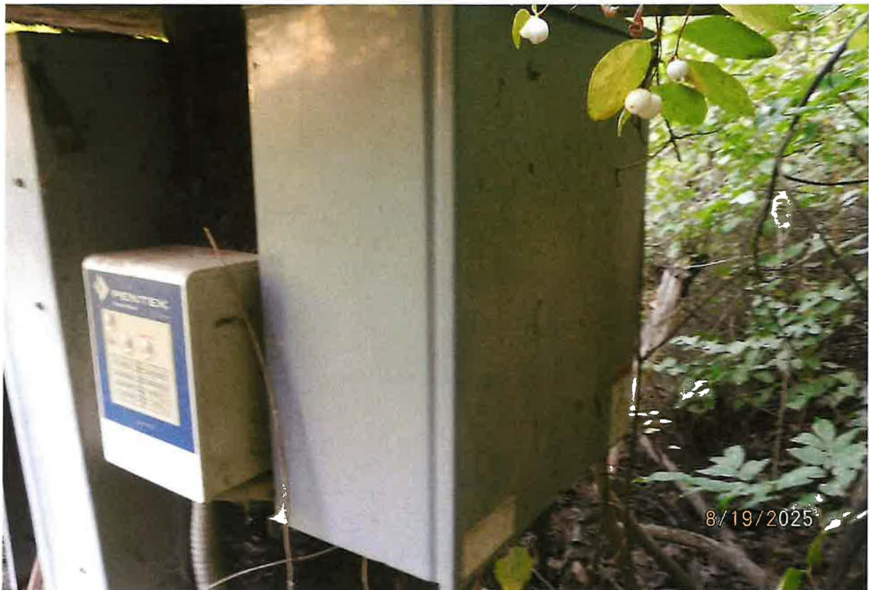
IRRIGATION FROM STORAGE CONVEYANCE SYSTEM – PENTEK/GOULDS MOTOR/PUMP FROM POND UP HILL TO IRRIGATION FROM STORAGE POU
