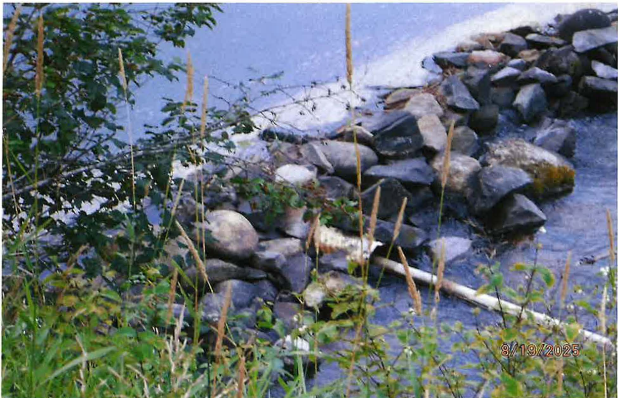
POD – 3-INCH PVC PIPELINE FROM COLLECTION POOL ROUTED DOWN STREAMBED, ACROSS ROADWAY, AND BY BURIED PIPELINE TO STORAGE POND
