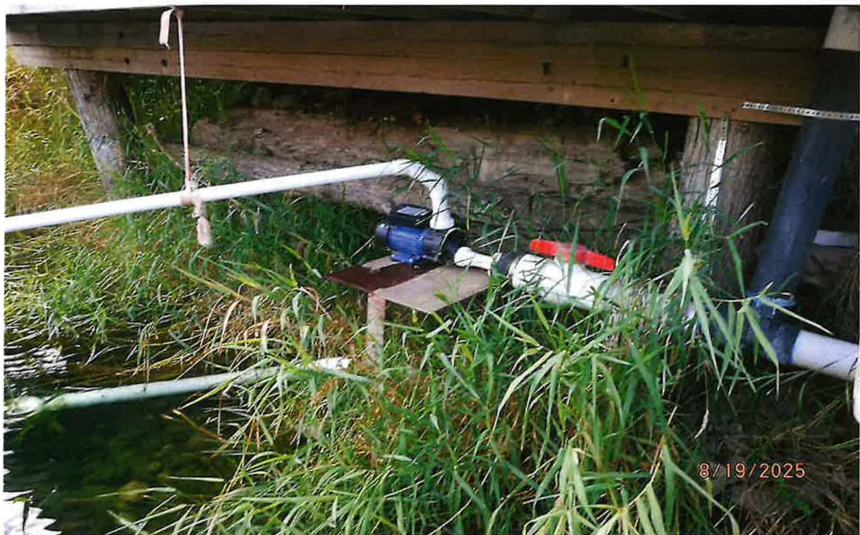
CONVEYANCE SYSTEM ENTERING STORAGE POND – AT THIS POINT GRAVITY FLOW IS ASSISTED BY A SMALL 0.8 HP CENTRIFUGAL PUMP TO STORAGE – DIVERSION TO STORAGE BENEFICIAL USE
