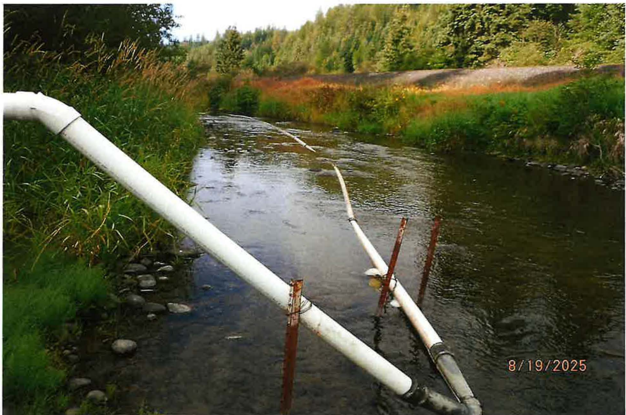
WATER CONVEYANCE SYSTEM – GRAVITY FLOW IN 3-INCH PVC PIPELIEN DOWN STREAM BED; PHOTO WHERE PIPLINE EXITS STREAM BED AND ROUTES BENEATH ROADWAY
