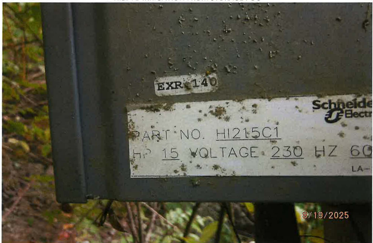
IRRIGATION FROM STORAGE CONVEYANCE SYSTEM – 15 HP SUBMERSIBLE PUMP/MOTOR FROM STORAGE POND TO POU FOR IRRIGATION
