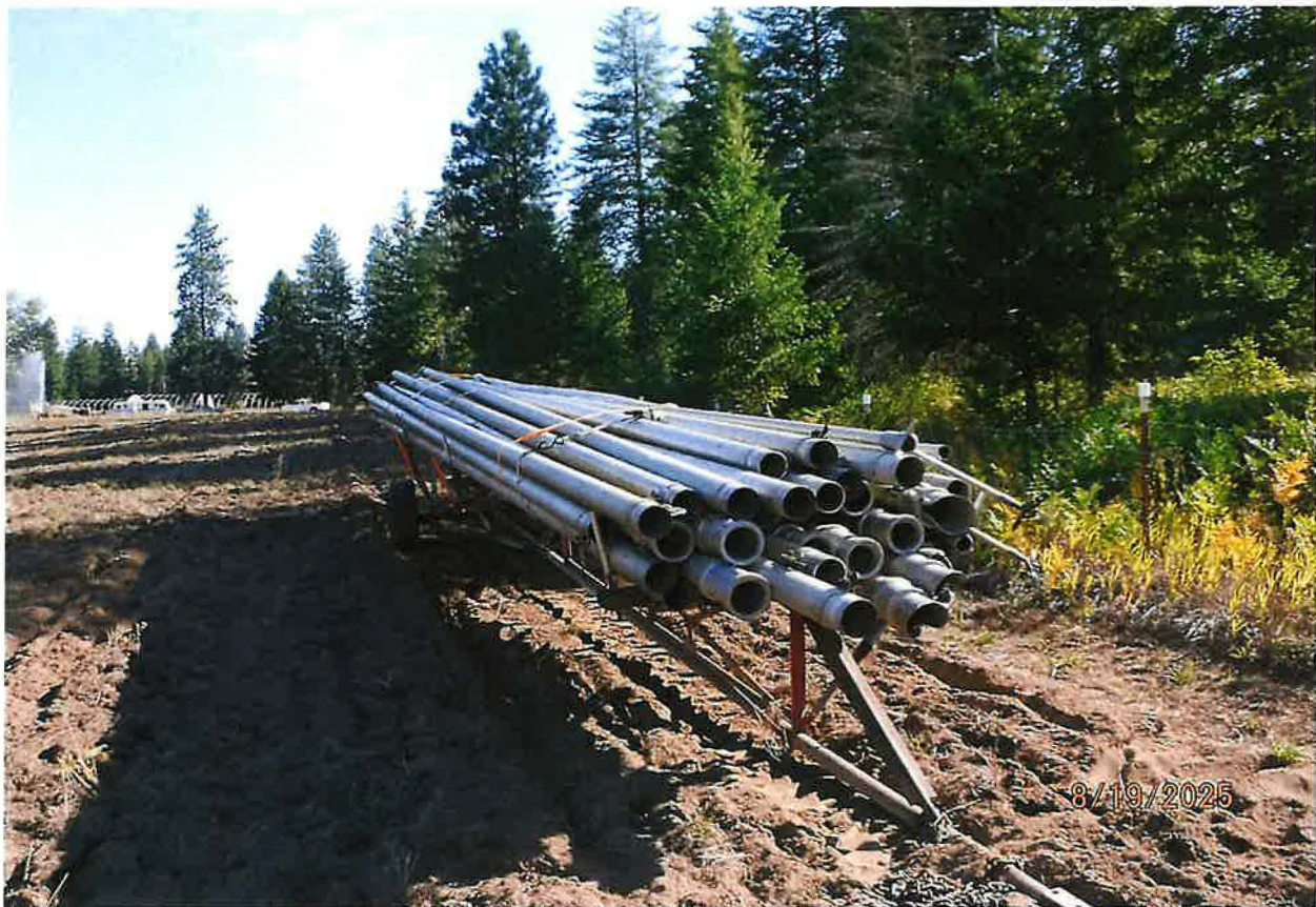
HAND LINE ON SITE FOR USE AS PART OF IRRIGATION FROM STORAGE POU
