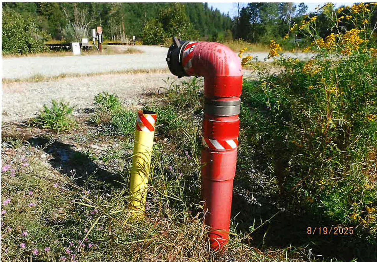
FIRE TRUCK FILL POINT FROM STORAGE POND LOCATED IN BETWEEN ROADWAY AND POND
