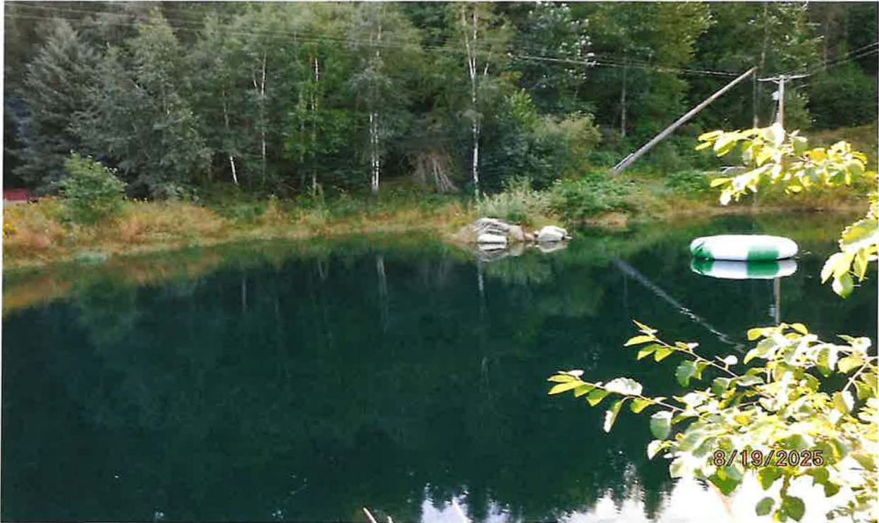
FIRE PROTECTION SUBMERGED PIPELINE TO TENDER TRUCK FILL POINT LOCATED ON NORTHWEST REACH OF STORAGE POND
