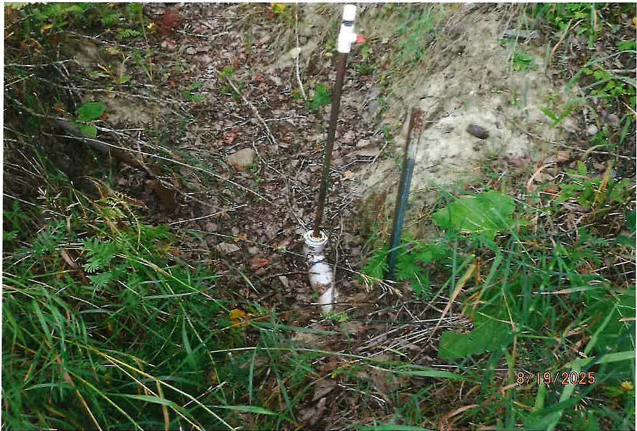
CONVEYANCE PIPELIEN ON EAST SIDE OF ROAD WITH BLOW-OUT VALVE. PIPELINE RUNS TO GROUND UP TO STORAGE POND
