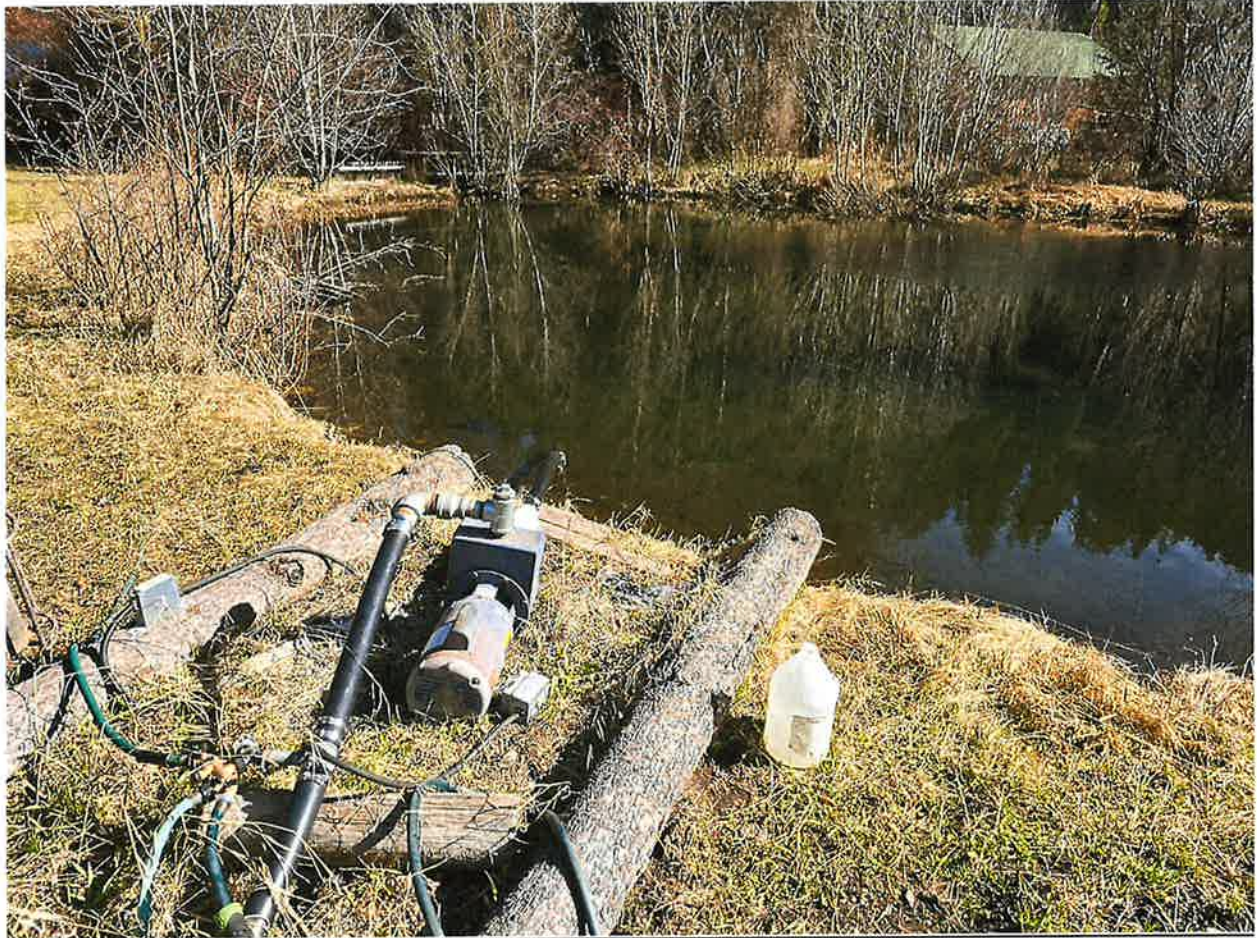
Irrigation pump pumping from the recreation pond.
