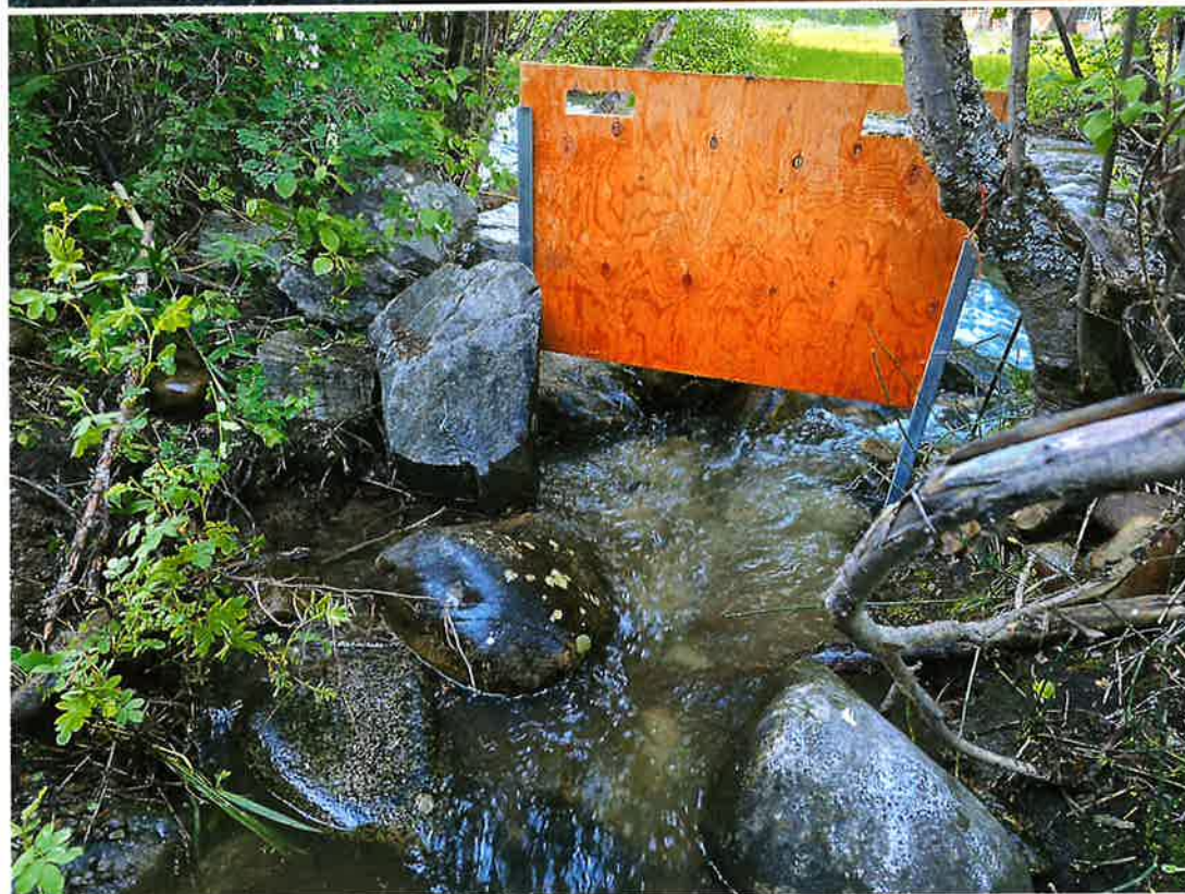
Permit 75-7601 lockable controlling works on NF Salmon River, 6/12/2026
