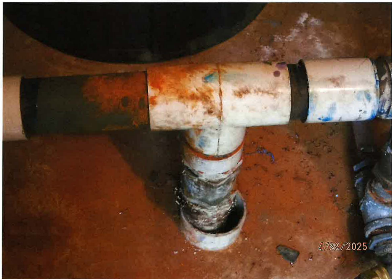
MAIN SERVICE PIPELINE (VERTICAL OUT OF PUMP STATION) RECEIVING FROM 3EA PRESSURE TANKS (HORIZONTAL PIPING)
