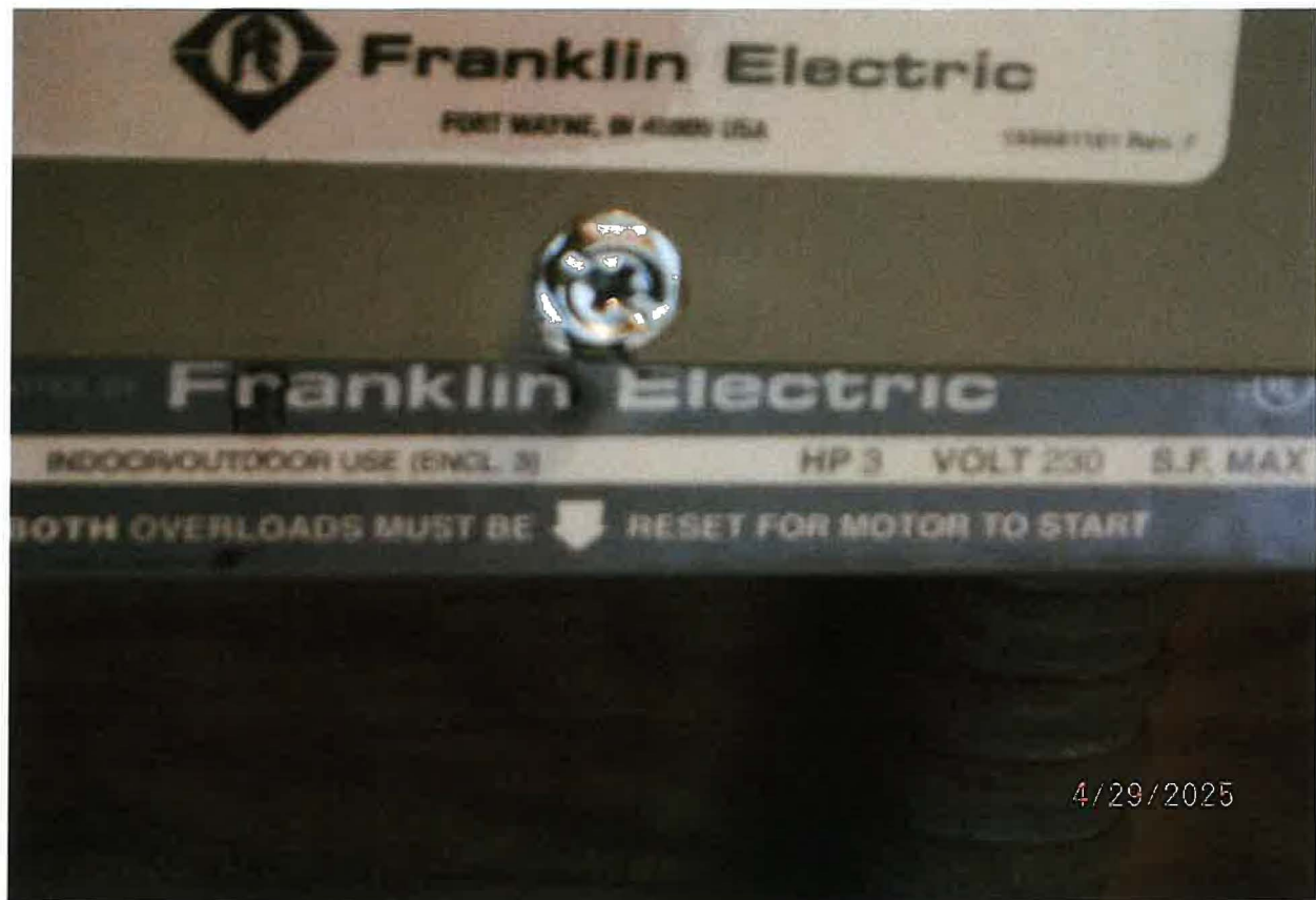
PUMP MOTOR 3 HP WITH 1 INCH MAIN SERVICE PIPELINE
