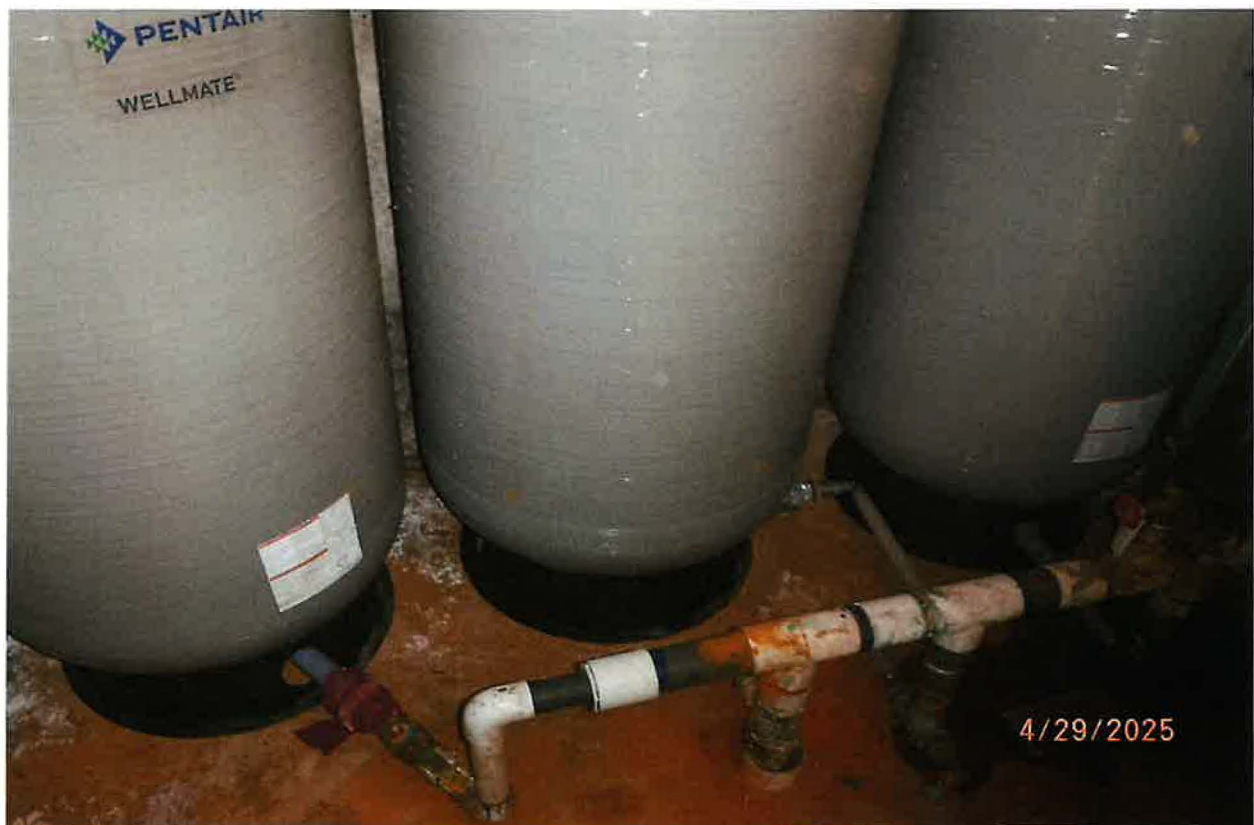
CONVEYANCE SYSTEM INCORPORATES 3EA PRESSURE TANKS WITH NO STORAGE COMPONENT TO WATER SYSTEM
