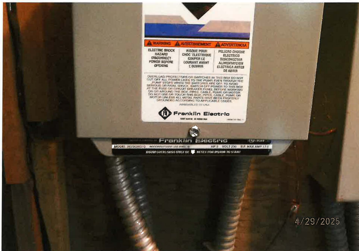
POD – 3 HP SUBMERSIBLE PUMP WITH FRANKLIN ELECTRIC 3 HP PUMP MOTOR
