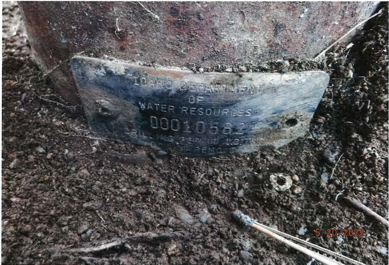
POD – GROUND WATER WELL D-TAD D0010582
