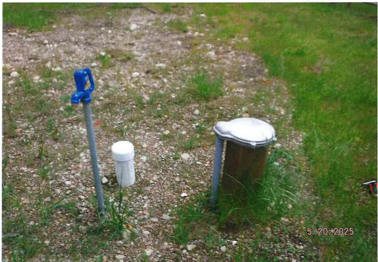
POD – 8-INCH CASED GROUND WATER WELL PERMIT NO. 96-95-N-30 CO-LOCATED FROST-FREE HYDRANT (USED FOR FLOW MEASUREMENTS)
