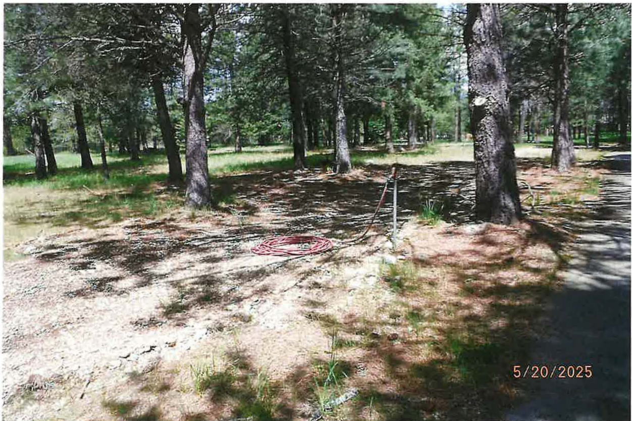
EXAMPLE – 1-OF-7 FROST-FREE HYDRANTS USED TO FACILITATE IRRIGATION BY HOSE AND SPRINKLERS
