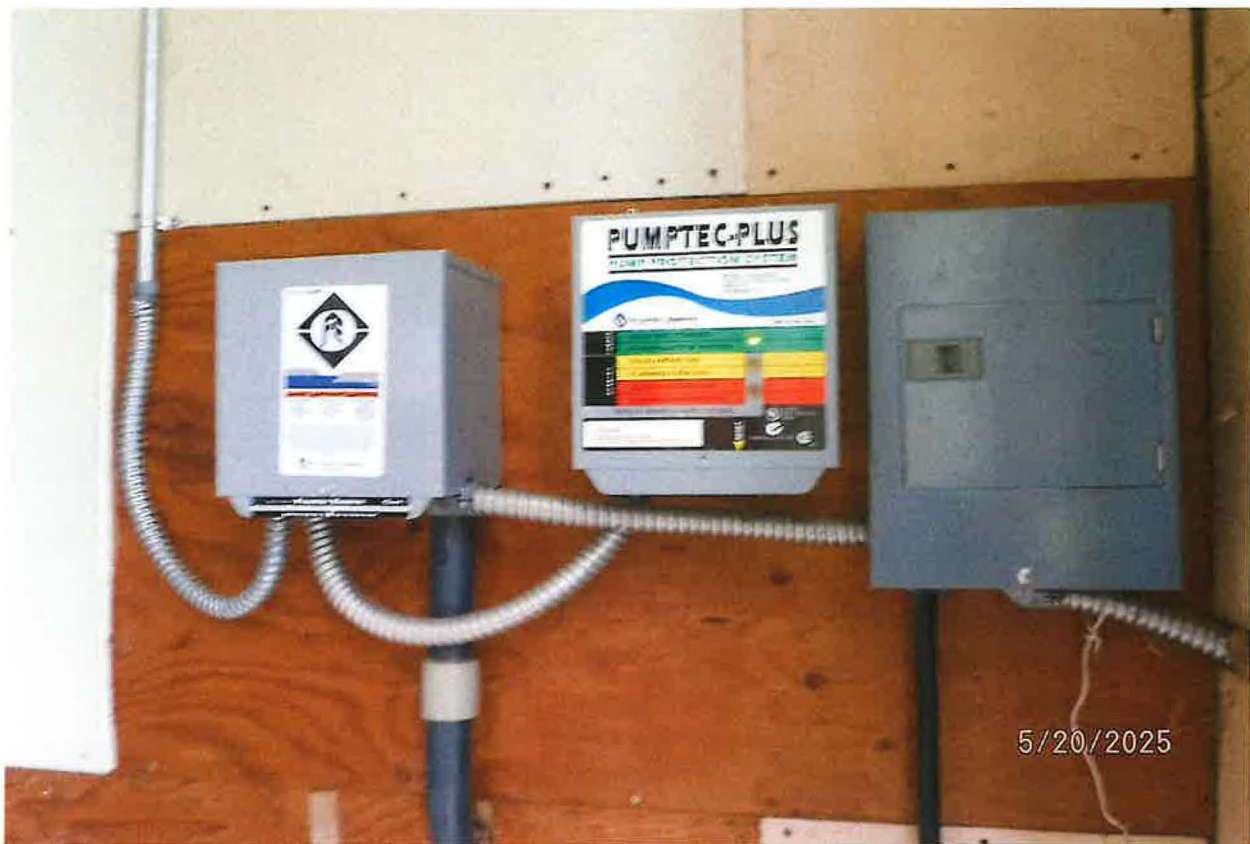
DIVERTING WORKS – WELL PUMP MOTOR CONTROL PANEL (LOCATED INSIDE SHOP NORTH OF WELL ACROSS PASTURE)
