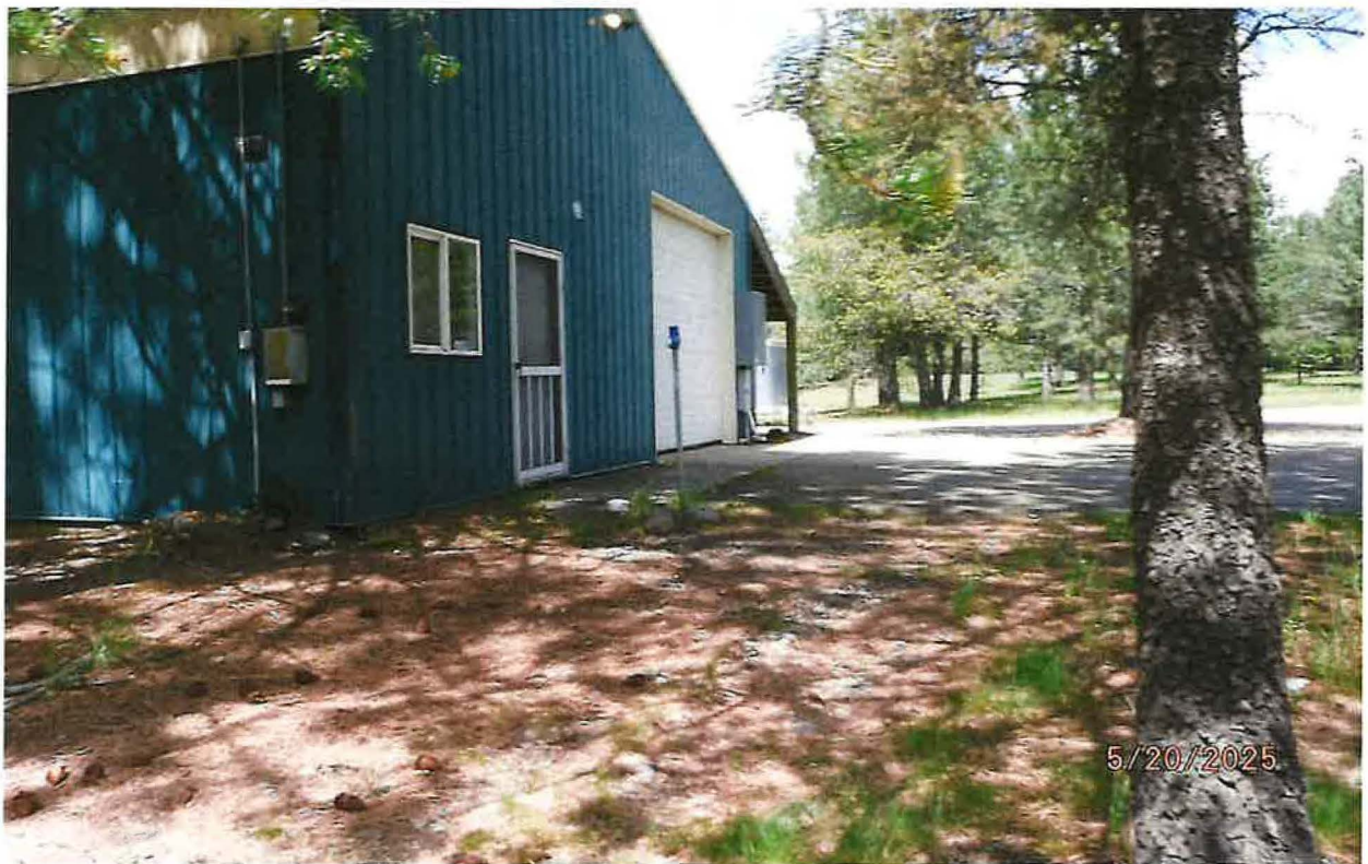
EXAMPLE – 1-OF-7 FROST-FREE HYDRANTS USED FOR IRRIGATION; 400 FT OF HOSE AND RAINBIRD TRIPOD SPRINKLERS USED TO IRRIGATE LAWN, PASTURE, AND LANDSCAPING
