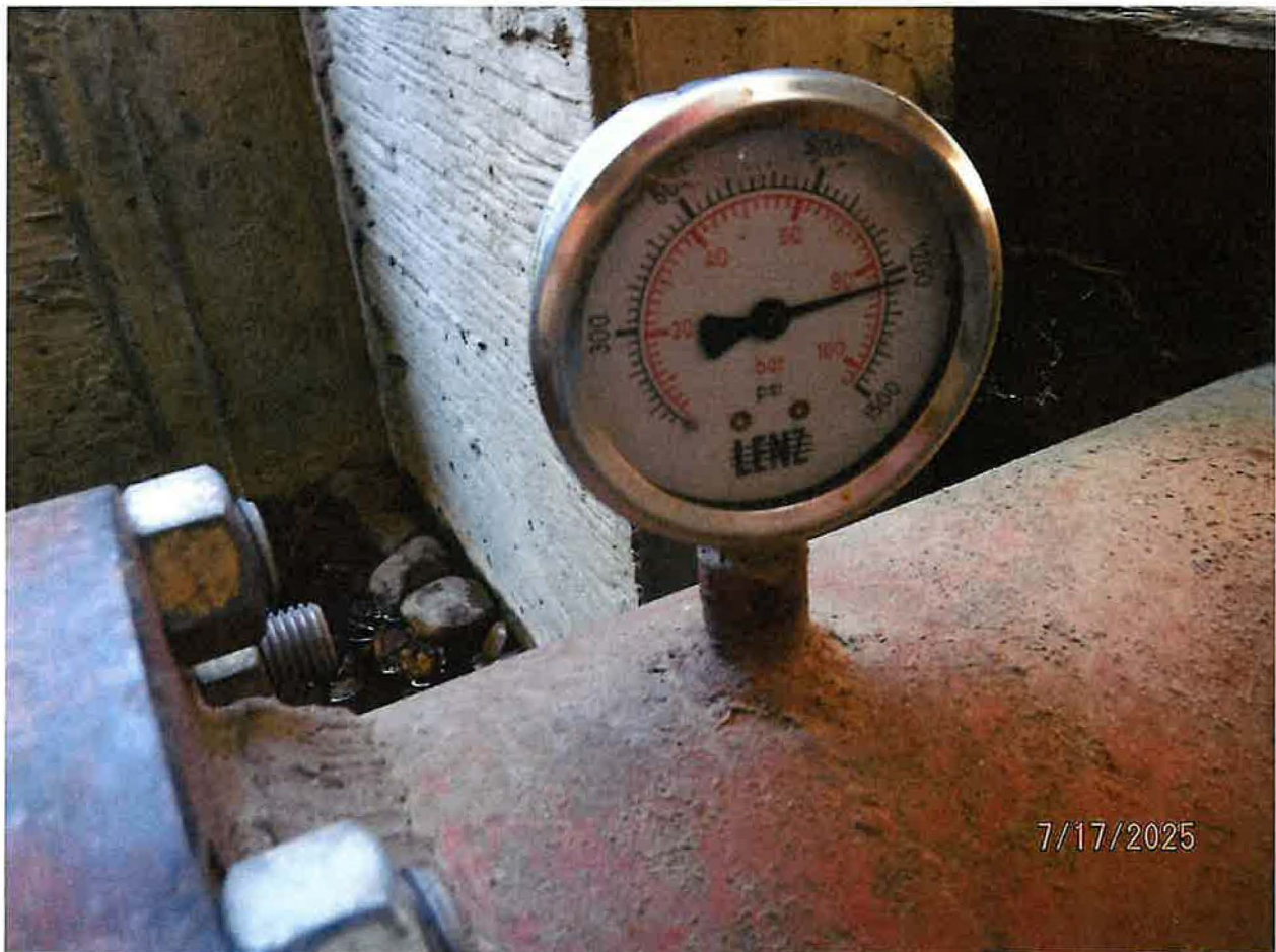
1225 PSI GAUGE PRESSURE WITH PUMP CYCLED ON
