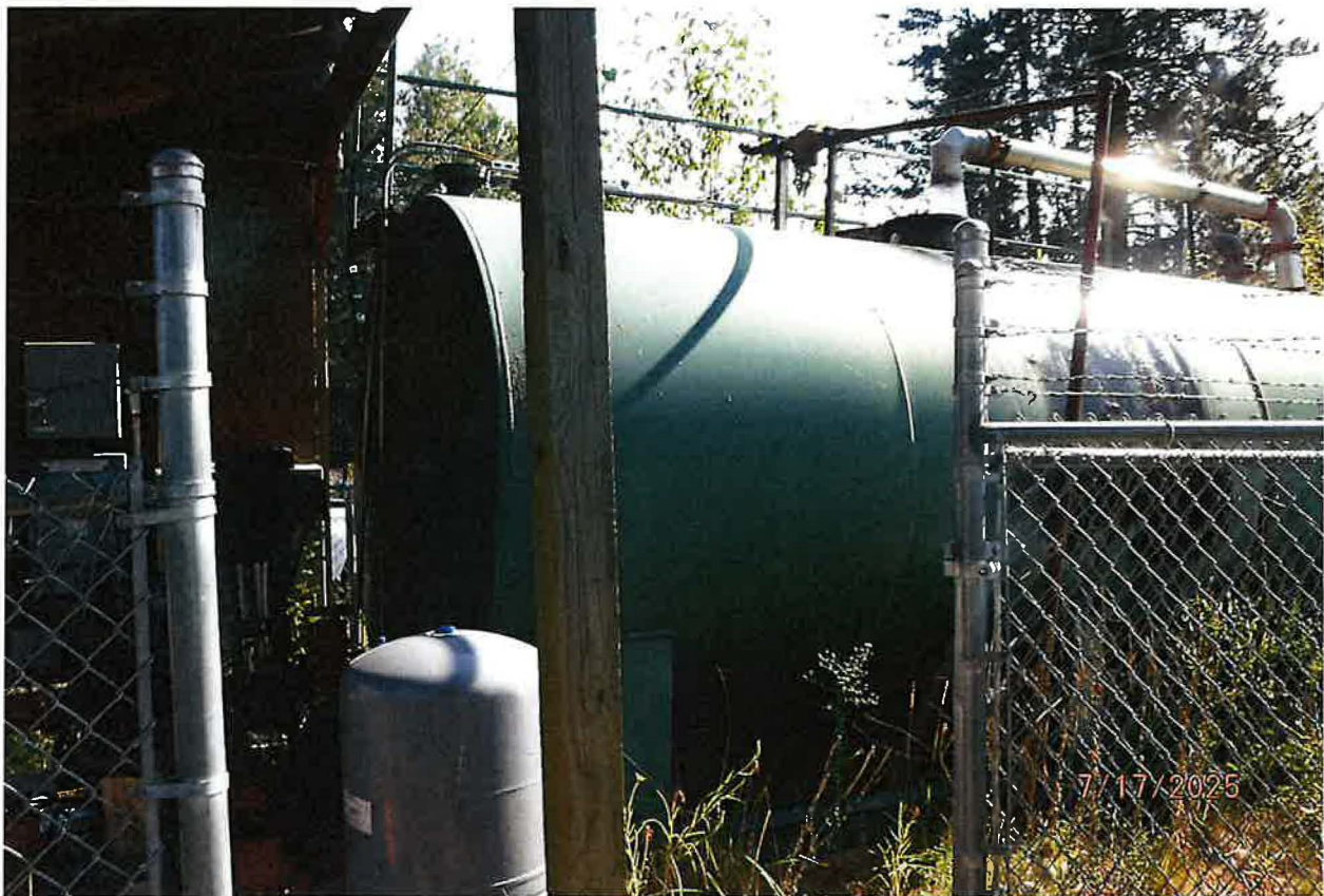
WATER CONVEYANCE SYSTEM – 6-INCH PIPELINE FROM POD FILLS 6,500-GAL STORAGE RESERVOIR PRIOR TO DISTRIBUTION BY THREE TRANSFER PUMPS
