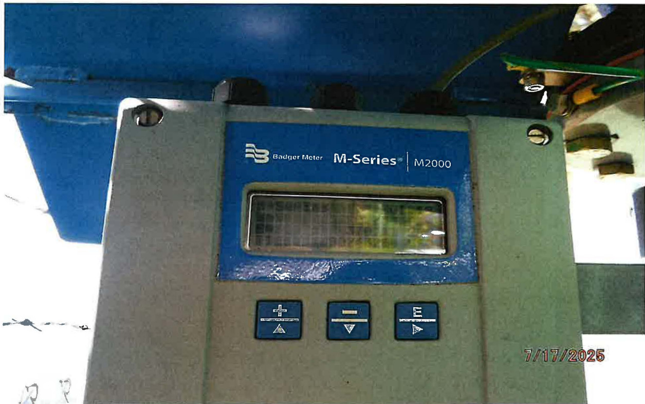
FLOW METER CONTROL PANEL – INDICATED 370-380 GPM DURING ACTIVE PUMPING
