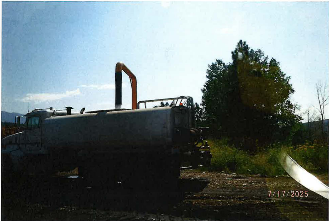
INDUSTRIAL / FIRE PROTECTION POU – J-HOOK WATER TRUCK FILL POINT
