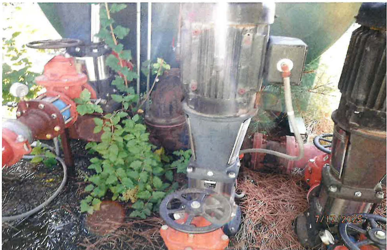
3EA – 25 HP BALDER PUMPS USED TO DISTRIBUTE WATER TO POU VIA THREE LOG DECK 6-INCH PIPELINES WITH 1-INCH SPRINKLER LATERAL POLYPIPE RUNS AT INERVAL & A WATER TRUCK J-HOOK FILL POINT
