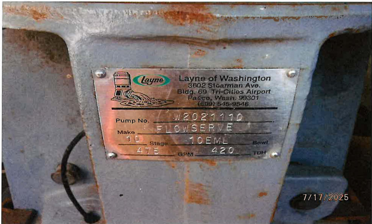
DATA PLATE ON MOTOR INDICATES 475 GPM PUMP CAPACITY
