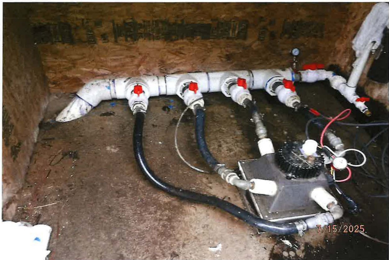
POU – MICRO POWER STATION; INFLOW FROM PENSTOCK ON L/H WITH 4EA NOZZLE STEM PIPES ATTACHED TO POWER UNIT
