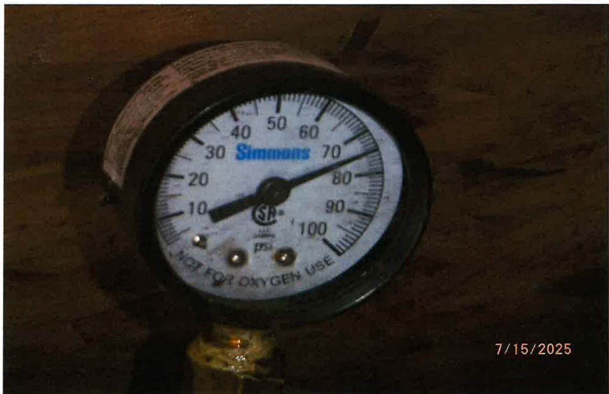
POU – POWER SYSTEM OPERATING AT 75 PSI AT TIME OF EXAM
