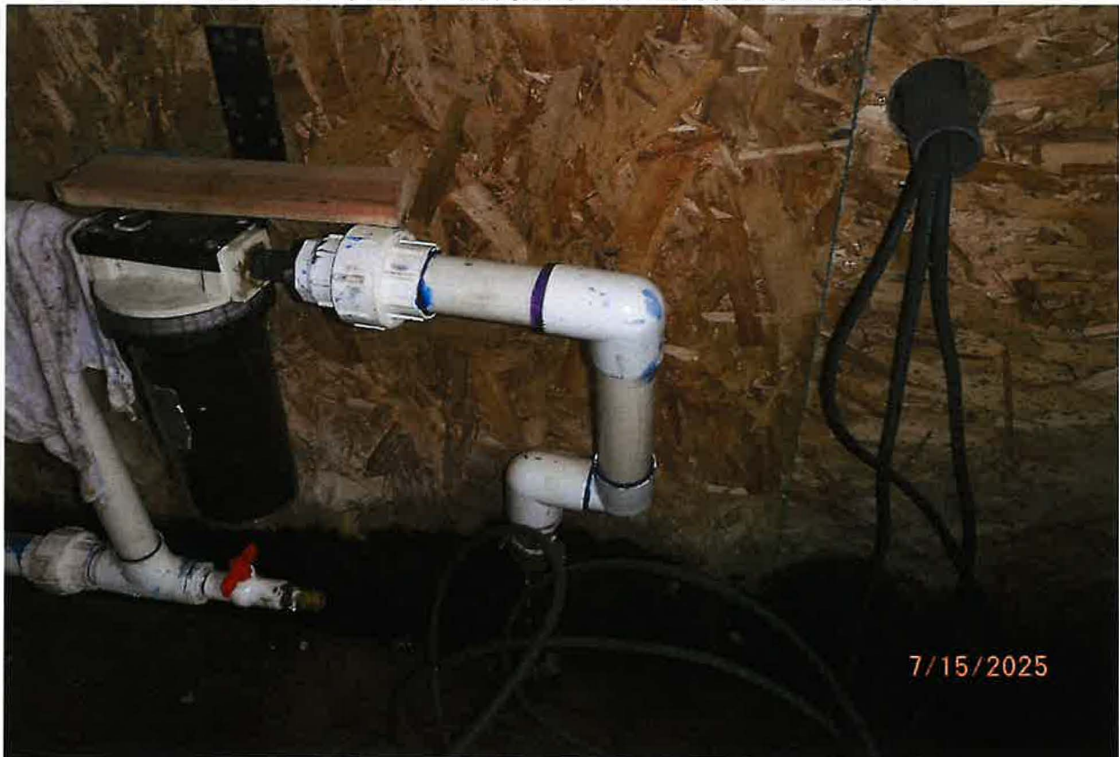
OUTFLOW FROM IRRIGATION SERVICE PIPE VAVLE ROUTES OUT OF POWER STATION TO MULTIPLE FROST-FREE HYDRANTS
