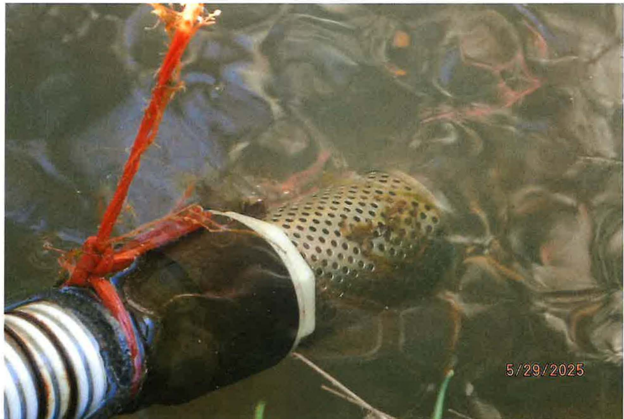
POD – FLEXIBLE 1.5-INCH INTAKE SUCTION PIPE WITH 3/32-INCH SCREEN IN CREEK
