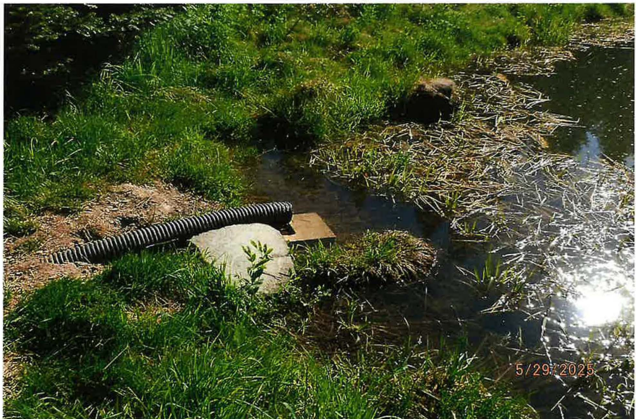
POND OVERFLOW DEVICE IS A 4-INCH CORRUGATED FLEX PIPE; WATER IS DIVERTED FROM THE CREEK UNTIL POND WATER IS OVERFLOWING THE DISCHARGE PIPE THEN THE PUMP IS TURNED OFF
