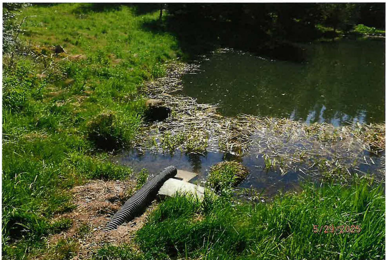
OVERFLOW DISCHARGE PIPE LOCATED IN NW CORNER OF POND
