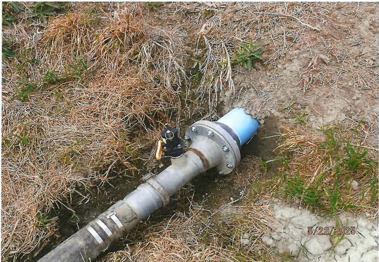
CONVEYANCE SYSTEM – 8-INCH ALUMINUM ROUTED ACROSS FIELD BURIED PIPELINE TO CENTER PIVOT
