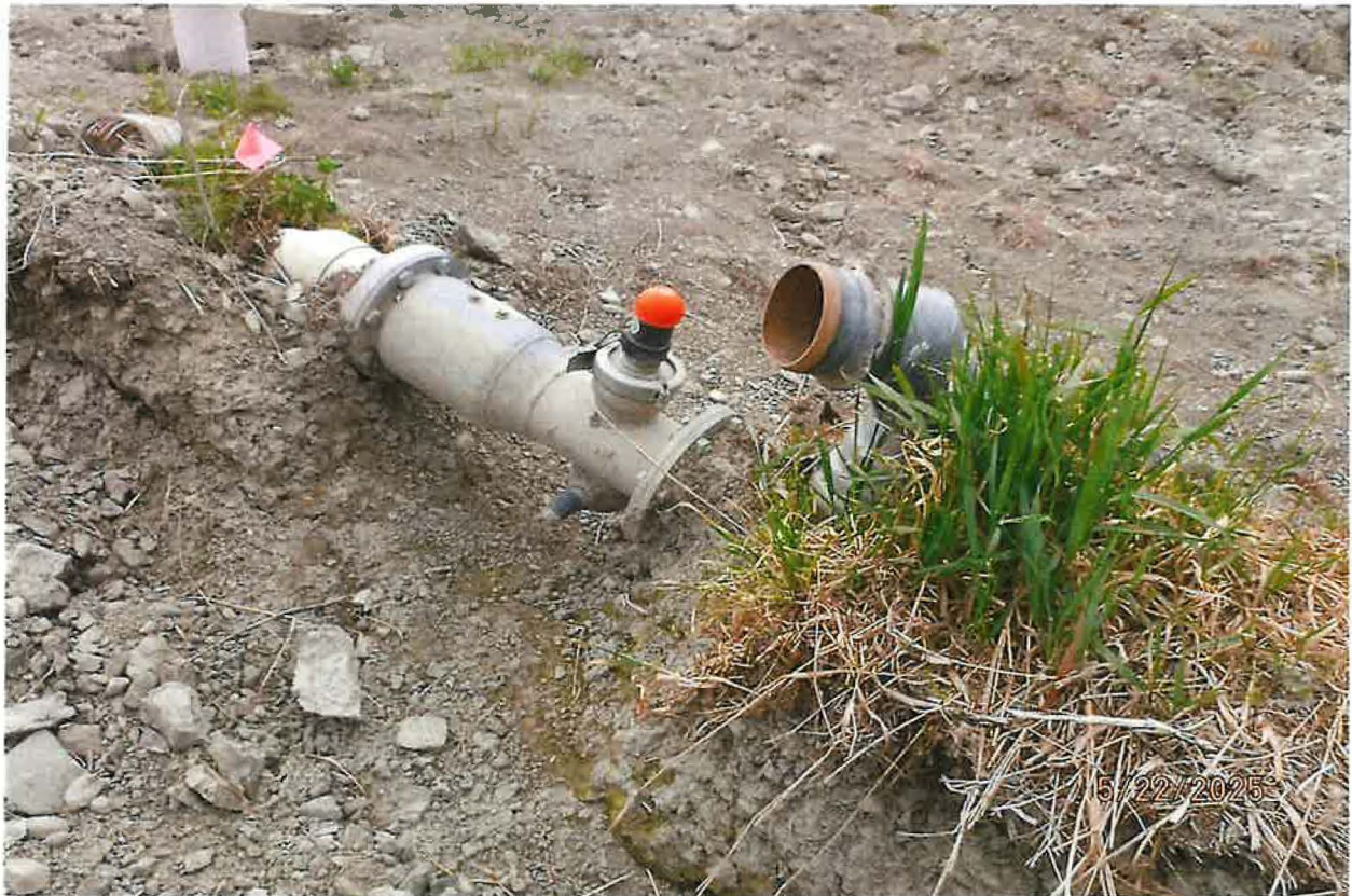
CONVEYANCE SYSTEM – 8-INCH ALUMINUM ROUTED EAST TO MAIN IRRIGATION RISER FOR WHEELED MARCHING PIVOT
