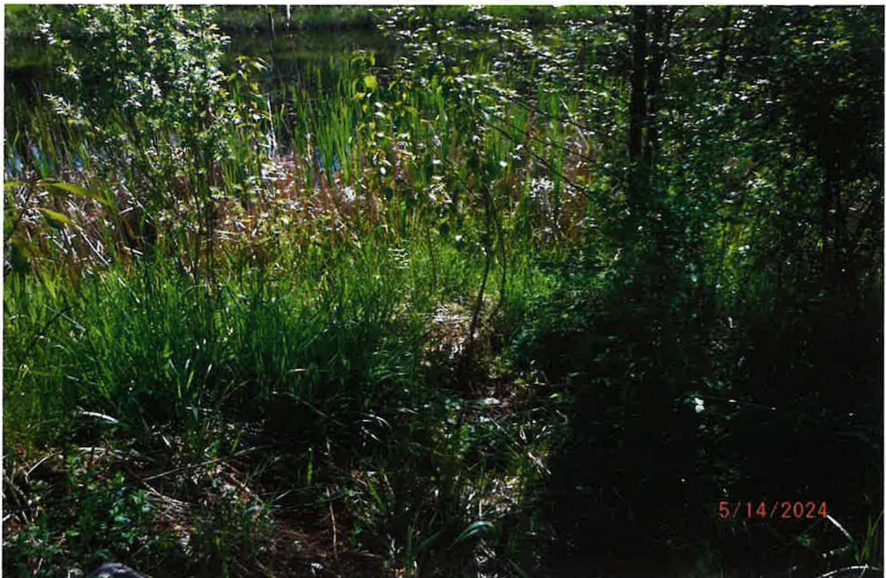
SURFACE RUNOFF INFLOW PIPE SET HIGH IN ELEVATION ON POND BANK, WELL ABOVE THE NORMAL 4-FT POND DEPTH MAINTAINED BY CONSTRUCTION DESIGN.
