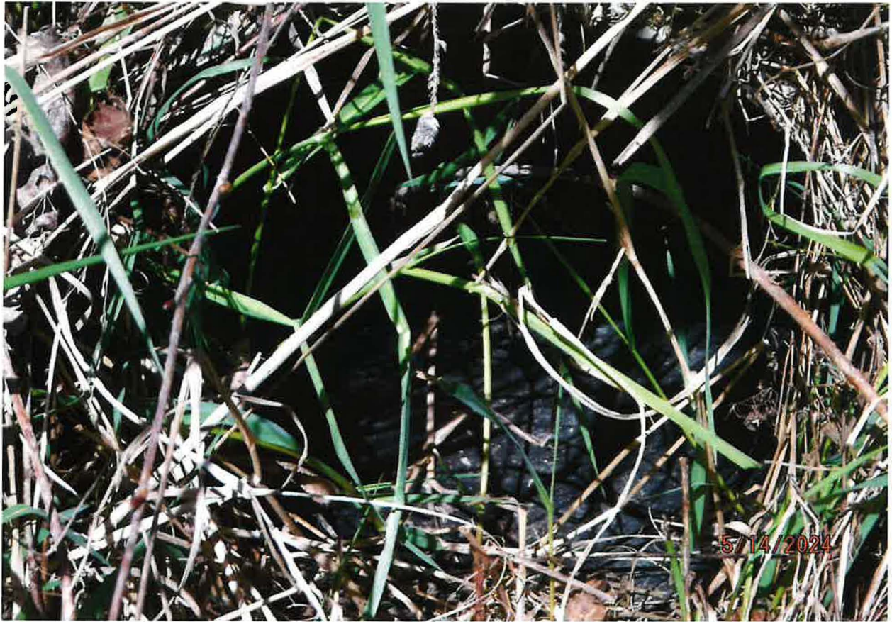
SINGLE 10-INCH CORRUGATED POLY PIPE LOCATED ON WESTERN BANK OF STORAGE POND. ALLOWS INFLOW OF SURFACE RUNOFF DURING SEASONAL RUNOFF EVENTS TO ENTER STORAGE POND.
