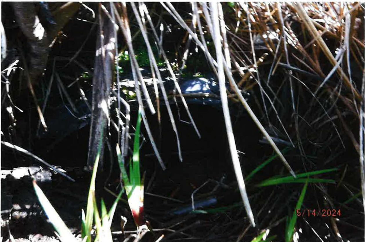
SINGLE 10 INCH BLACK CORRUGATED POLY PIPE ALLOWS SURFACE RUNOFF WATER TO ENTER POND FROM THE WESTERN BANK DURING SEASONAL RUNOFF EVENTS
