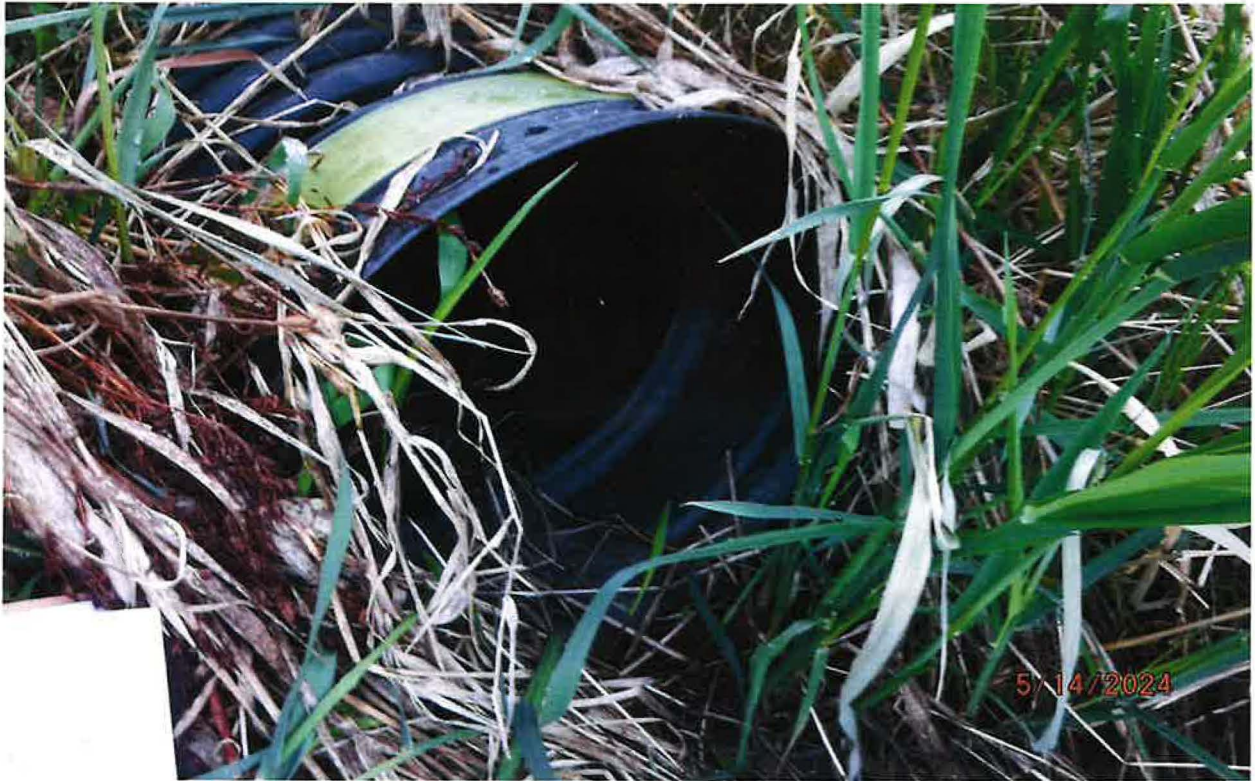
ONE OF TWO OVERFLOW DISCHARGE PIPES - 10 INCH CORRUGATED POLY PIPE SET IN ELEVATION TO MAINTAIN A 4-FT POND DEPTH AT ALL TIMES OF YEAR TO MAINTAIN ICE SKATING FREEZE DEPTH IN WINTER. OVERFLOW DISCHARGE FLOWS OUT OF THE SOUTHEAST CORNER OF POND.
