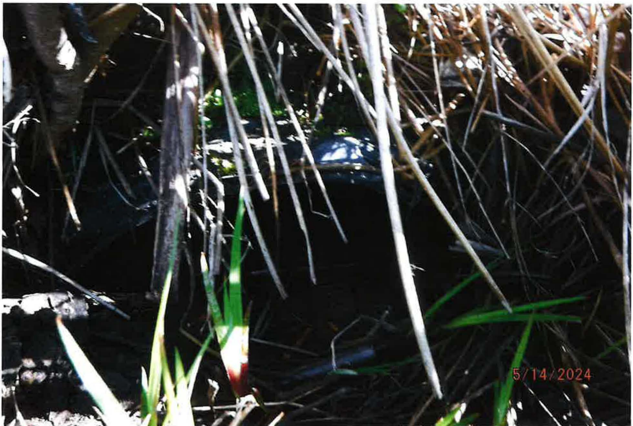
SECONDARY OVERFLOW DISCHARGE PIPE SET TO SAME ELEVATION AS FIRST; LOCATED AT THE NORTHEASTERN CORNER OF THE STORAGE POND.
