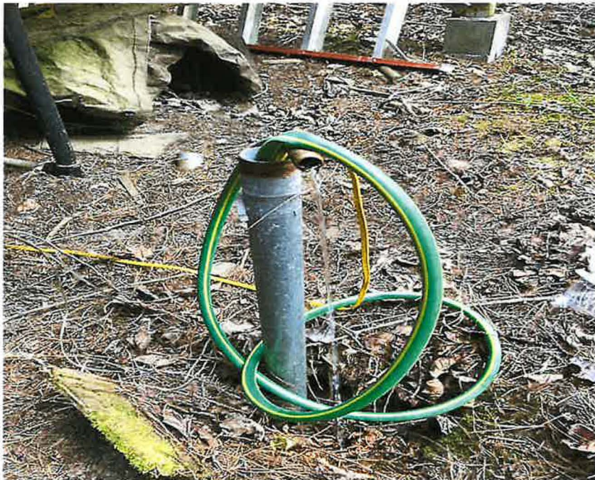
POD – HAMMERED SAND POINT WELL WITH SMALL ELECTRIC PUMP TO HOSE TO DOMESTIC USE – IMAGE PROVIDED BY PERMIT HOLDER (EMAIL) ON 7/28/2025
