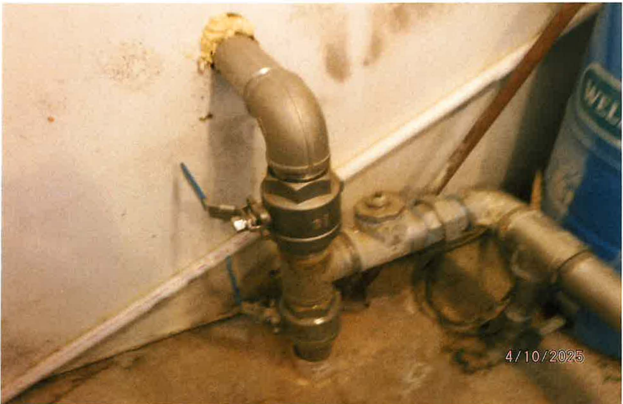
CONVEYANCE SYSTEM – 2-INCH MAIN PIPELINE ROUTING DOWN TO FLOOR OF PUMP STATION WITH EXTERIOR MANUAL SHUT OFF VALVE. MANUAL SHUTOFF BLOW-OUT VALVE ROUTING UP AND THROUGH WALL OF PUMP STATION
