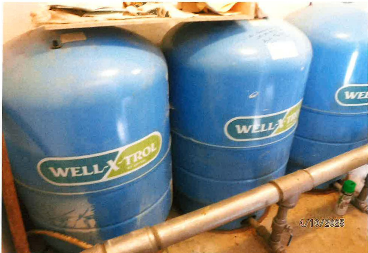
WATER CONVEYANCE SYSTEM INCLUDES 6EA PRESSURE TANKS REGULATED AT 25-28 PSI
