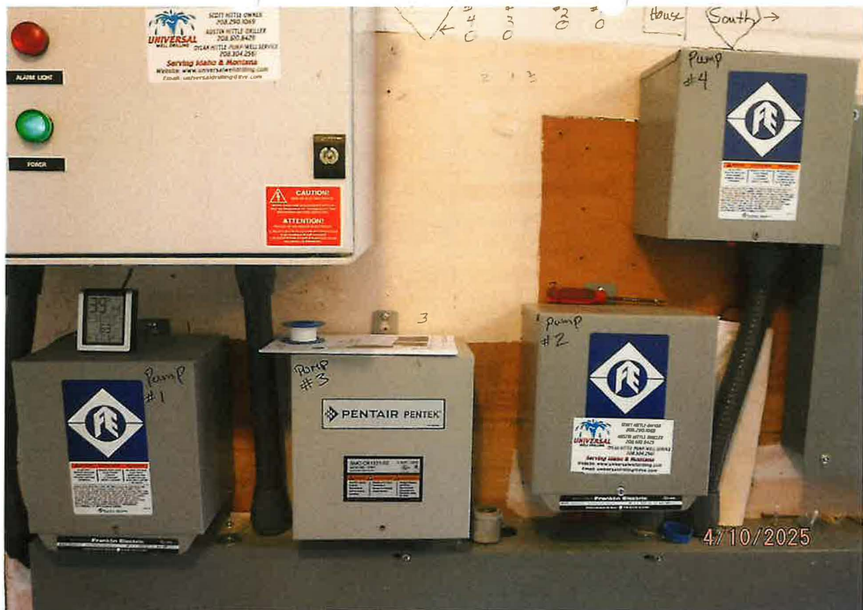
DIVERTING WORKS – 3EA FRANKLIN & 1EA PENTEK 1.5 HP PUMP MOTORS LABELED BY WELL #
