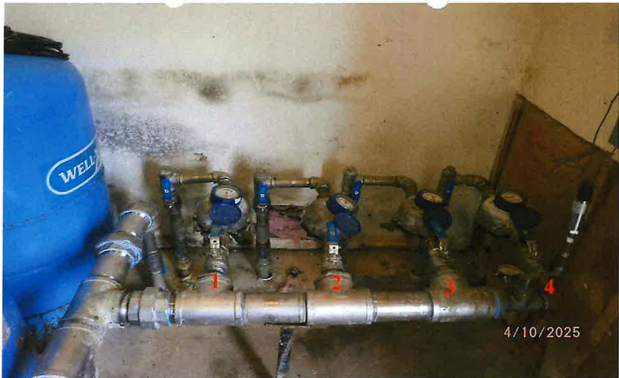
DIVERTING WORKS – EACH WELL HAS AN IN-LINE 1-INCH FLANGED HERSEY FLOWMETER INSTALLED WHERE THE MAIN SERVICE PIPE FROM WELL ENTERS PUMP STATION (PRIOR TO PRESSURE TANK & DISTRIBUTION PIPELINE)
