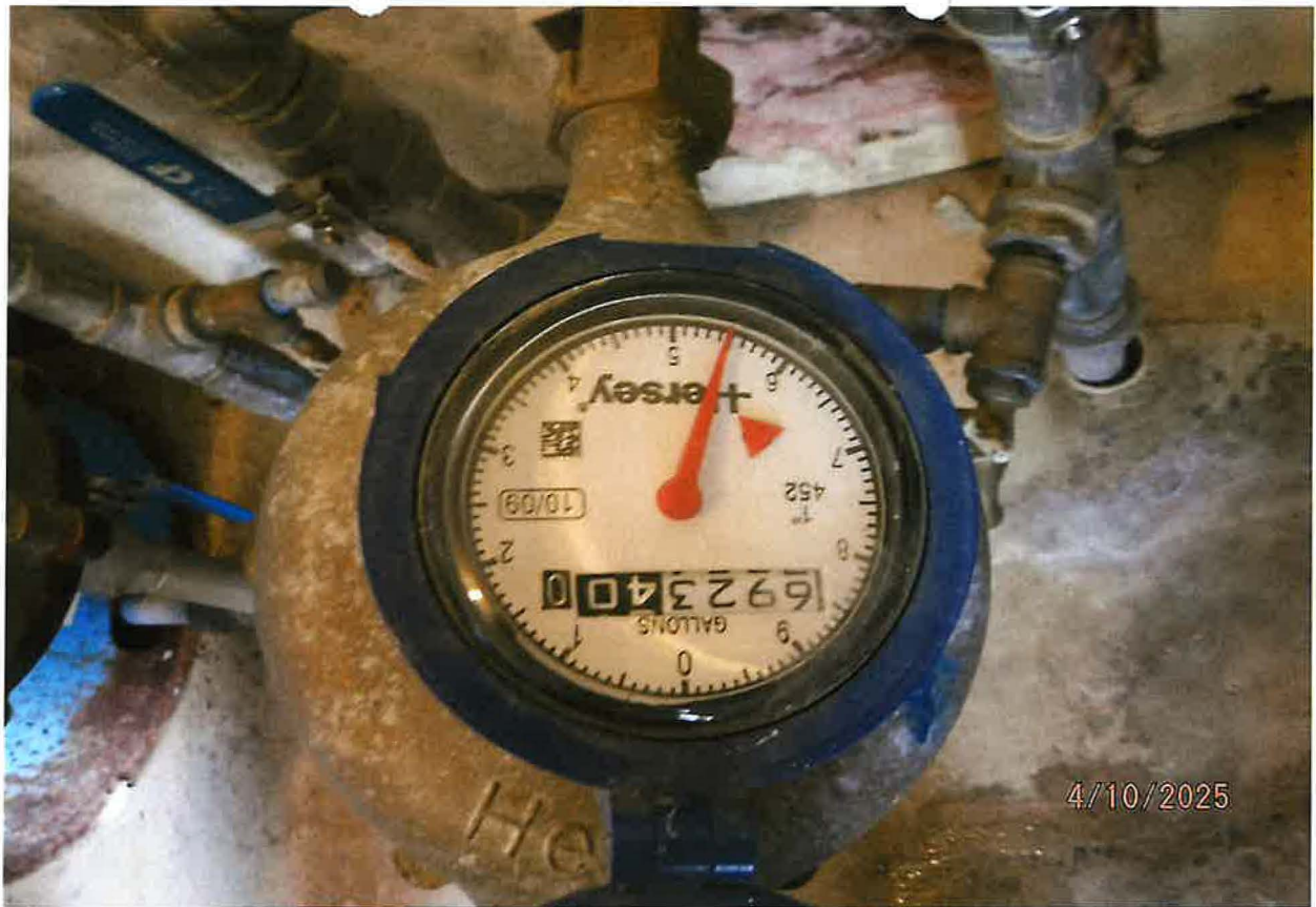
HERSEY FLOWMETER WELL #2
