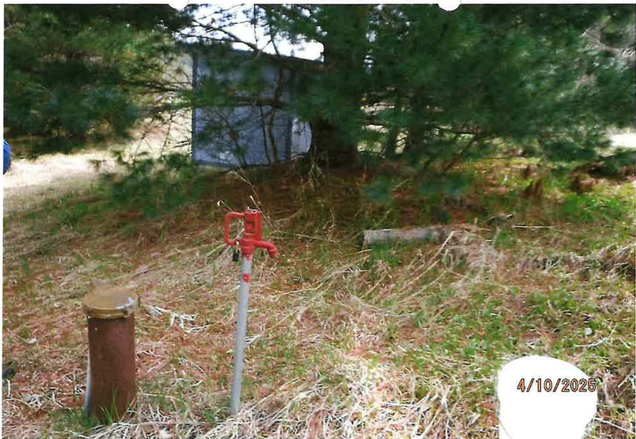
POD - PUMP STATION (BACKGROUND) & WELL #1 – 96-94-N-0204-000
