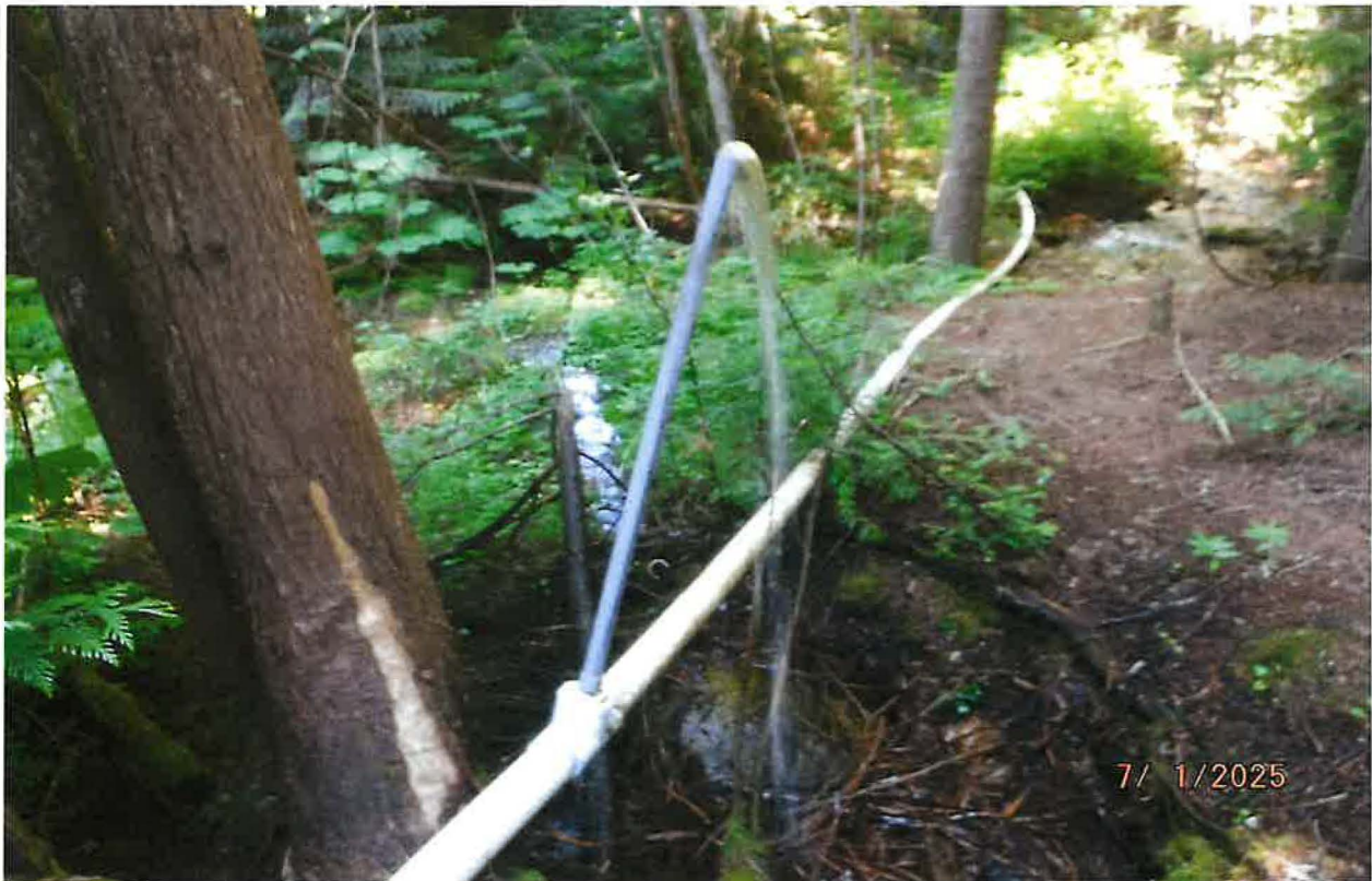
POWER SYSTEM PENSTOCK/CONVEYANCE CONSISTS OF 780-FT OF 3-INCH PVC; VENT/PRIMING PIPE LOCATED NEAR POD RETURNS FLOW TO STREAM
