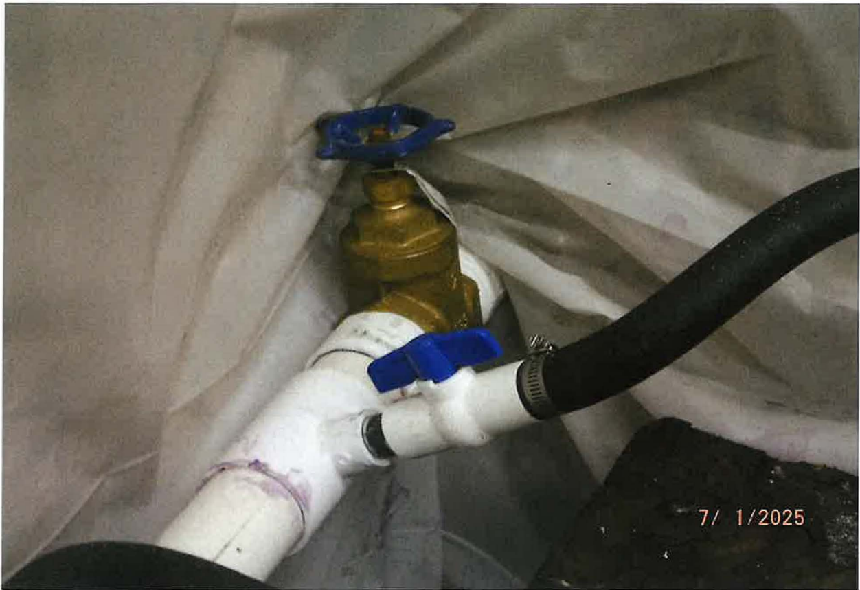
FIRE PROTECTION – MAIN 3-INCH PVC PIPELINE AT END OF POWER NOZZLE TEE(S); NOZZLES CAN BE CYCLED OFF TO ALLOW FULL PIPELINE FLOW THROUGH BALL VALVE (BLUE BRASS VALVE IN PHOTO) EXITING REAR OF POWER STATION
