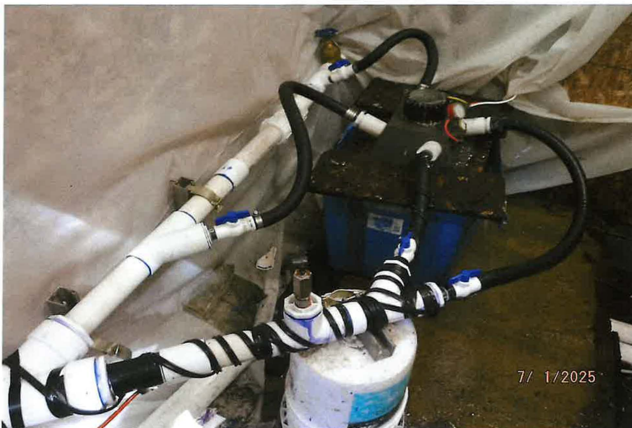
OVERFLOW FROM HYDRO POWER UNIT COLLECTS IN BLUE BIN WHERE IT'S PIPED AS OVERFLOW DISCHARGE BACK TO FLUME CREEK
