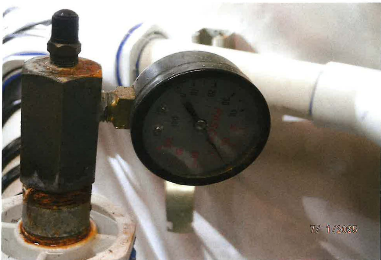
WATER SYSTEM PRESSURE GAUGE IDENTIFIES 65 PSI (PERMIT HOLDER ASSERTS THE GAUGE MAY BE MALFUNCTIONING AS THE SYSTEM NORMALLY OPERATES AT 50 PSI)
