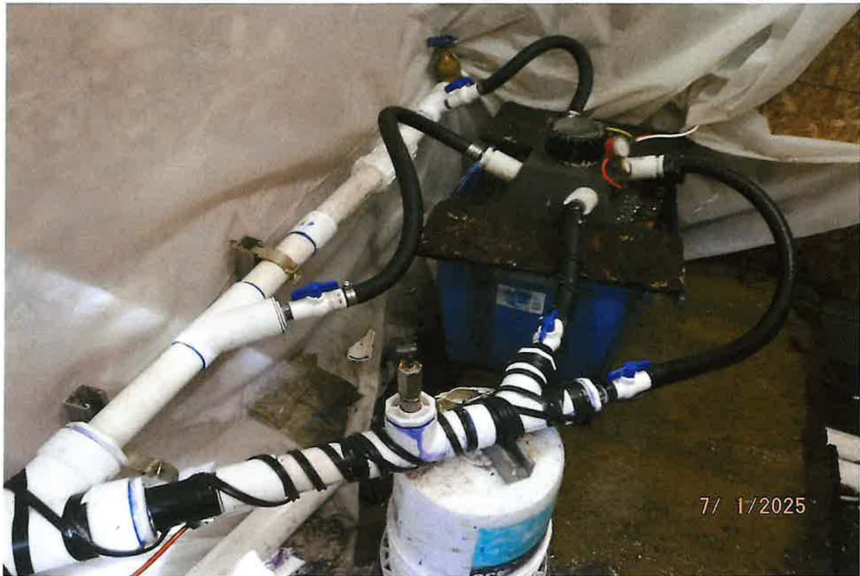
POWER POU – HARRIS LV800 MICRO-HYDRO GENERATOR
