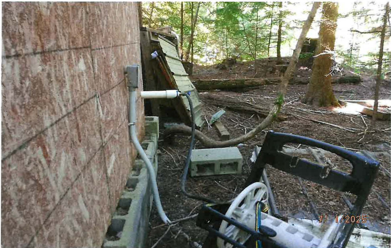
FIRE PROTECTION POU – BYPASS VALVE OFF 3-INCH PENSTOCK PIPELINE TO MULTIPLE 100-FT HOSE ROUTED UP TO PRIMARY RESIDENCE STAGED FOR FIRE SUPPRESSION
