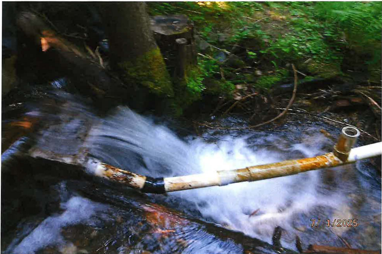
POD – REPURPOSED ELECTRIC CONTROL PANEL BOX WITH MESH SCREEN CAPTURING CREEK WATER INTO 3-INCH PVC PIPELINE
