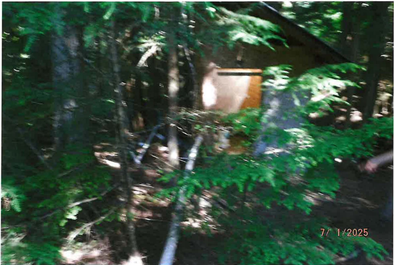
3-INCH PIPELINE RUNS ABOVE GROUND AND BURIED FOR A LARGE SECTION OF RUN, DAYLIGHTING AND ABOVE GROUND LAST 40-FT TO POWER STATION
