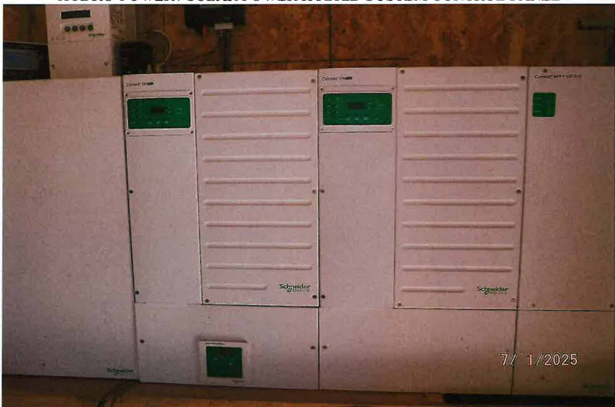
HYBRID HYDRO-SOLAR POWER BATTERY BANK (CO-LOCATED WITH RESIDENCE)
