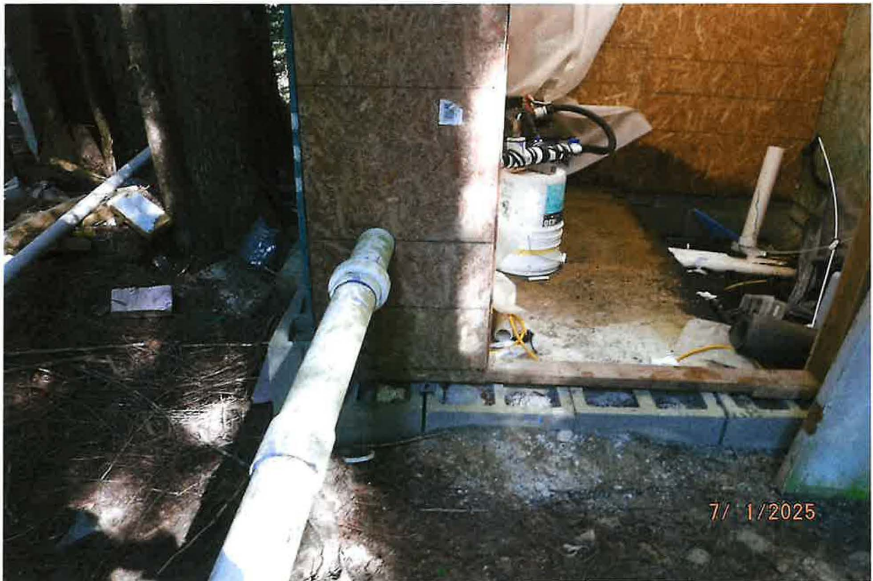
POWER POU – 3-INCH PIPELINE ENTERING POWER STATION
