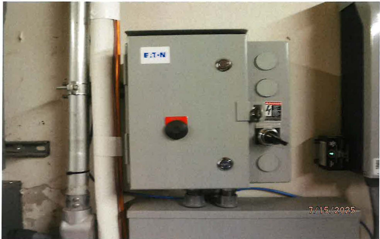
PUMP MOTOR RELAY CONTROL PANEL – 7.5 HP
