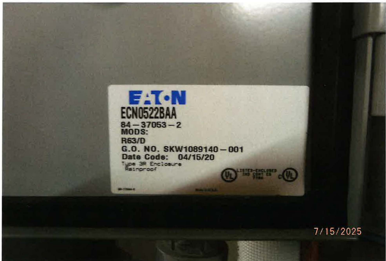
FRANKLIN ELECTRIC EATON MODEL ECN0522BAA 7.5 HP PUMP MOTOR RELAY CONTROL PANEL, ATTACHED TO A GOULDS MODEL 85 GS 7.5 HP WELL PUMP
