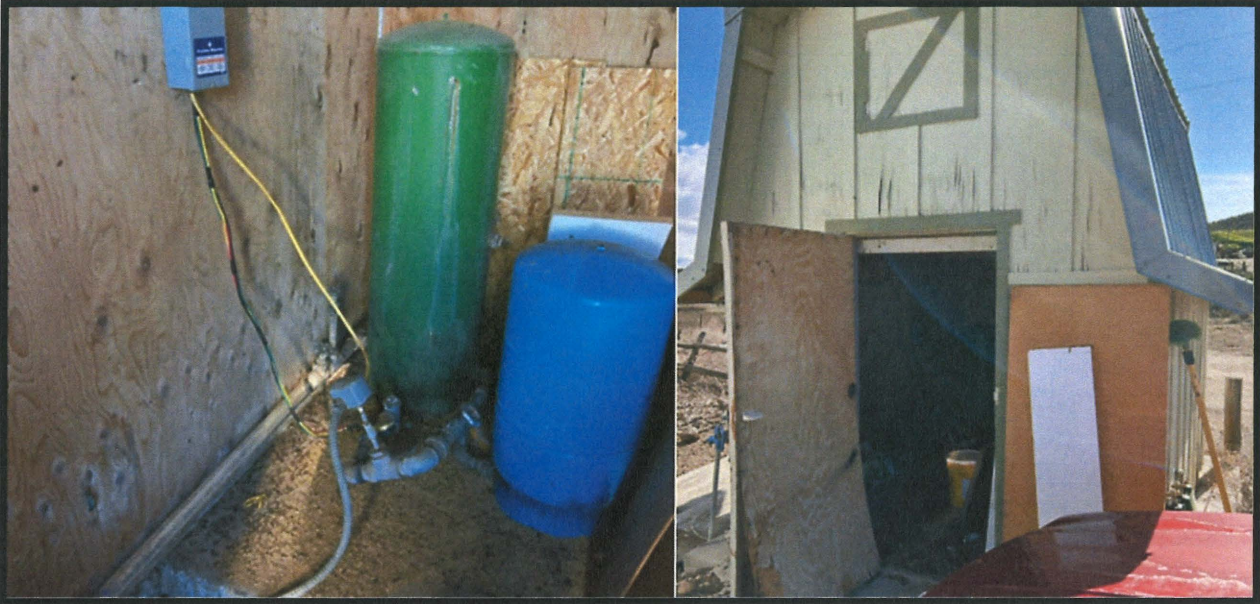
Photos 24 & 25- Domestic / stockwater pump house near the home north of the southwest stockyard area.
