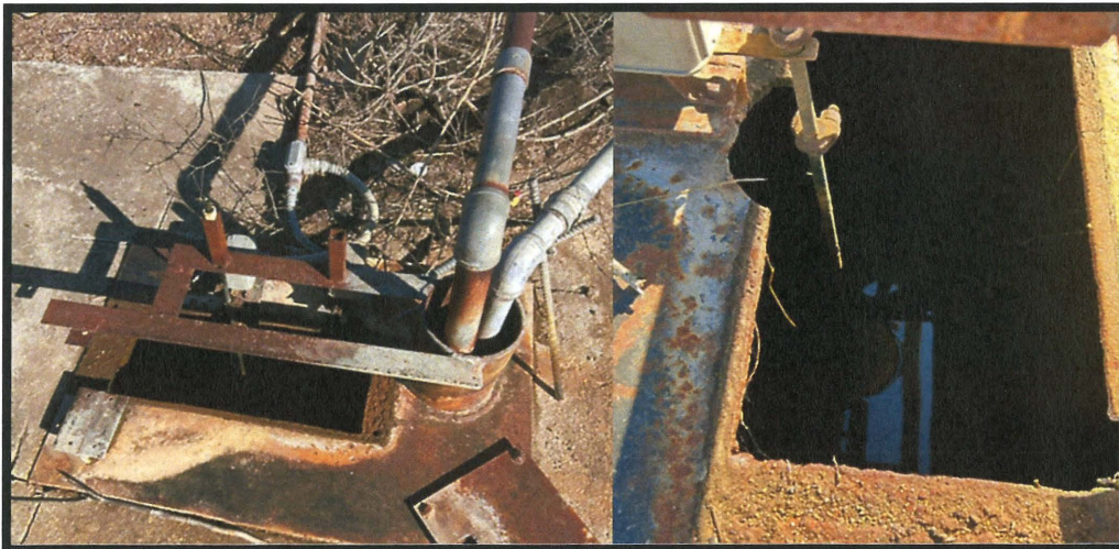
Photos 8 & 9- The control cable to the float valve sensor on the left and the other 2 pipes entering the hatch are the water lines from wells. The float valve is visible in the hatch (right image).
