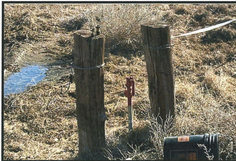
Photo 33- Frost-free hydrant found in “doctoring” areas north of the road crossing the southwest stockyard area.
