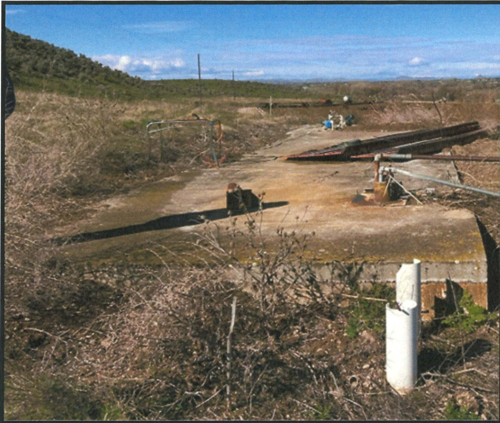
Photo 7- Standing on the east side of the 10' deep cistern, facing west. The hand valves for the gravity fed flow from the cistern in the white standing pipes. The 1 7/8" and 1 5/8" steel lines from the other 2 wells enter the cistern through the steel hatch in the top.
