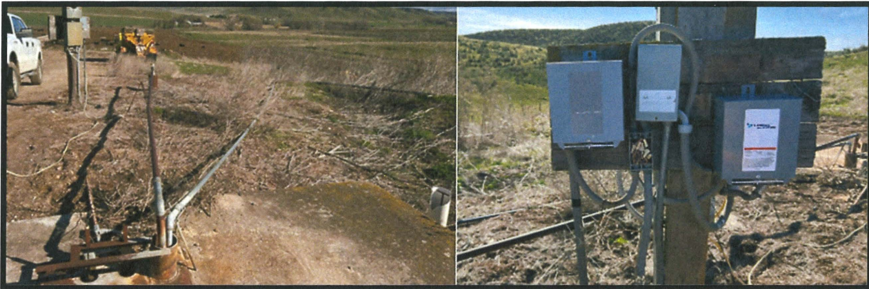
Photos 10 & 11- Standing on the cistern facing north (left) two well heads are in the background. Power for 3 wells (right).
