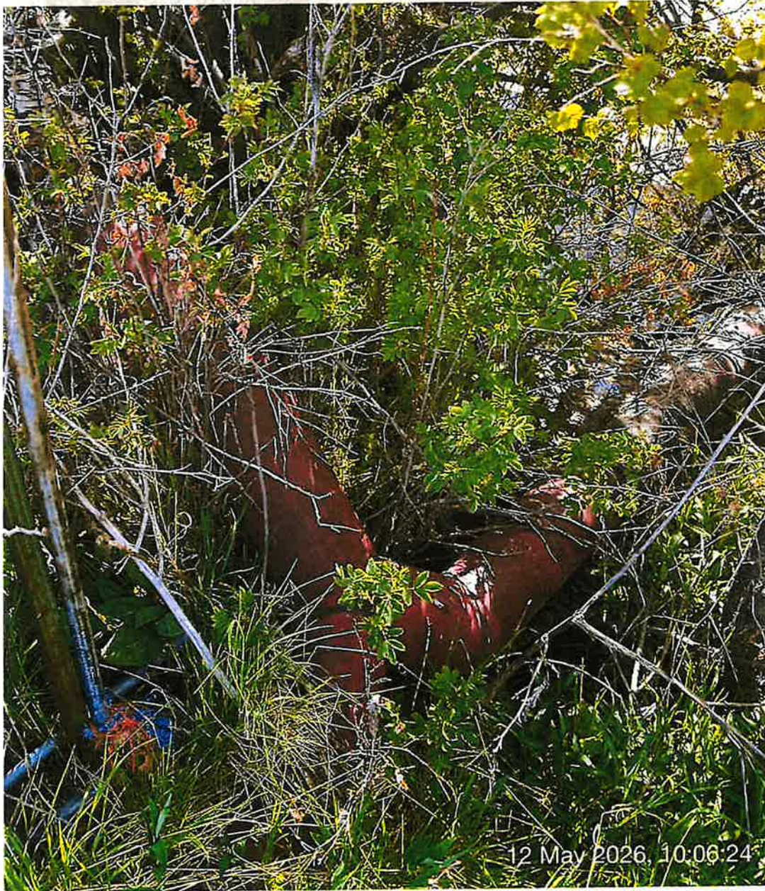
Pipe near the point of diversion splits flow. The 6" pipe pictured on the right directs flow across the creek. The pipe is buried and surfaces at the two openings at the top of the hill.
