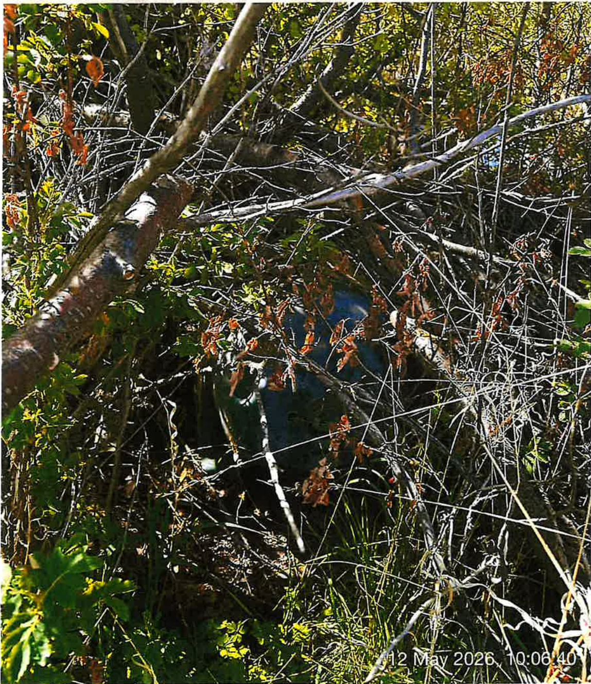
Irrigation pump. Very old condition, inactive, not currently functional. Buried in trees. Pump characteristics unknown.
