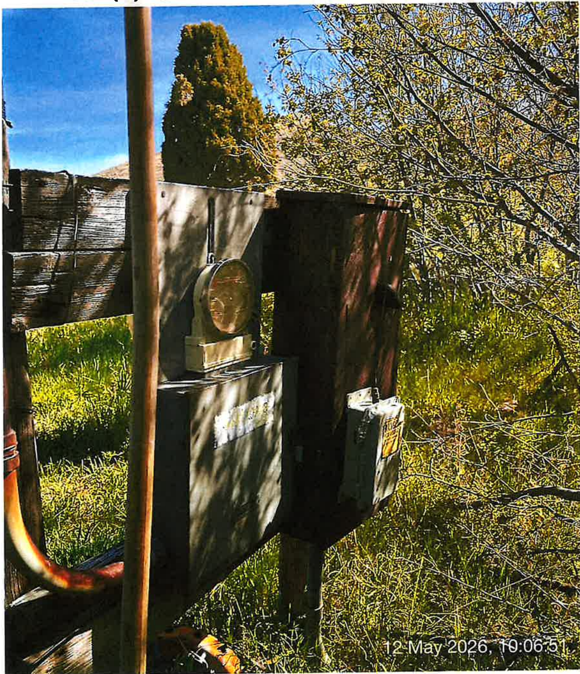
Power panel to pump. Not functional in 2026.
