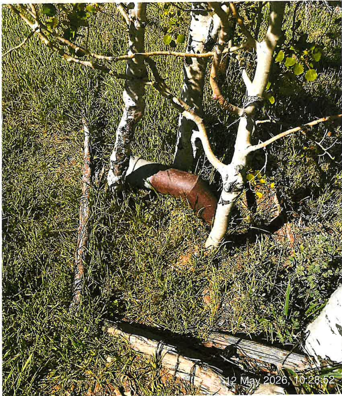
4" surfaced pipe opening that would direct water to handlines.
