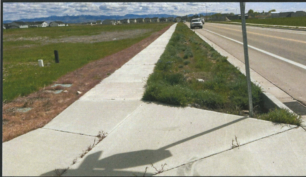
Photo 25- Taken at the northeast corner of N Owyhee Storm Ave & Achievement Dr. Facing east. The field is mostly overgrown with bunch grass and weeds. No sprinkler heads could be identified in the field or mow strip.
