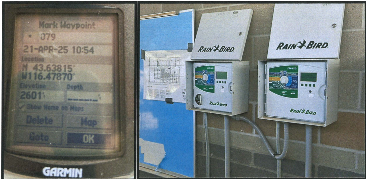
Photos 9 & 10- GPS Coordinates for the well head (left image). Two irrigation timers controlling distribution throughout the POU on the north wall of the pump house (right image).
