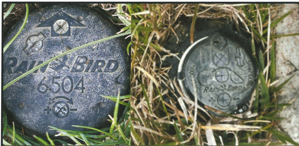
Photos 11 & 12- Rain Bird 6504 head (left image), as found throughout the rugby, soccer, baseball, and softball fields. Rain Bird 5000 (right image) as found throughout the smaller lawn areas and the landscaping surrounding the school.
