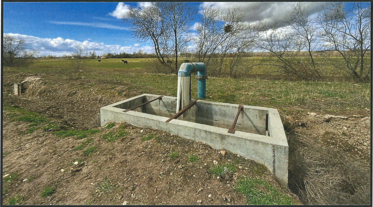
Photo 3- The diversion from the Snake River runs 93-100 via a buried line crossing under the drain ditch to the ditch pictured here, west of the permitted stockwater use.
