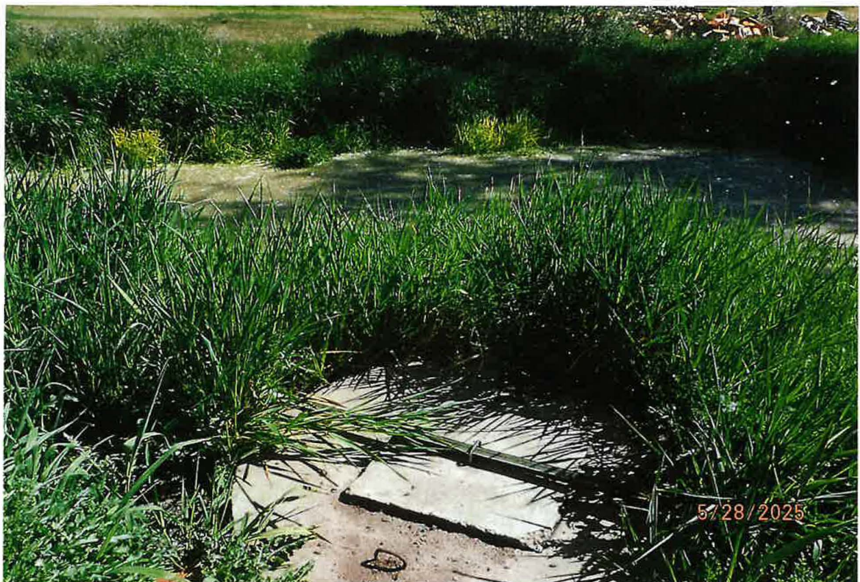
POD – WET WELL WITH INTAKE PIPE IN UNNAMED STREAM DIVERTED BY CENTRIFUGAL PUMP
