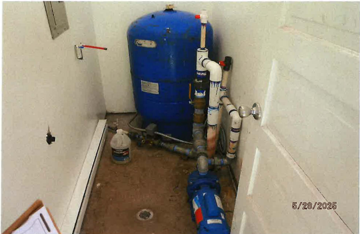
DIVERTING WORKS INCLUDE A GOULDS 2 HP CENTRIFUGAL PUMP AND 2-INCH DISCHARGE PIPE; SMALL PUMP STATION CO-LOCATED AT POD WITH WET WELL
