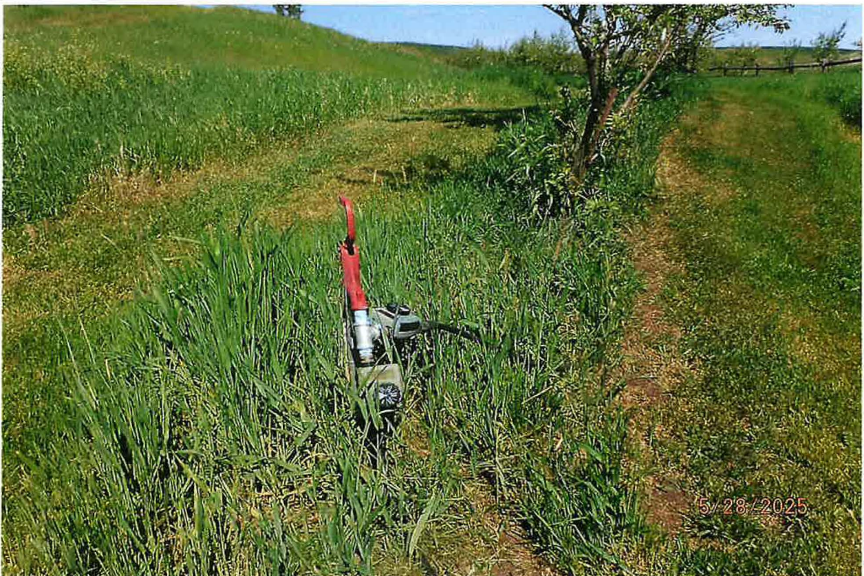
IRRIGATION POU – 2-INCH BURIED PIPELINE WITH HYDRANT RISERS TO SOAKER HOSE TIMER OPERATED ORCHARD TREE ZONES
