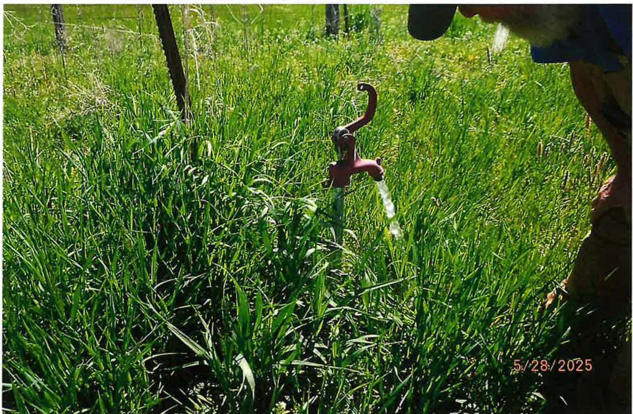
IRRIGATION POU – SOUTHWESTERN MOST IRRIGATION ZONE AND HYDRANT WITH FLOW SHOWN IN IMAGE
