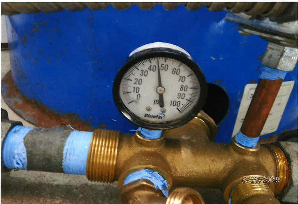
WATER SYSTEM PRESSURE 45 PSI WITH IRRIGATION ONGOING
