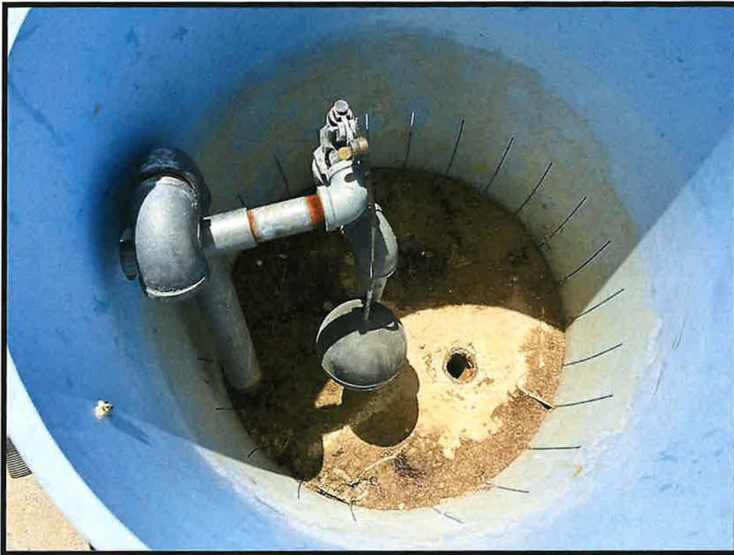
Photo 5- Float Valve system in the center of each trough. Taken at the trough in the NENE of Section 34 and NWNW of Section 35.
